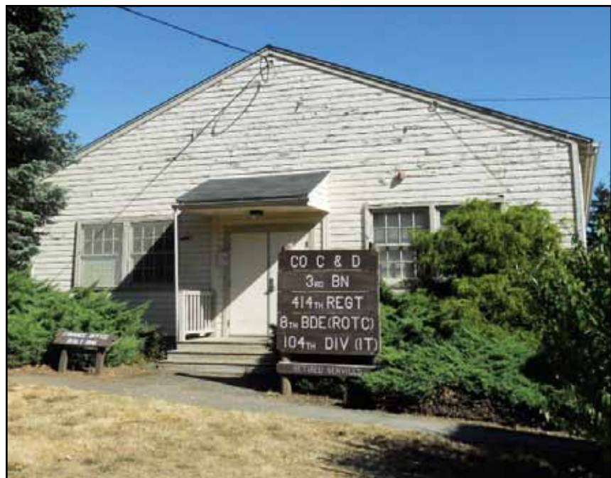
Figure 15. The west facade of building 728, showing distressed paint as one example of maintenance activities needed to stabilize and protect buildings in the East and South Barracks. (National Park Service)
