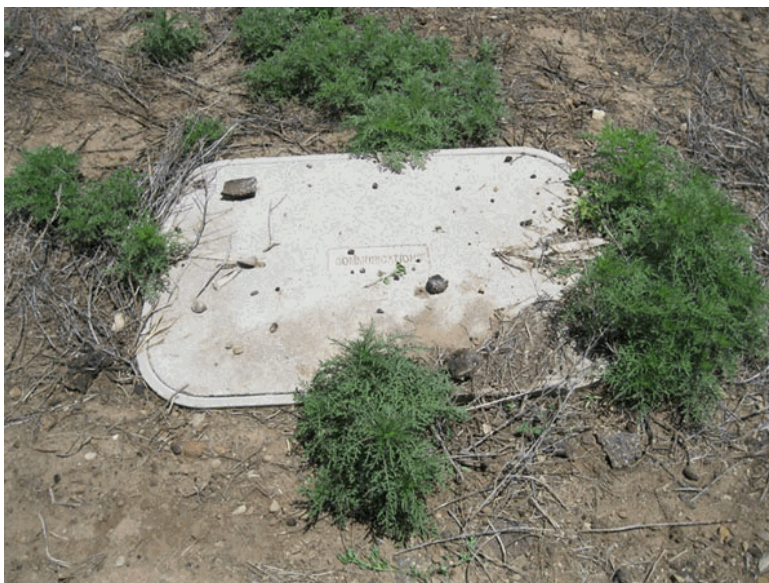
Utility cover that reads, "Communications," July 2010, Source: National Park Service.
