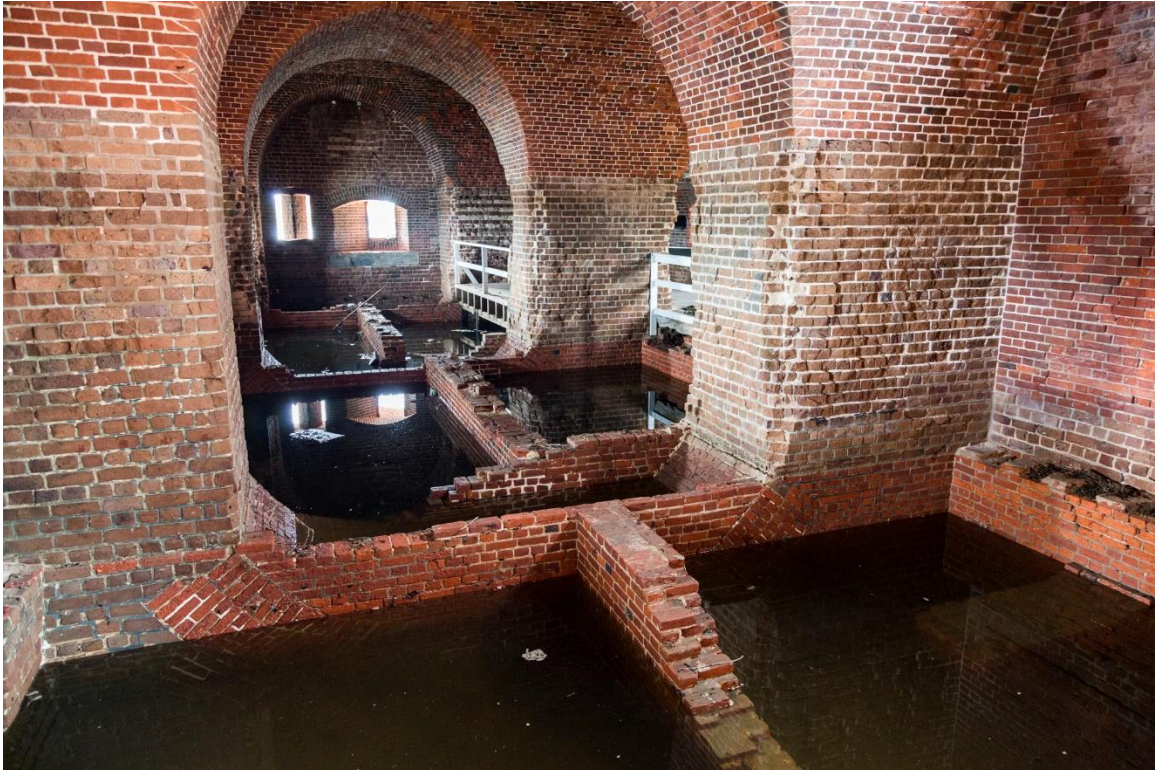
Figure 3. Flooding in the casemates of Fort Pulaski after Hurricane Irma (Eastern IMT, “091317_Fort Pulaski_Fort_031”).
