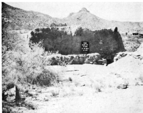
Ⓓ HS 026 • NORTH ELEVATION BEFORE 1967 STABILIZATION, SAME VIEW AS Ⓐ.
