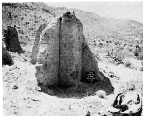
Ⓓ HS 035 • NORTH ELEVATION BEFORE 1967 STABILIZATION. SAME VIEW AS Ⓓ.
