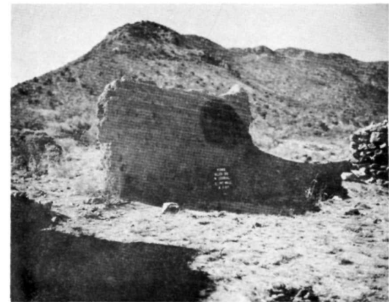
Ⓕ HS 035 • WEST ELEVATION BEFORE 1967 STABILIZATION. SAME VIEW AS Ⓒ.
