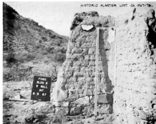
Ⓑ HS 004 & 005 • NORTH ELEVATION BEFORE 1967 STABILIZATION. SAME VIEW AS Ⓐ.
