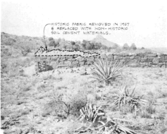
Ⓓ HS 034 * NORTH ELEVATION BEFORE 1967 STABILIZATION. SAME VIEW AS Ⓒ
