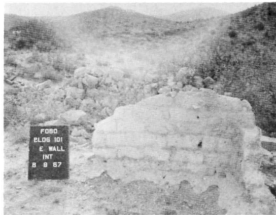
Ⓑ HS 101 • WEST ELEVATION BEFORE 1967 STABILIZATION. SAME VIEW AS Ⓐ
