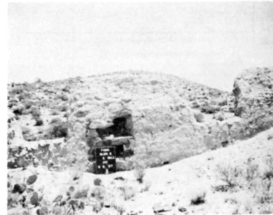
(C) HS 000 • WEST ELEVATION BEFORE 1967 STABILIZATION, SAME VIEW AS (D) 36
