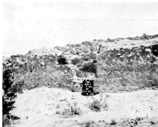
(E) HS 000 • WEST ELEVATION BEFORE 1967 STABILIZATION, SAME VIEW AS (A) 37 & (B) 37
