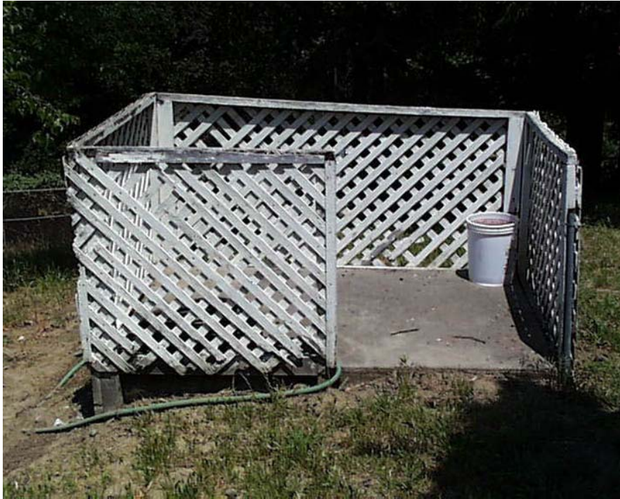
Photograph of the garbage enclosure. This is a contributing structure and is in poor condition (PWR, Seattle 2003).
