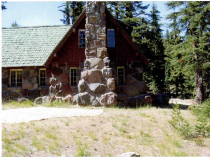
Photo 55 Fill is necessary particularly along the base of the chimney to prevent the large boulders from appearing to 'float' above surrounding grade.
