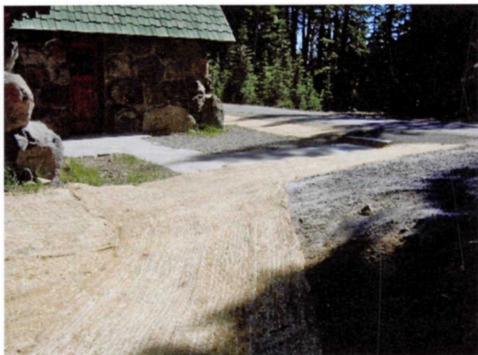
Photo 51 It is unsurprising that the access path, inconvenient, illogical and with a dangerous step is unused and users of the house walk straight cross the gravel and erosion matting to the door.
