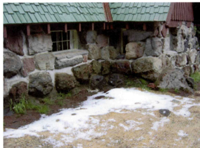
Photo 59 Erosion where roof runoff is concentrated requires extensive fill and small stones at drip line to break force of water.
