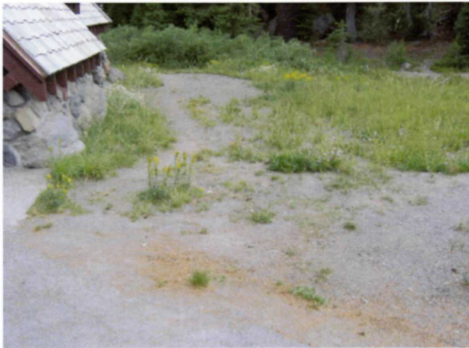
Photos 36-37 Extensive regrading and clearing of construction debris is required throughout the area particularly at the north end in the vicinity of the snow tunnel.
