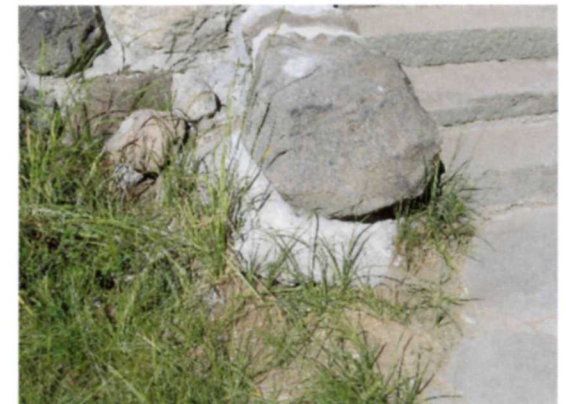
Photo 58 Detail of concrete shim holding up boulder at steps. Fill material should completely cover concrete so that boulder appears to merge into ground.
