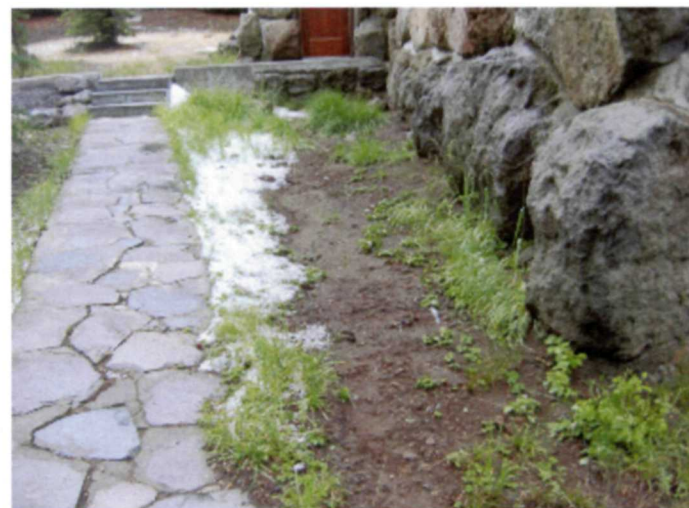
Photo 60 Erosion along west side of house requires fill to divert water away from building.
