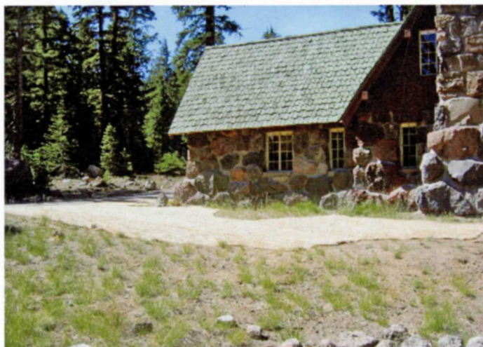
Photo 52 A 'sea' of erosion matting surrounds the building much of it on flat areas where erosion is unlikely. It appears to suppress rather than encourage natural tree, forb and grass regeneration.
