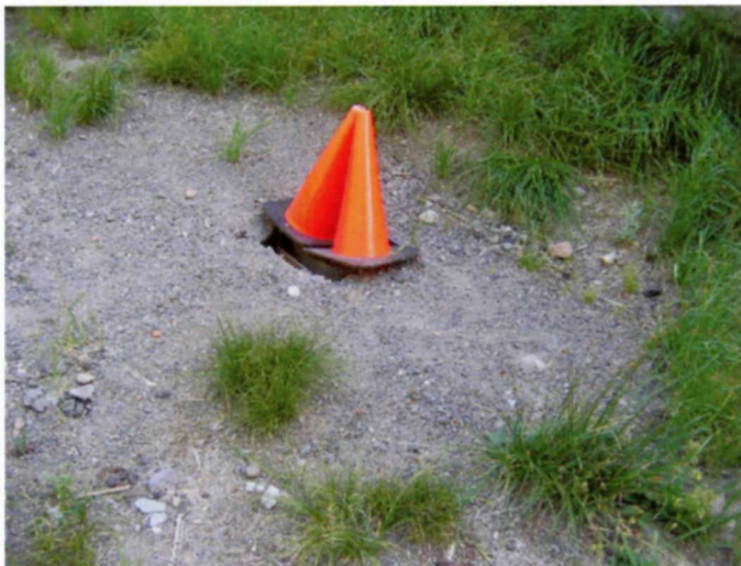
Photo 37 Holes remaining from earlier utility work should be capped or filled. Orange cones are not a long-term nor aesthetically pleasing solution.
