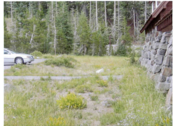
Photo 41 Thin vegetation behind the Administration Building probably resulting from vehicle damage. Planted clumps of firs should not obscure views from windows or be located close to the wall.
