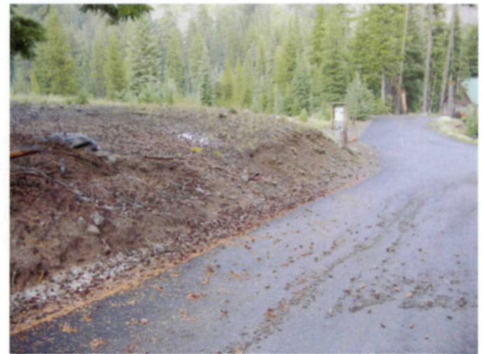
Photo 68 Steep and eroding cut bank needs to be cut back to merge with meadow surface.
