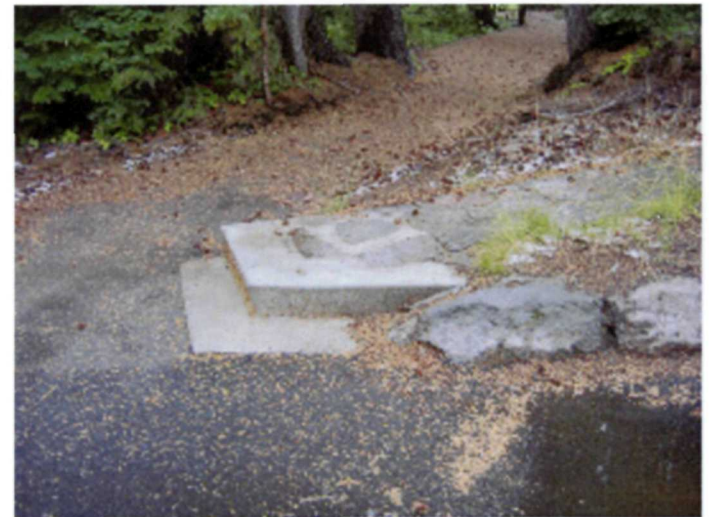
Photo 64 Dangerous tripping hazard step at end of path should be removed.
