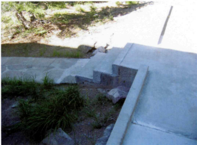
Photo 62 Fill to reduce the obtrusiveness of the awkward steps
