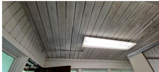
West Comfort Station, women’s room, paint needs cleaning or repainting.
