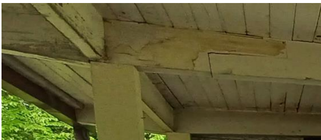
Pavilion, smaller area, failing scarf joint. Beam failure due to water ingress.
