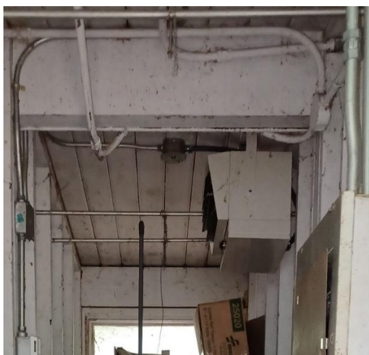
Mechanical closet, East Comfort Station, Heater.
