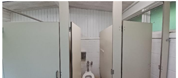
West Comfort Station, women's room, south partition wall.
