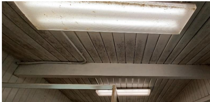
Light fixture in East Comfort Station, women's Room.
