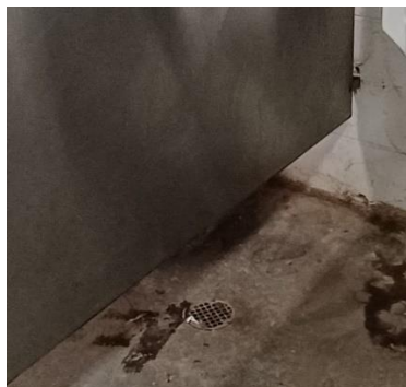
West Comfort Station, men's room drain.
