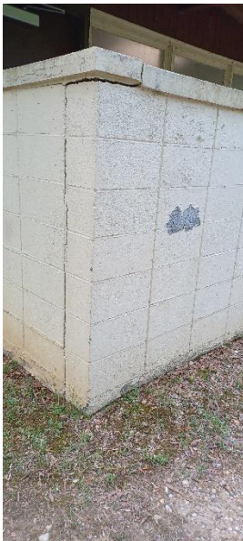
East Comfort Station – Southwest oblique. Damaged Privacy wall.
