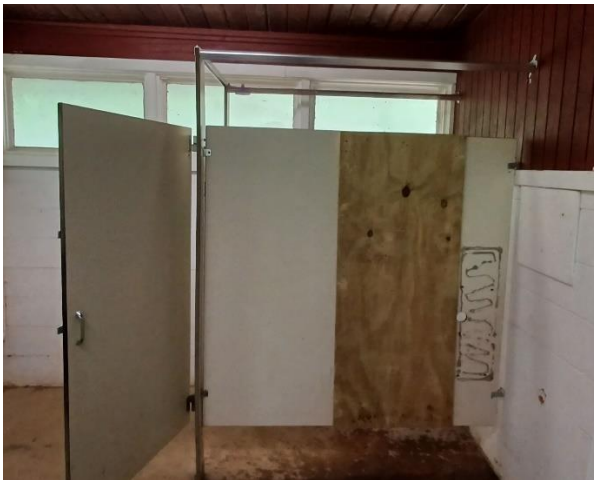
East Comfort Station, men's room stall walls.
