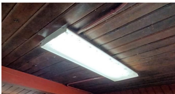
Light fixture in West Comfort Station, men's room.
