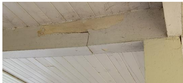
Pavilion, large picnic area, failing scarf joint.
