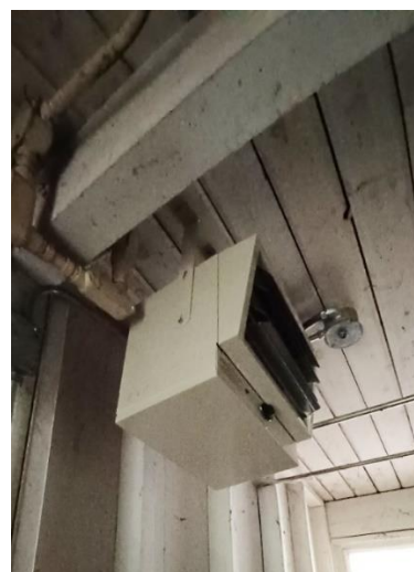
Mechanical closet, West Comfort Station, heater.
