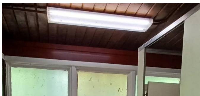
Light fixture in East Comfort Station, women's Room.
