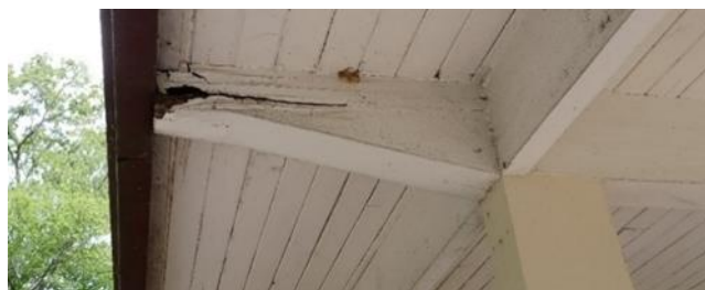
Deteriorated large rafter tail and tongue-and-groove wood ceiling paneling in need of repair and paint.
