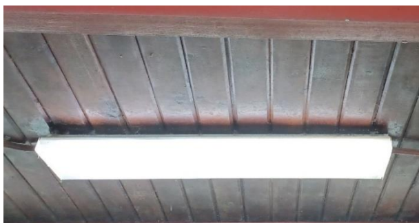
Light fixture in East Comfort Station, men's Room.
