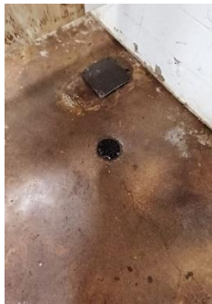
East Comfort Station men's room drain.
