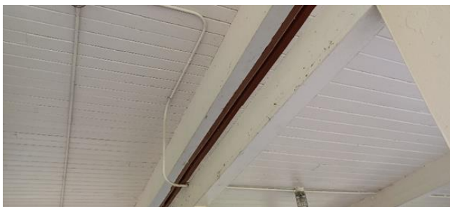
Central beams in larger picnic area. Note deteriorating paint on beams.
