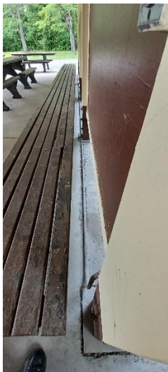
Bench and wood panels. Note: cracking paint on wood panel.
