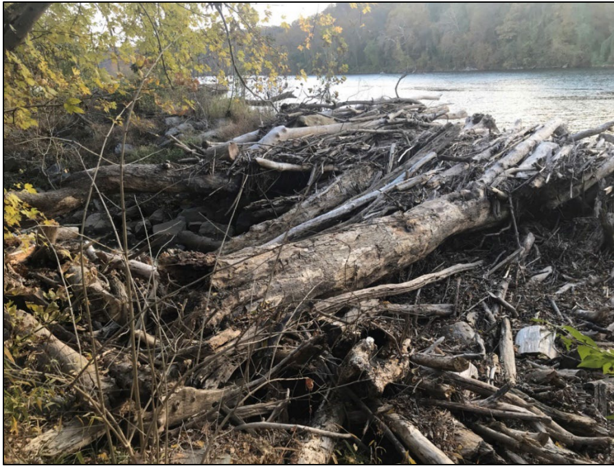
Figure 3-16. Flood debris such as fallen logs block the entrance to the sluiceway (Quinn Evans, 2021).
