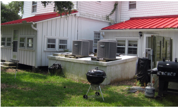
FIGURE 3-69. HVAC units, 2014. (NPS/SER-CRPS Collection)
