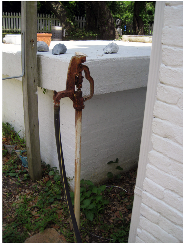
FIGURE 5-21. Metal yard hydrant with hose post in the background. (NPS/SER-CRPS Collection)
