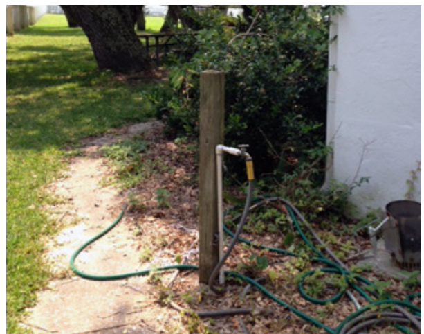
FIGURE 3-61. Spigot near south apartment, 2014. (NPS/SER-CRPS Collection)
