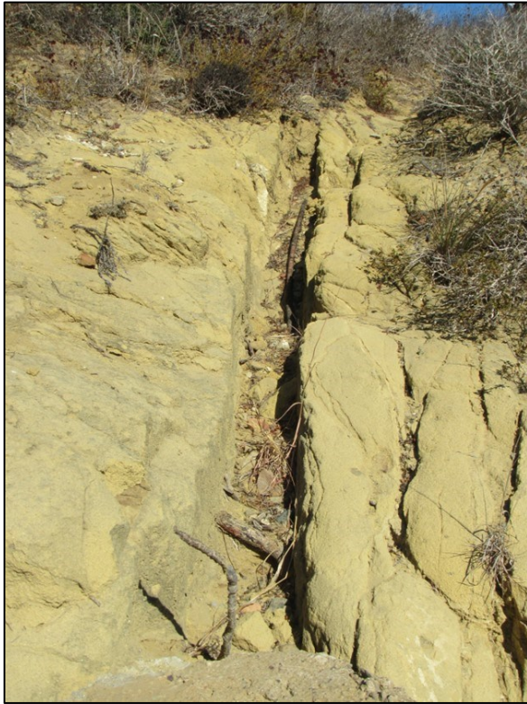
Archaeological Sites #12. Unfilled vertical cut along Bayside Trail with exposed pipe (PWRO, November 2017).
