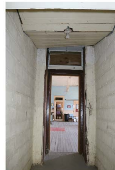
6 The wood ceiling in the hallway connection is deteriorated, shows signs of previous roof leaks, and appears to be dropping.
