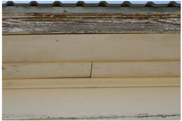
4 Deteriorated wood at fascia, soffit, trim board and molding.
