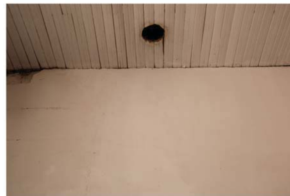
5 Hole in the beaded board tongue-and-groove ceiling boards from a previously installed chimney flue.
