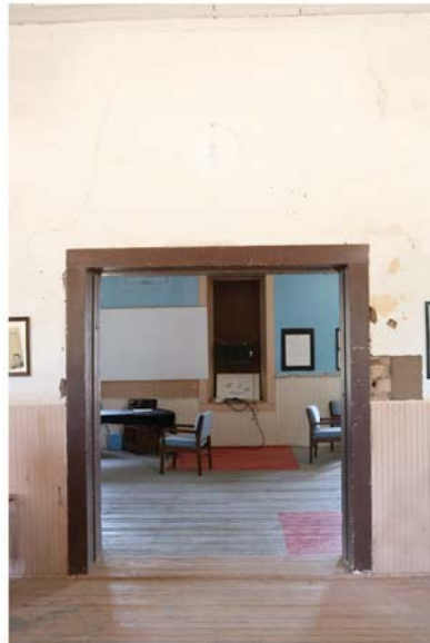
1 There is a raised wood threshold at the opening between rooms.
