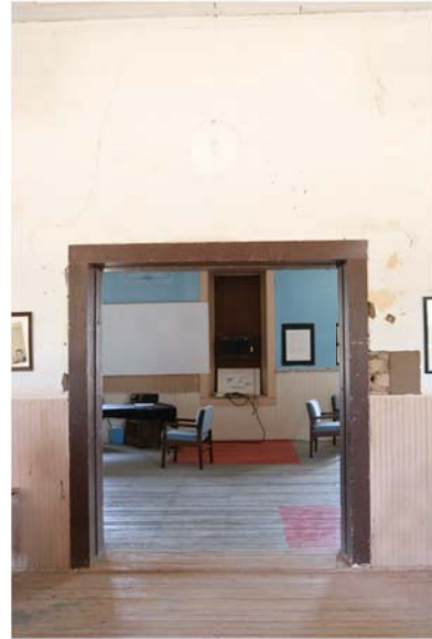
2 Opening between classrooms shows evidence that hinges and doors were previously installed. Opening may not be original.
