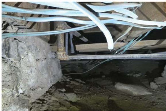
4 The rubble foundation has been knocked out to provide access , plumbing and electrical lines. The wood ledger supporting the floor joist has been modified and is in a cantilever position which has caused some damage to the floor joist.
