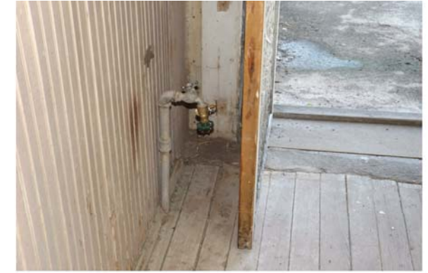
4 Hose bib inside building is assumed to be part of trade school period. Wood has rotted due to the unusual location of the faucet.
