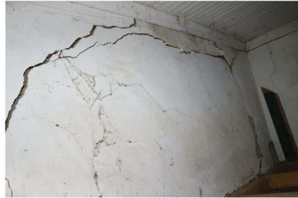
3 Numerous surface cracks at inside corner reveal delamination from wall and surface plaster is out of plane. Cracks are not visible below office ceiling due to installation of paneling on lower portion of wall.
