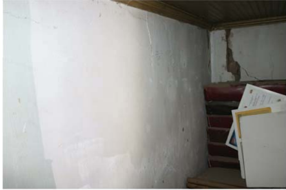
1 Vertical cracking at inside corner appears in structure along with numerous plaster repairs.
