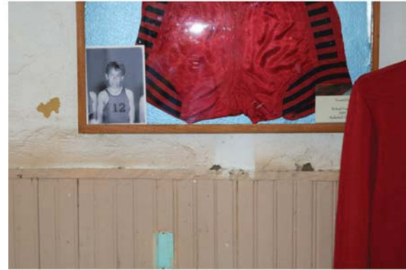
5 Repairs are evident above the wainscot where the cap has been chiseled off. The missing electrical outlet reveals a previous layer of aqua paint.
