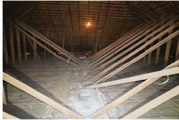
2 The regular diagonal supports on the south side of the building are missing, lack of support has caused the roof deck to sag on portions of the roof.
