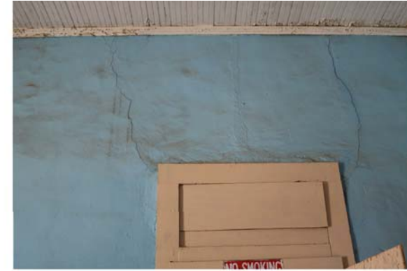
3 Cracks appear on both sides of door assembly transom is blocked at connection to band hall beyond.
