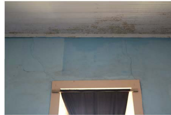
3 Cracking above window at the corners is common where the window creates a natural weakness in the structure.
