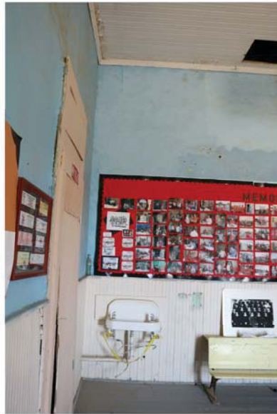
1 Water fountain appears to have been a source for visible moisture damage. Cap of wainscot has been chiseled off.
