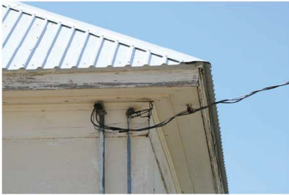
1 Corner shows hard cement stucco edge and deteriorated fascia and trim.
