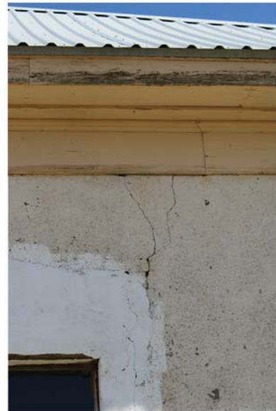
5 Cracks extending upward from window are not unusual and not of major concern.
