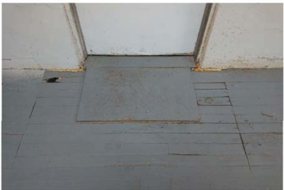
4 Plywood partially covers deteriorated floor boards which appear to have been previously replaced.
