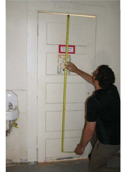
6 the five-panel wood door has been cut along the bottom rail.
