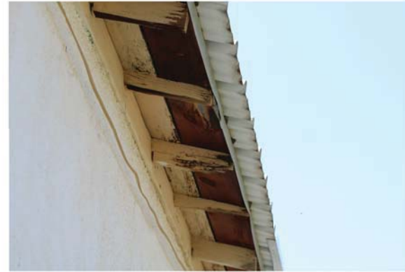
3 Rafter tails and roof deck are rotted.
