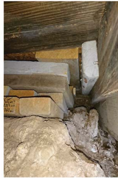
3 Random assortment of wood blocks support rotten floor above, floor joists in this area also deteriorated.
