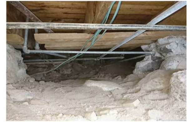
4 Rubble foundation wall has been knocked away for plumbing access. Wood joists are not fully supported.
