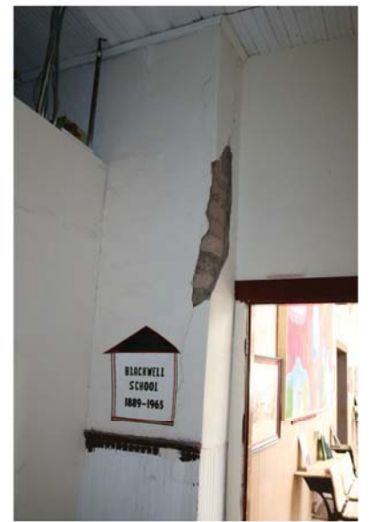
6-B Loose plaster was determined to be a safety concern and was taken down.
