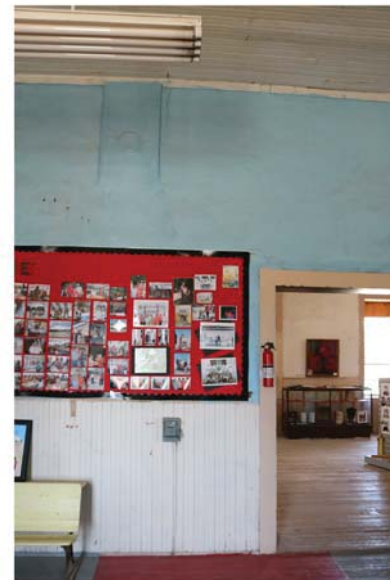
3 Breaker box may date to period of trade school. Cap of wainscot has been chiseled off. Repair at upper left corner of doorway should be investigated.
