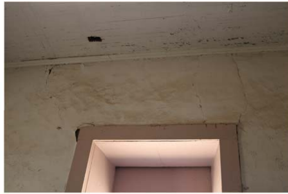
1 Wall above window shows signs of moisture and numerous plaster repairs. An opening has been cut in the ceiling and there is a ghost of a previously installed cross wall on the ceiling.
