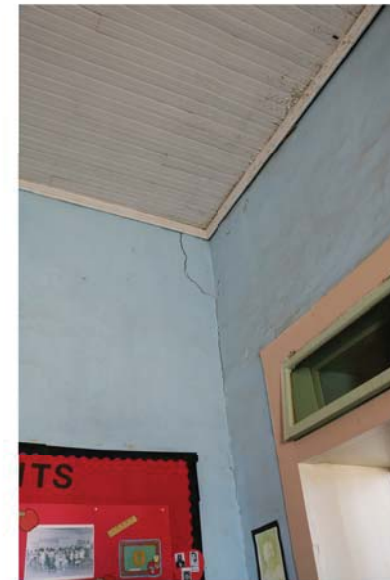
4 Crack at intersection of walls and plaster which is out of plane indicate movement in the structure.
