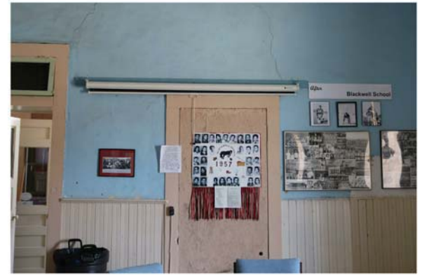
8 The wainscot cap remains intact to the left side of blocked doorway but has been crudely removed to the right side of the door.
