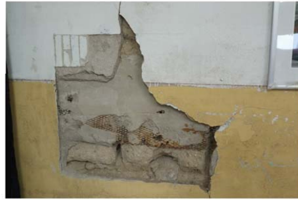
3 Previous attempt to tie stud wall to adobe wall where original north/south wall was removed. The wainscot along this wall has been removed and is indicated by a difference in paint color.
