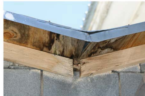
2 Valley of hallway link is badly deteriorated and poorly constructed.
