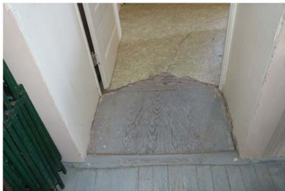
1 Plywood transition at threshold between blue room and office.
