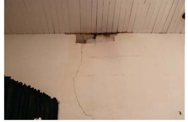
4 Metal lath and cement plaster have failed to tie the stud wall to the adobe where original wall was removed. Wood trim at ceiling no longer exists along this wall.
