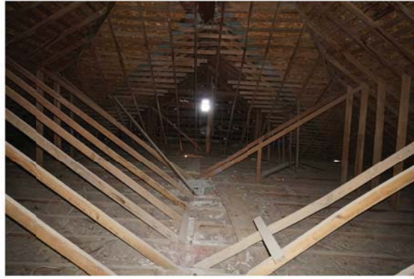
7 Framing members in attic are missing. This area corresponds with the bow seen in the roof from the exterior.
