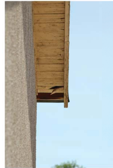
4 Soffit at rake of band hall is rotted.
