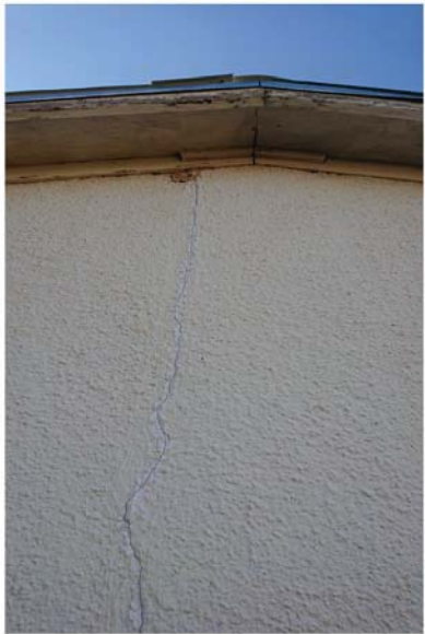
5 Crack in stucco runs full height of wall at location of abandoned chimney flue.
