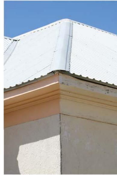
4 Gap below ridge cap and deteriorated fascia allow for pest intrusion.
