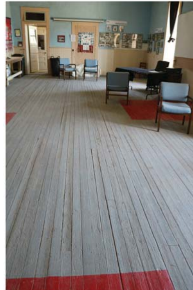
2 Floor planks show signs of wear and some cupping but are in useable condition.
