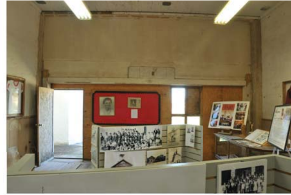
2 Infill wall at loading dock where original adobe wall was removed and is in poor condition.
