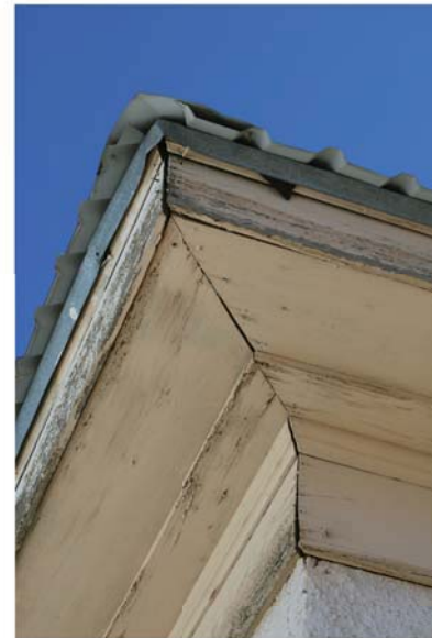
3 Weathered fascia and soffit hole at roof line allows pest intrusion.
