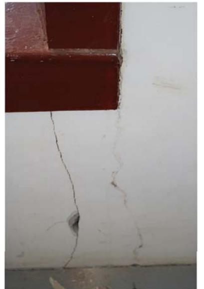
5 Vertical crack below window shows break in cement plaster which is expected at an opening.
