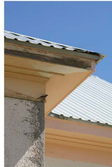
6 Deteriorated wood fascia and trim.
