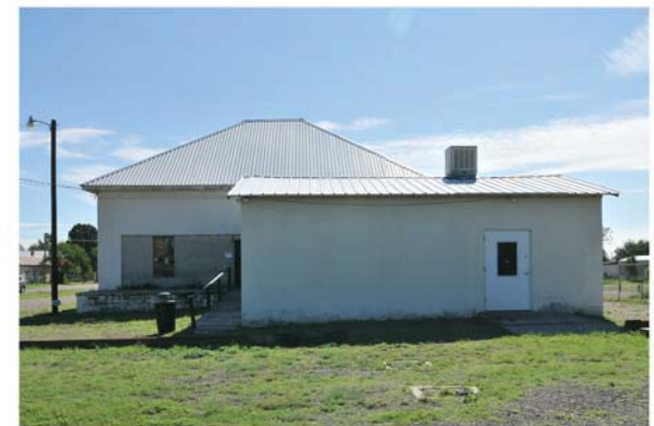
5 The "ghost" of five previously blocked windows is visible.
