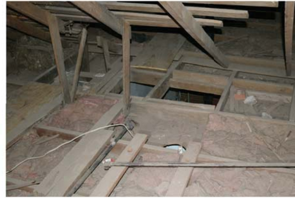
3 Remains of previously removed brick chimney are visible next to one of the roof attic access points.
