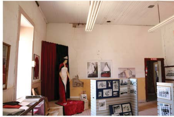
1 Overall view looking east in museum room shows the vertical crack where two structural systems intersect.
