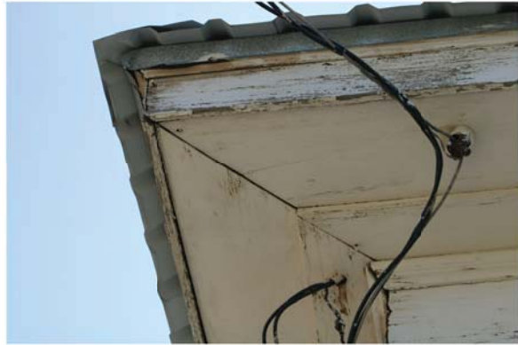
1 Deteriorated fascia and soffit, gap at drip edge.
