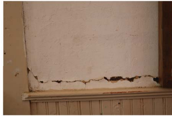
2 Various layers of plaster have fallen off revealing the adobe beneath.
