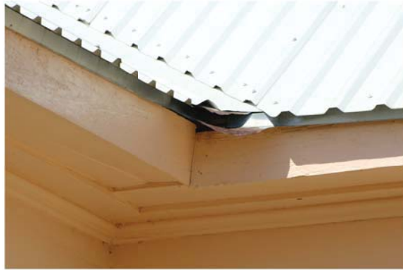
3 Gap in fascia below valley flashing allows for bird and pest intrusion.
