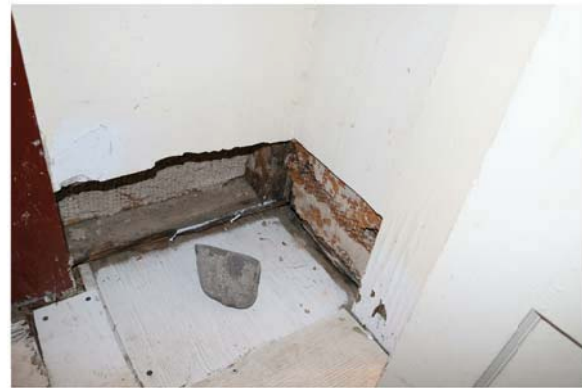
1 Water leak has caused floor to rot as well as sole plate and studs. Metal lath is rusted.
