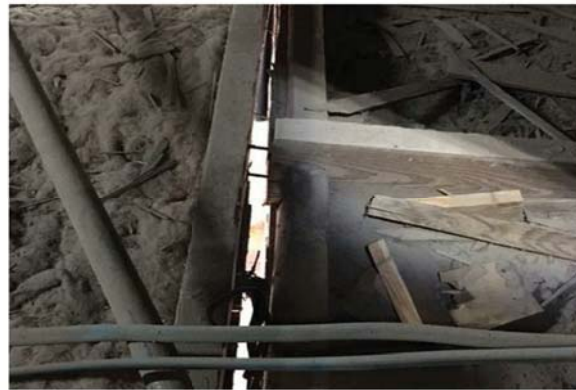
2 Structural members were pulled apart where structure changes direction.
