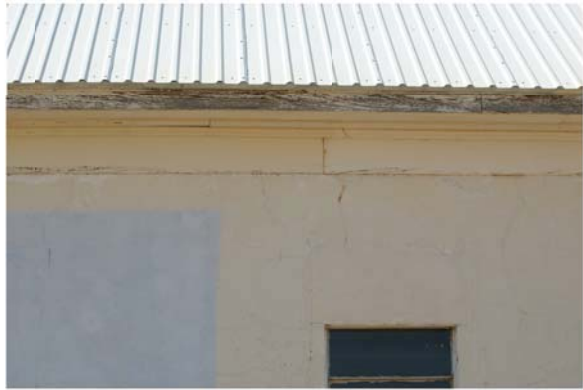
3 Deteriorated wood, plaster cracks on surface and at modified windows.
