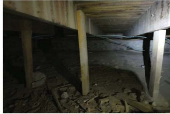
2 Secondary supports placed randomly under the floor joists.
