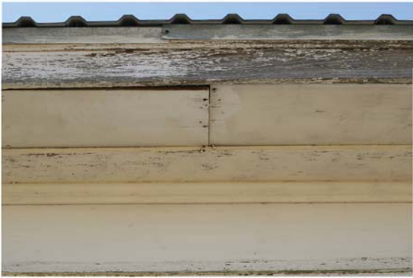
2 Fascia and soffit are deteriorated and detached from structure
