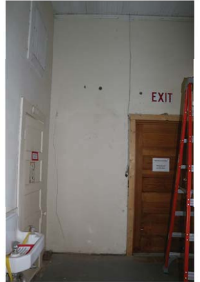
4 Vertical crack runs full height of wall and corresponds with location of previous reconstruction of adobe wall. Surface boring was conducted at two locations to locate and verify concrete lintel. Stucco on expanded metal lath and plaster was verified.
