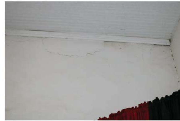
3 Cracks appear where repairs with different material content are placed adjacent to each other; There is no bond.
