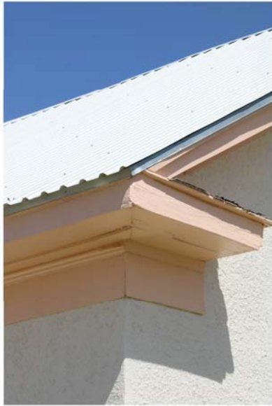
1 Closed soffit in relatively good condition though some pieces of trim are missing.
