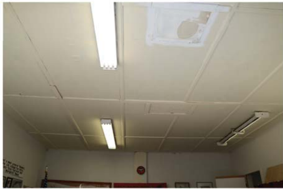
1 Attic of the band hall is accessible through hatch. Ceiling is patched under abandoned swamp cooler.
