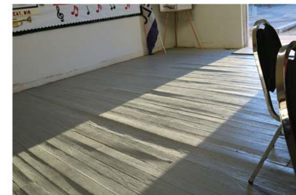
6 Floor planks in the band hall show some signs of wear and some cupping but are still in useable condition.
