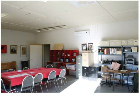
1 Doorway at ramp to main building. A new mini-split HVAC system has been installed on this wall.
