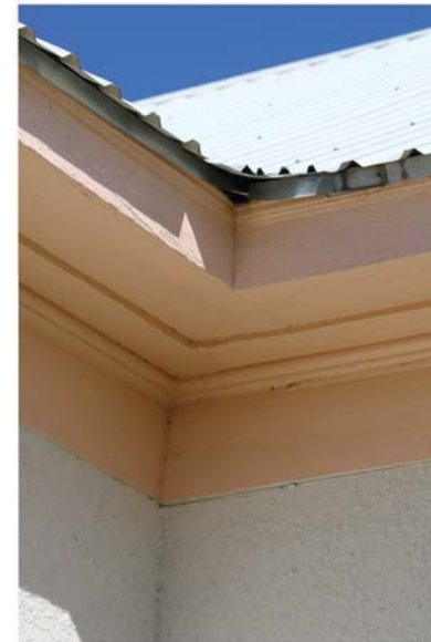
7 Gap below valley flashing allows for bird and pest intrusion.
