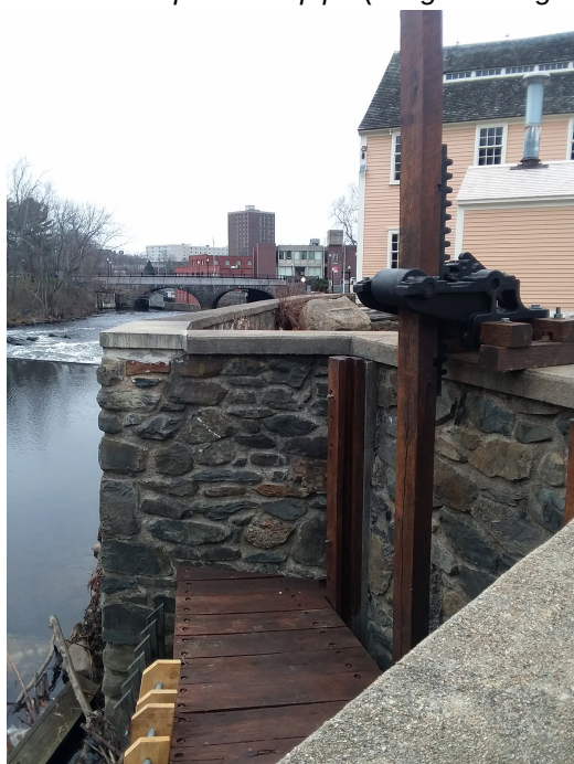
Figure 39. View of the trash rack and gate at the inlet of the penstock pipe. (OCLP 2021, IMG-20210111-140514)
