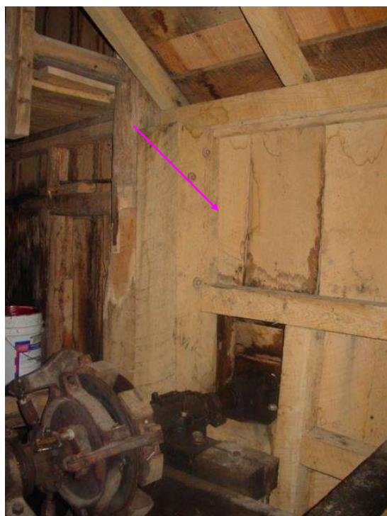
Showing water stains on the east wall of the interior in the mill section of the building, above case opening for the clutch of the mill.
