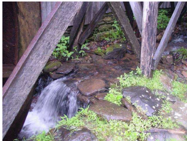
Siltation-clogged flumes overflow under the flume supports, sending sand/dirt/debris directly into the mill pond.
