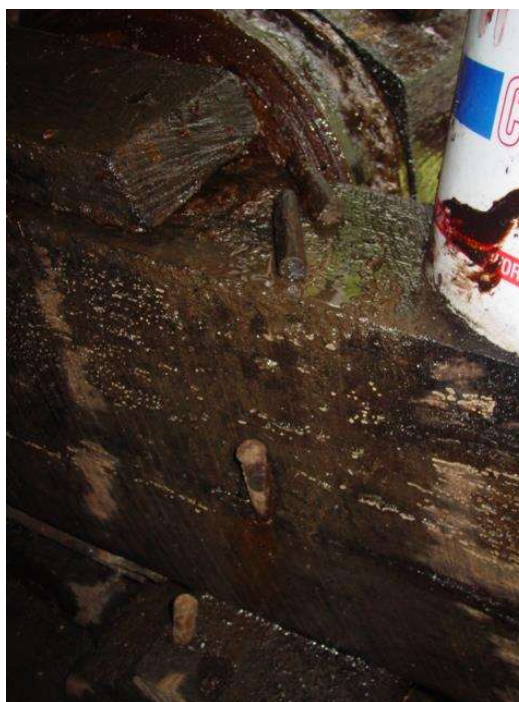
Viewing water damage on case opening of water wheel axle.
