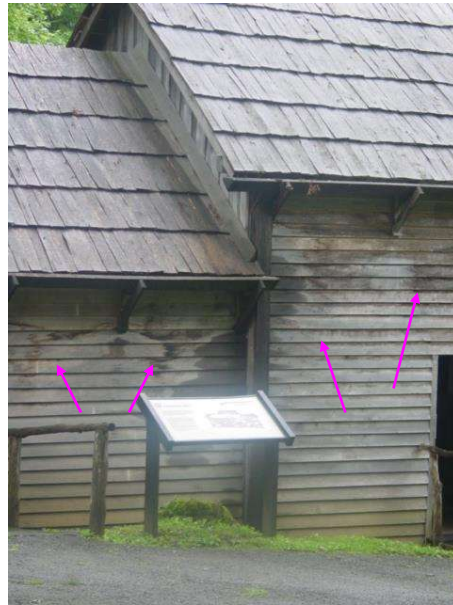
Connection of sawmill and gristmill on west elevation. Connection of gutters and down spout, that leads to leak problems if not cleaned. Roof shakes also visible.
