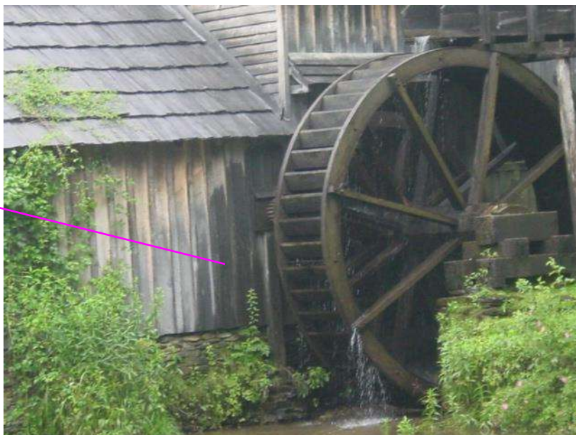
Viewing east elevation; note the wet façade and leaking water wheel and flume; seek professional evaluation of wheel; consider using an appropriate clear sealant for the east façade wood.
