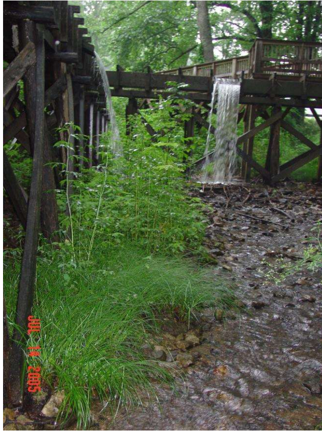
Water from overflow leaves a stream under flume.
