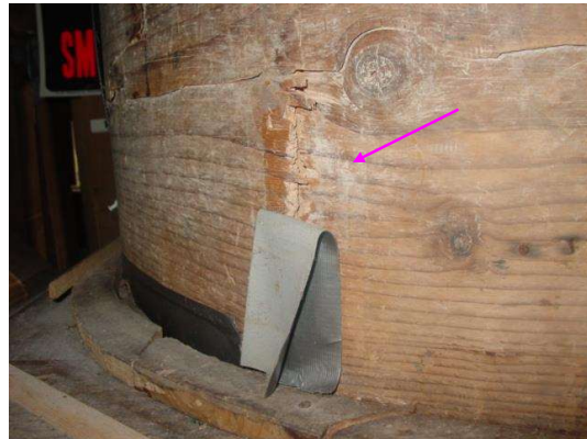
Cracks in buckwheat stone cover are under the duct tape.
