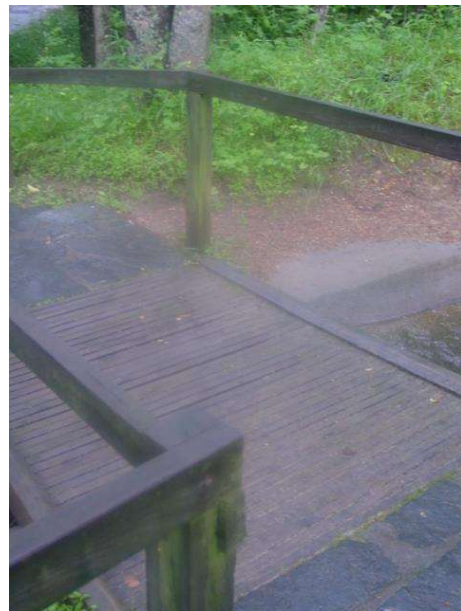
Slippery walk way/bridge: Stays wet during rainy/snowy season.
