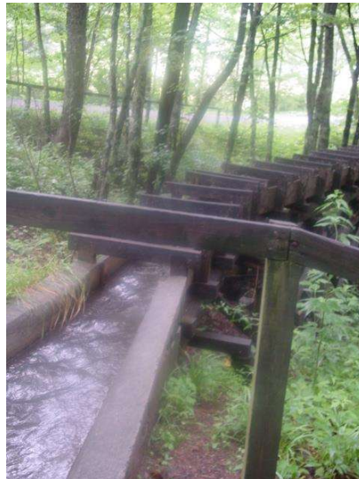
Concrete swell and flume connection; view is from standing on the wooden handicap walkway, looking east.
