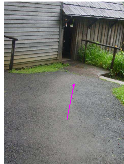
Viewing erosion, photo taken while standing near millstones in from of the west elevation of the mill looking towards the woodworking shop entrance near the north of the mill.
