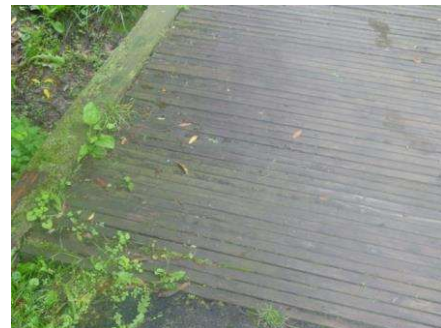
Slippery walkways are located near blacksmith shop and flume.
