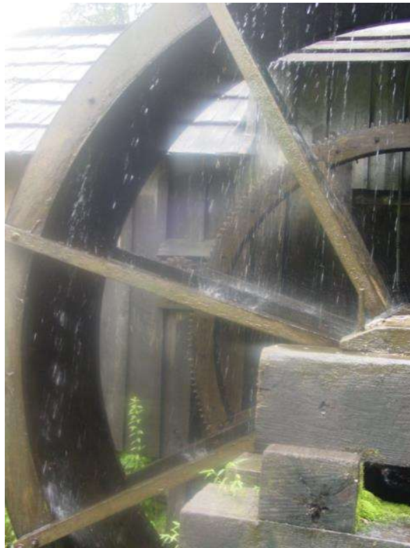
Wet water wheel: water wheel leaks, buckets inside of wheel need to be sealed; seek professional evaluation of the wheel leaks; water splashes on east elevation.
