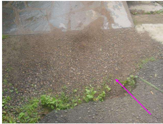
Erosion on the west elevation side near the carpenter shop entrance
