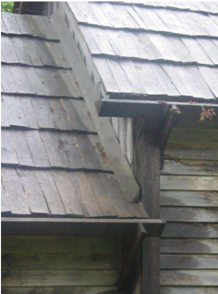
Connection of sawmill and gristmill on west elevation. Connection of gutters and down spout, that leads to leak problems if not cleaned.
