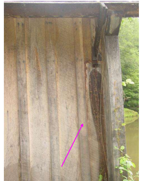
Corner on woodworking shop on west elevation [nearest to the north] vines are attached to the building and buildup will cause moisture.
