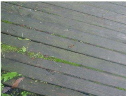
Algae that form on wet wooden walkways near the blacksmith shop.
