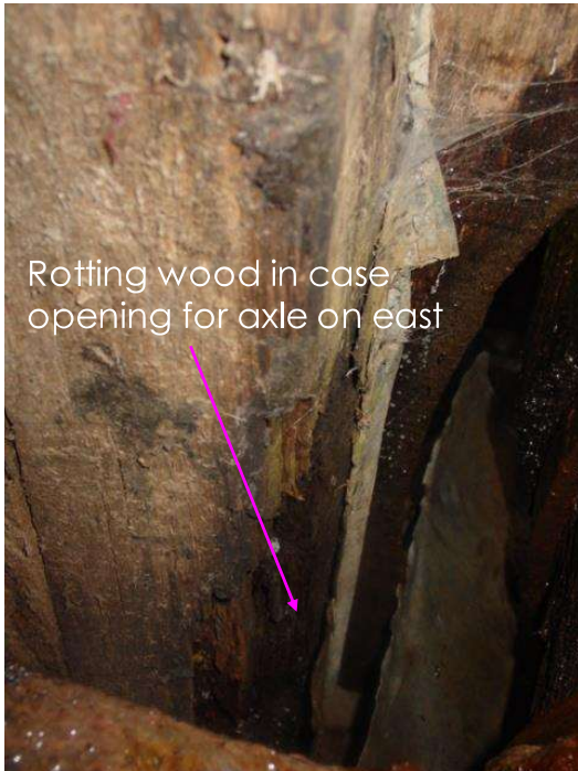
Water damage on case opening creates wood rot and needs to be replaced.
