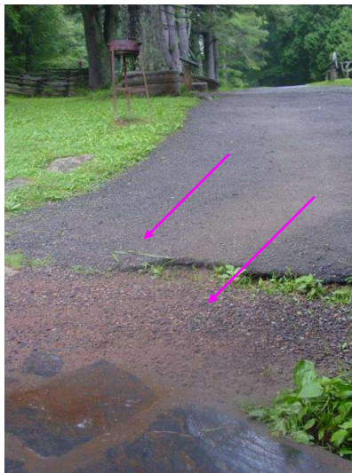
Viewing erosion on handicap walkway standing inside of woodworking shop looking to the west of the complex. Note: the uneven connection with the asphalt and ground. This should be fixed.
