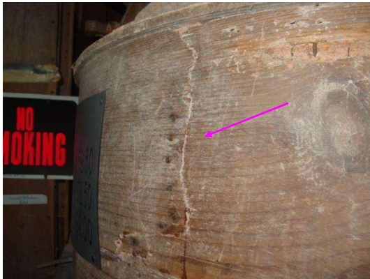
Cracks in buckwheat stone cover.
