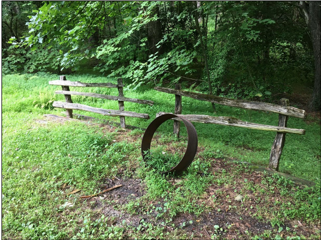
Fig 8-38. Deteriorating split rail fencing near trailer campsite along Loop C. Camera facing west (2021)
