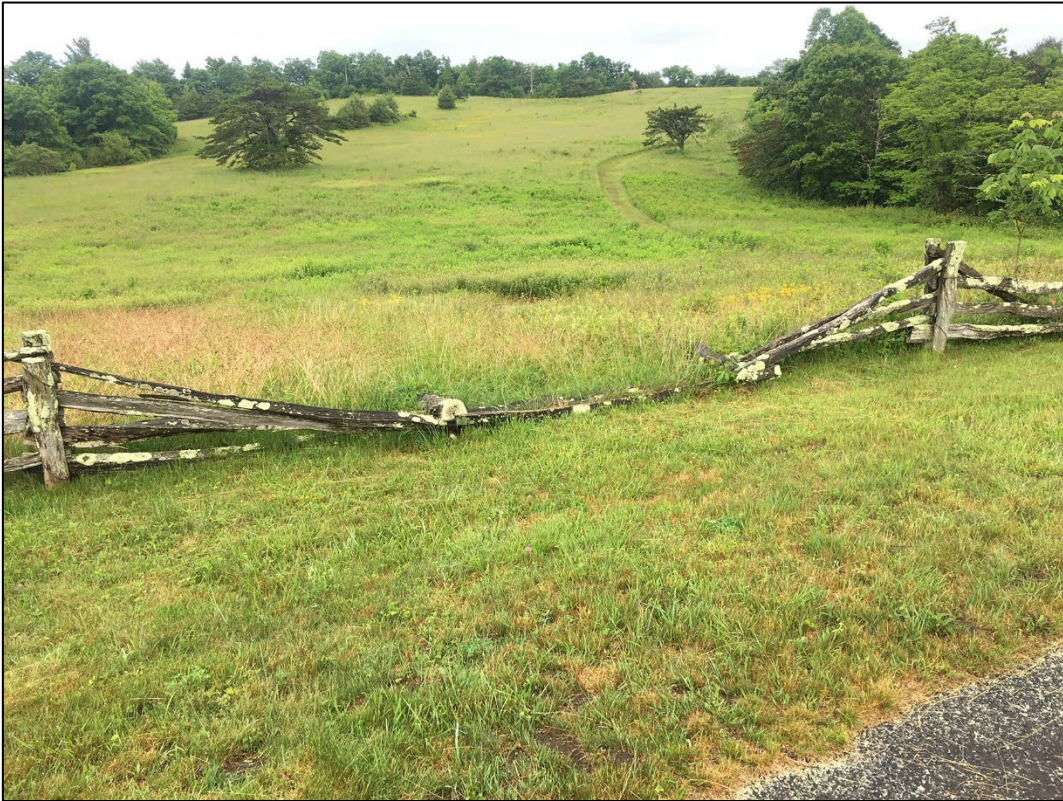
Fig 8-22. Section of collapsed split rail fencing near south meadow. Camera facing south (2021)
