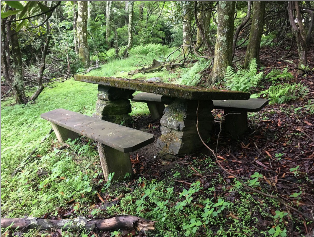
Fig 8-20. Stone picnic table in forested area downslope of Comfort Station #102. Partially collapsed. Camera facing northeast (2021)
