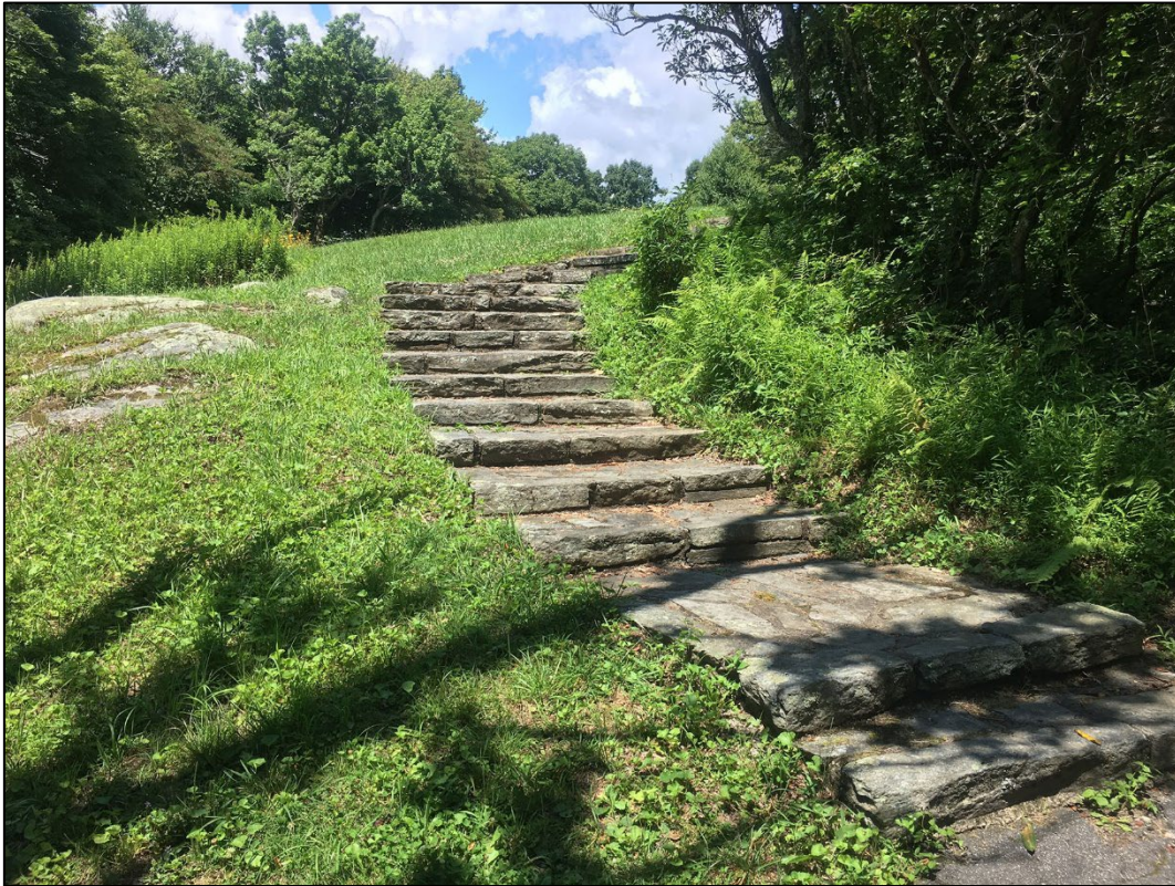
Fig 8-27. Set of 12 stone steps near Comfort Station #104 in fair condition, with deteriorated mortar joints. Camera facing northeast (2021)
