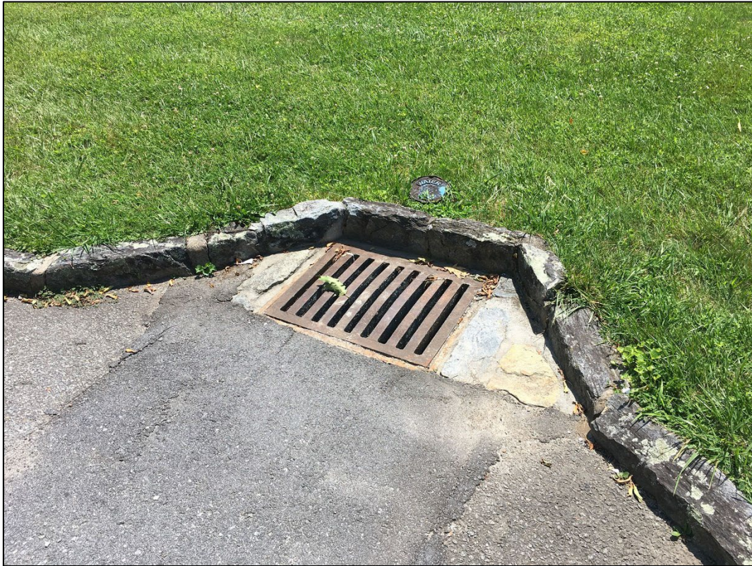
Fig 8-26. Drop inlet on south side of central access lane (2021)
