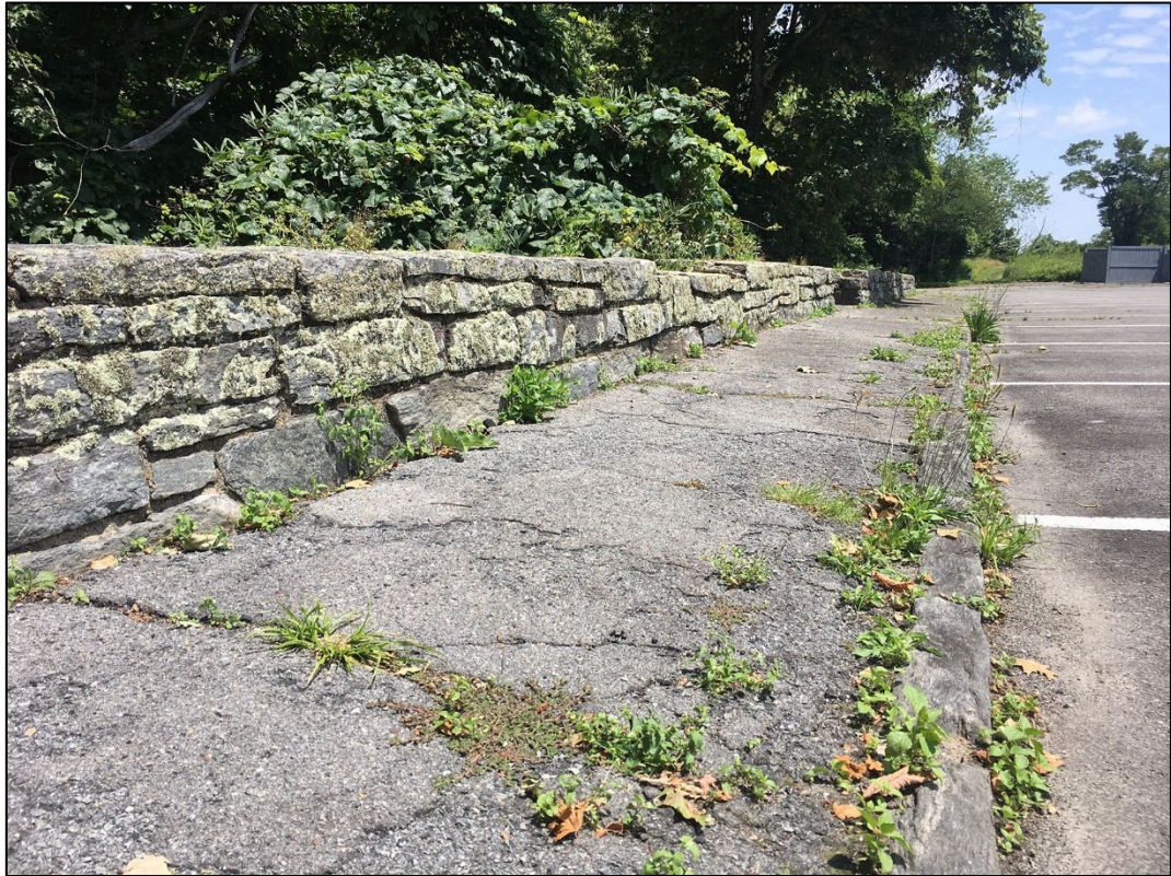
Fig 8-10. View of asphalt sidewalk along north end of east parking lot. Cracking and other wear evident (2021)
