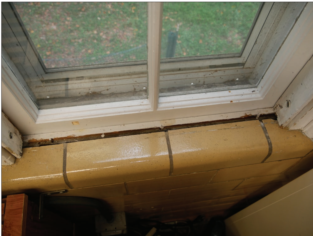
Figure 221. Losses in wood frame at tripartite window. Building Conservation Associates, 2025.
