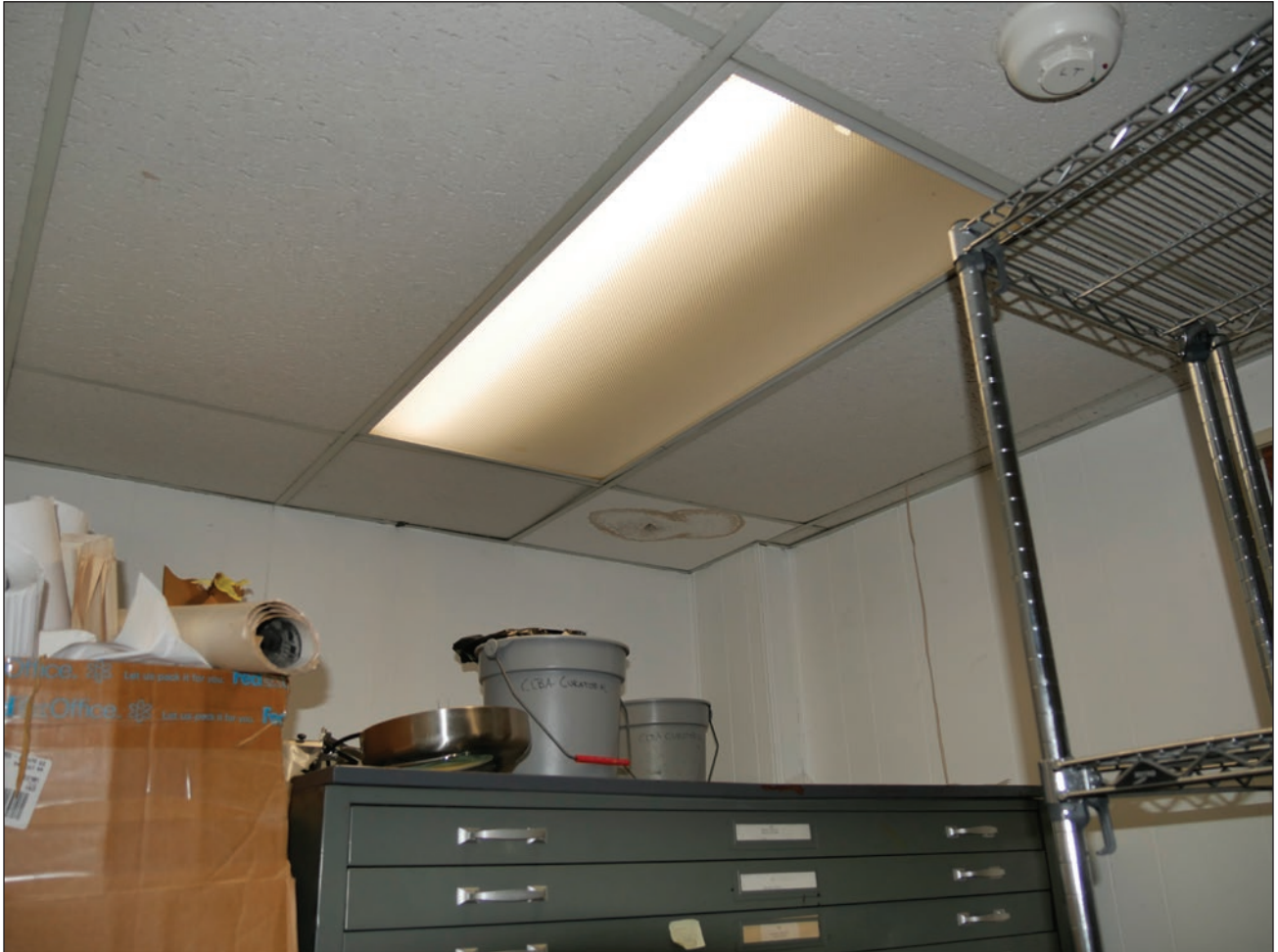
Figure 272. Water damage at suspended ACT in first floor southeast room. Building Conservation Associates, 2025.
