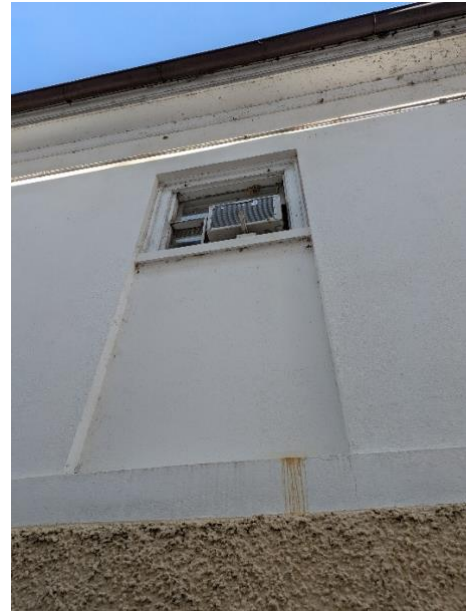
Photo M 010: Window AC Unit
