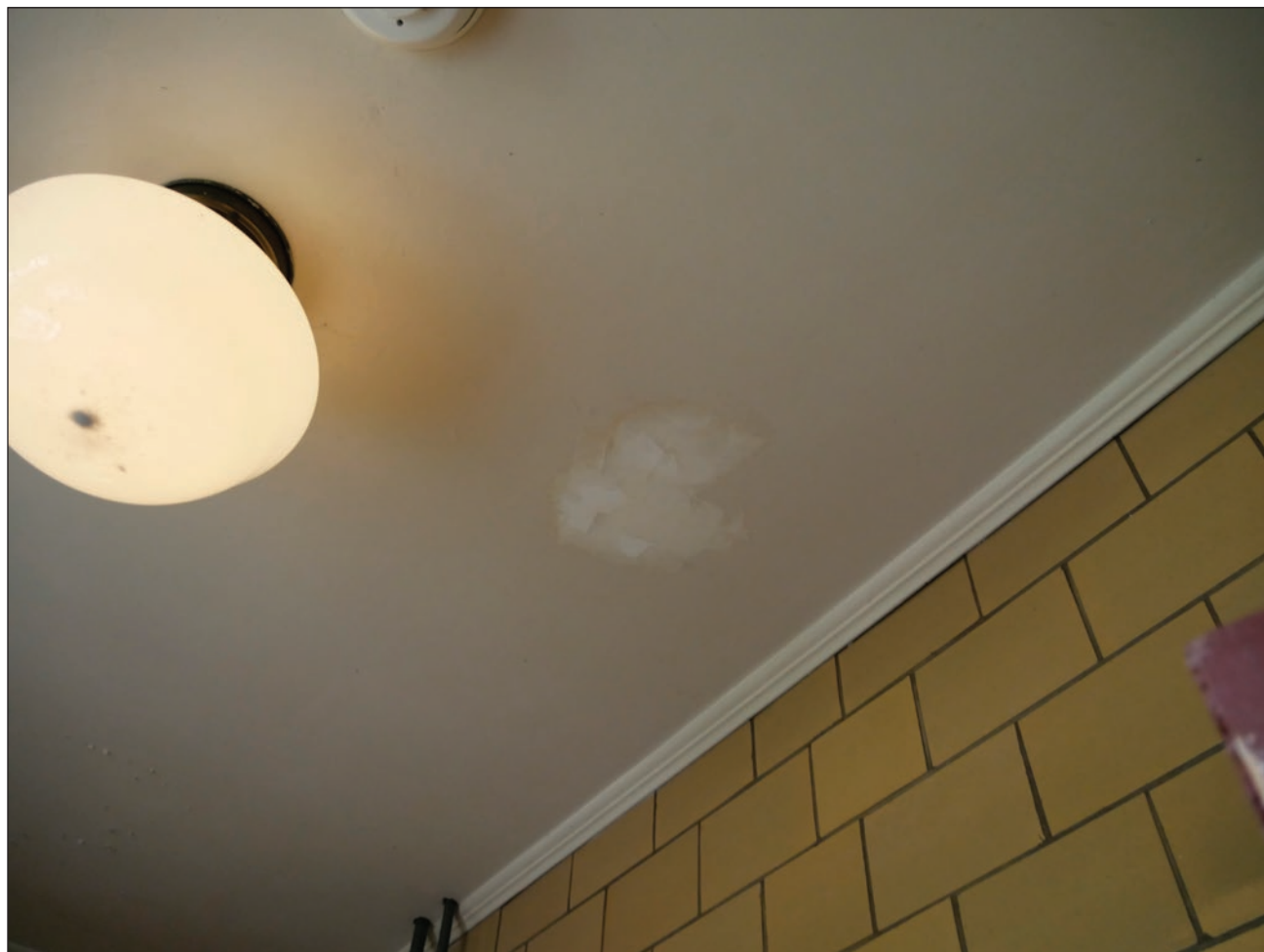
Figure 267. Water damage and paint loss at vestibule ceiling. Building Conservation Associates, 2025.
