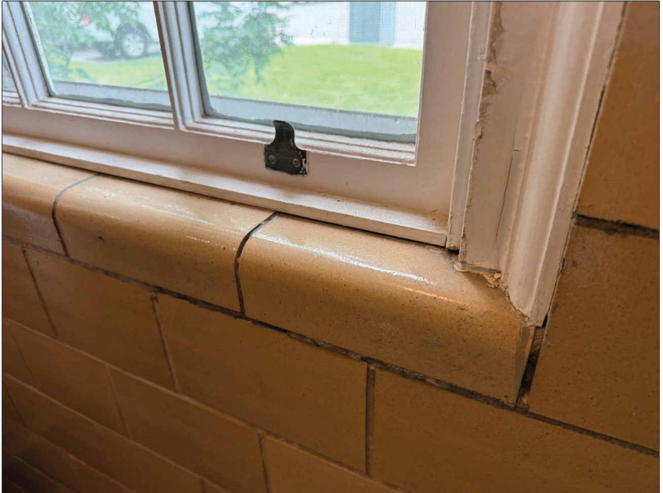
Figure 262. Grout loss at glazed tile in vestibule. Building Conservation Associates, 2025.
