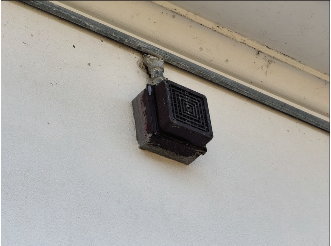
Figure 157. Detail of the SelecTone® speaker below the west cornice. Building Conservation Associates, 2025.
