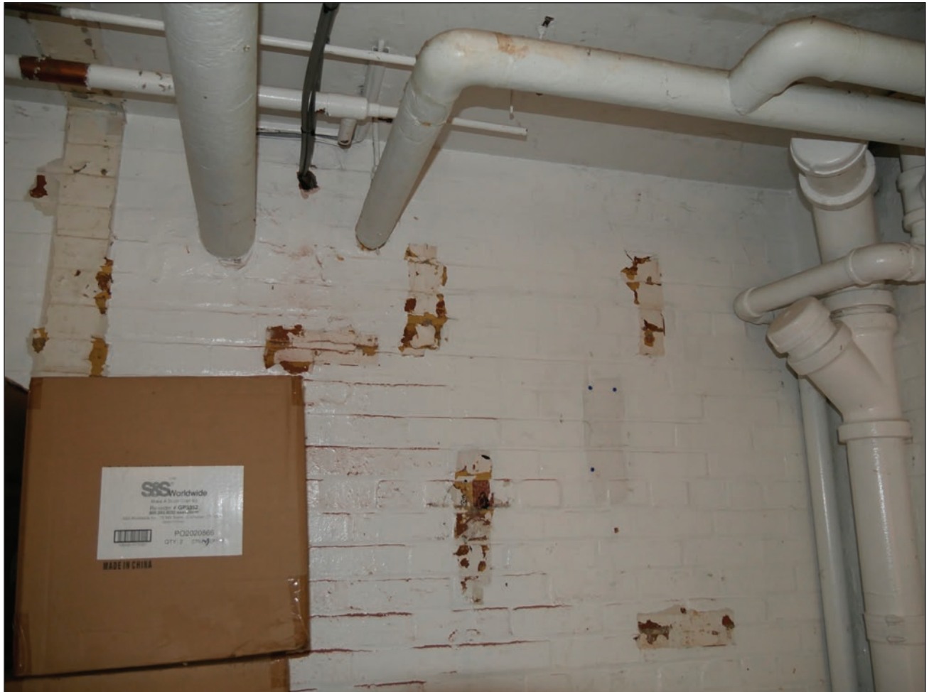
Figure 250. Paint loss at southeast basement room. Building Conservation Associates, 2025.
