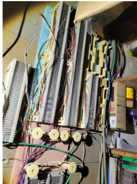
Photo E22: Wall-mounted inactive telephone backboard.
