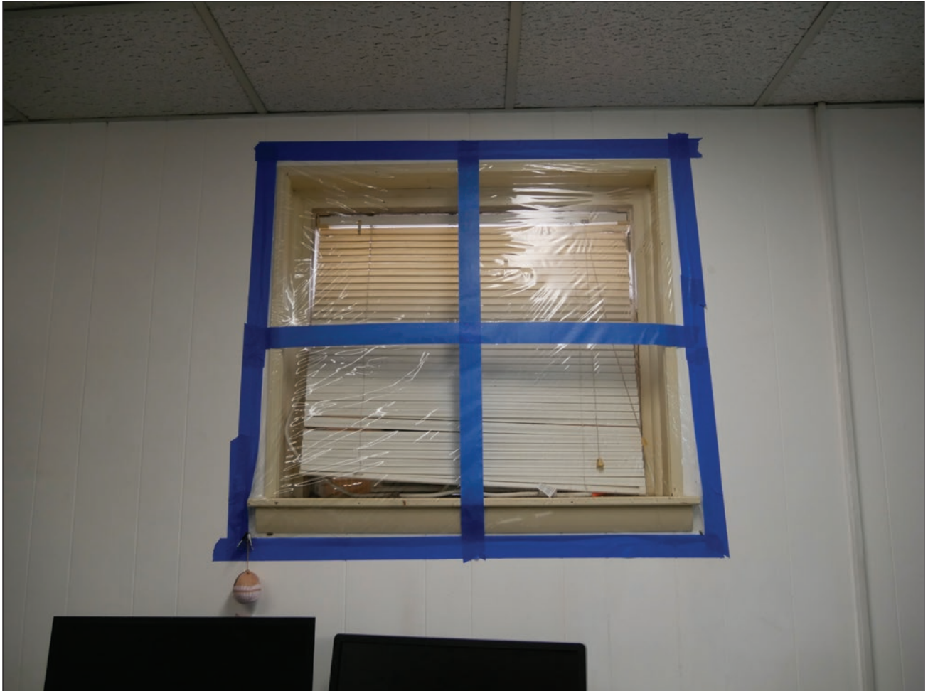
Figure 220. Window at south elevation sealed with plastic and tape. Building Conservation Associates, 2025.
