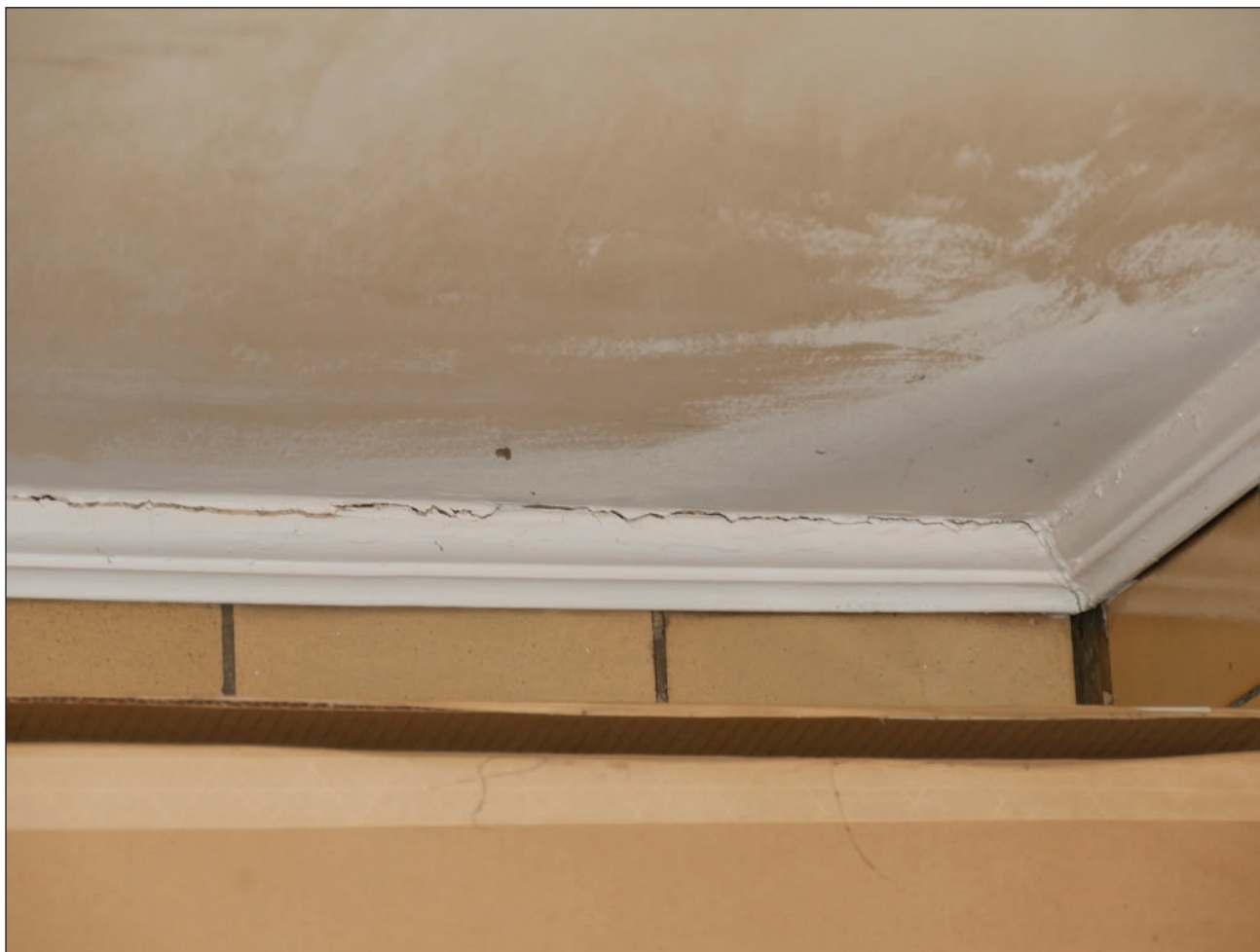
Figure 271. Crack at seam between plaster ceiling and wood trim in first floor east room. Building Conservation Associates, 2025.
