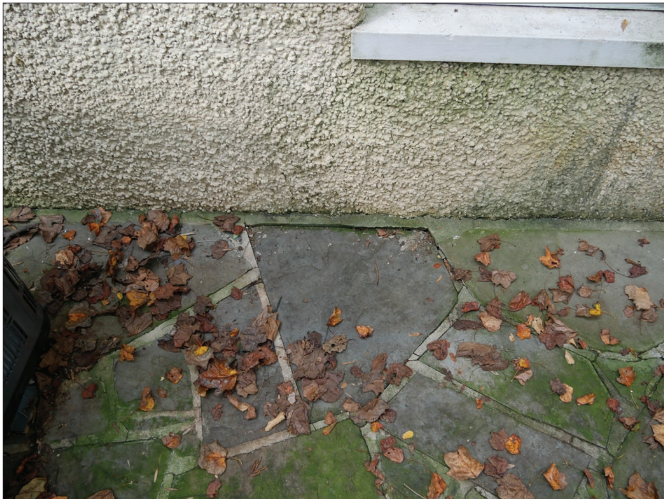
Figure 225. Stains from biological growth at the east patio. Building Conservation Associates, 2025.
