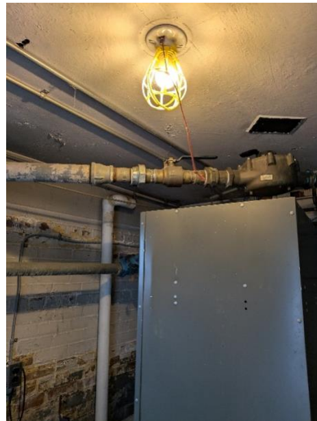
Photo P 002: Water Meter
