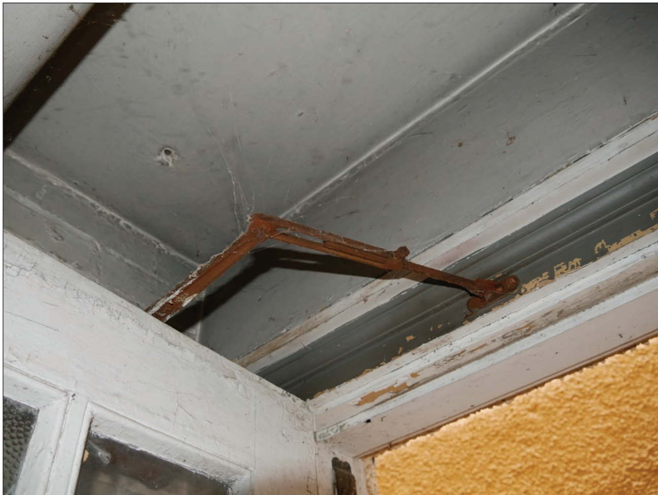
Figure 235. Rusted hardware at southwest basement door. Building Conservation Associates, 2025.
