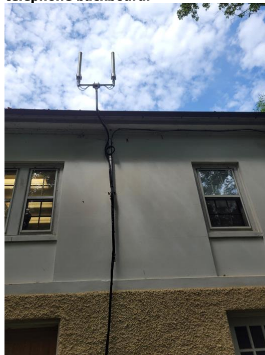
Photo E24: Roof and pole-mounted antennas providing building data service.
