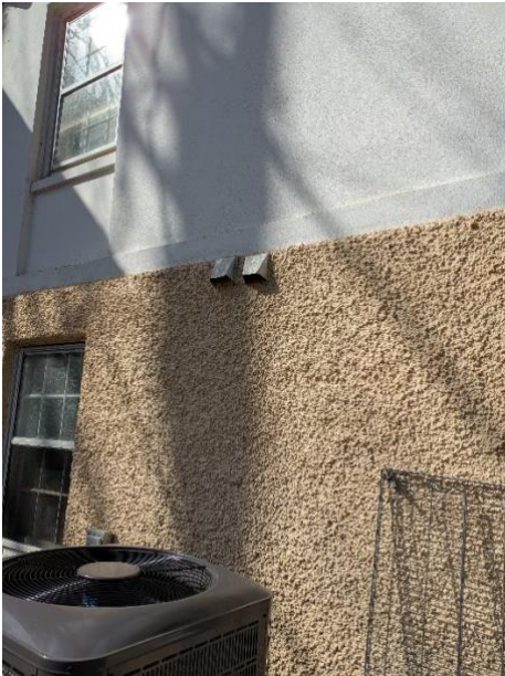
Photo M 019: Abandoned Exhaust Vents
