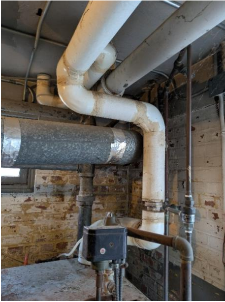
Photo M 015: Boiler Piping
