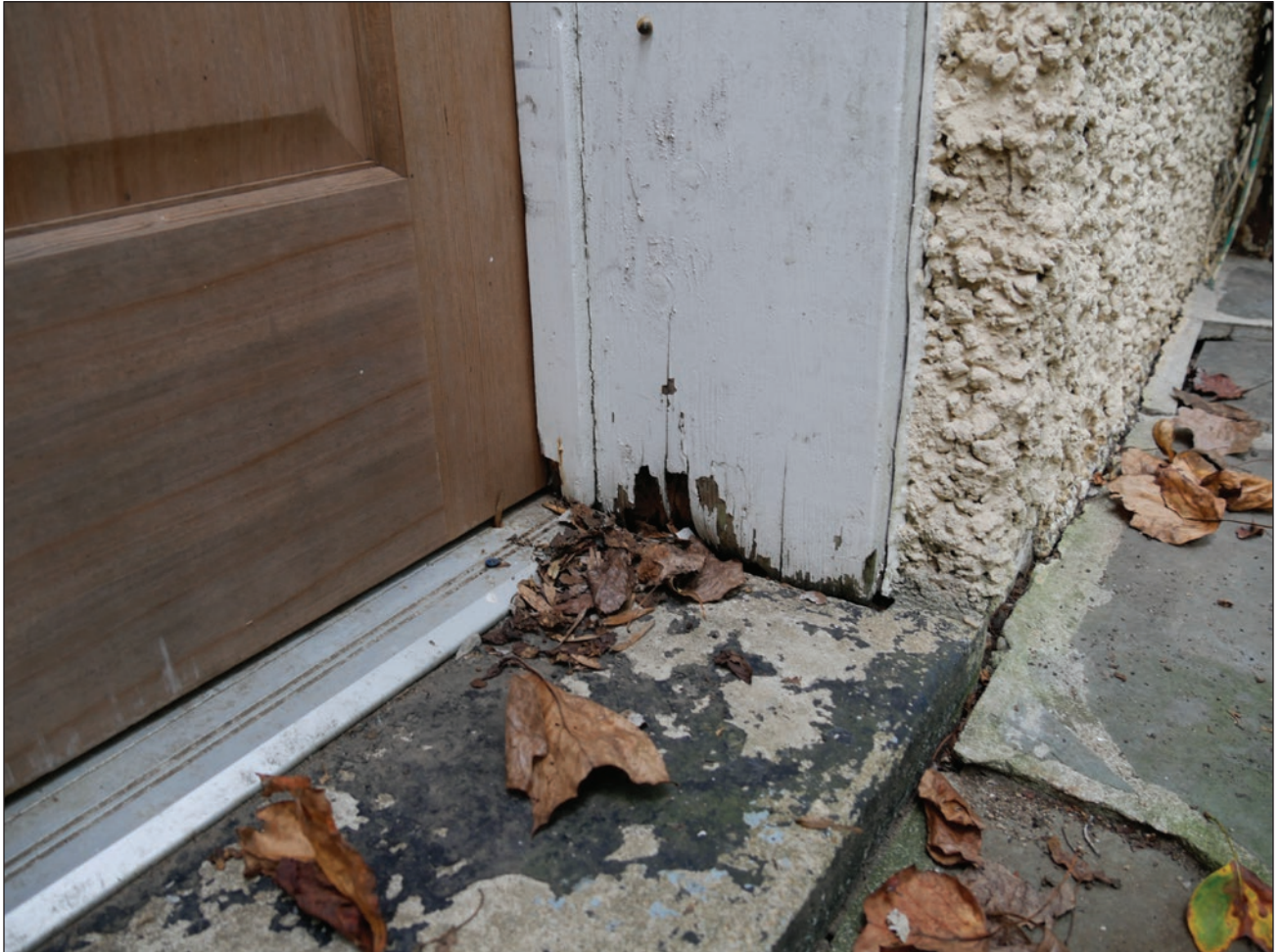
Figure 238. Wood loss at east basement door surround. Building Conservation Associates, 2025.
