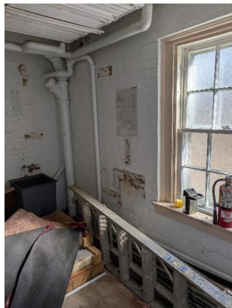
Photo P 006: Abandoned Sanitary Stack
