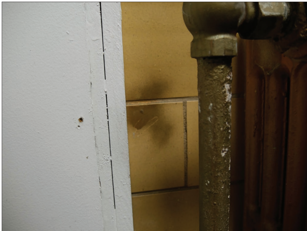
Figure 263. Overpaint on glazed tile wall in north office. Building Conservation Associates, 2025.
