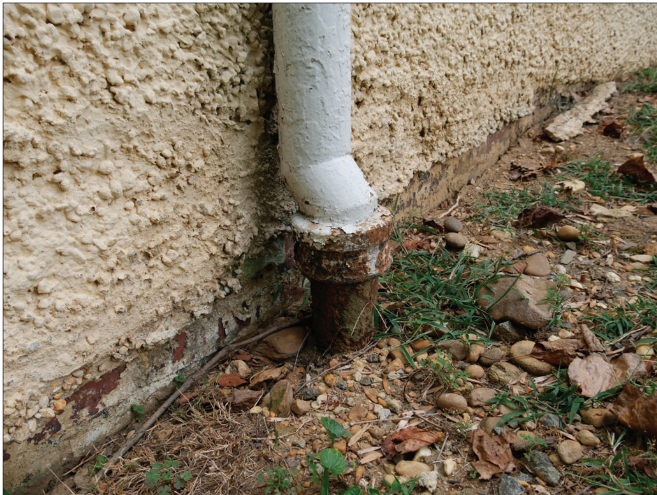
Figure 241. Rusting cast-iron shoe at northeast corner. Building Conservation Associates, 2025.
