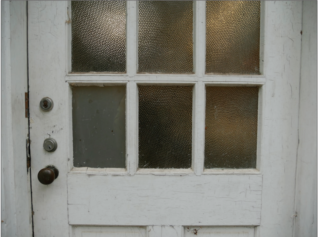
Figure 234. Replacement glass pane, non-historic hardware, and paint failure at northeast basement door. Building Conservation Associates, 2025.
