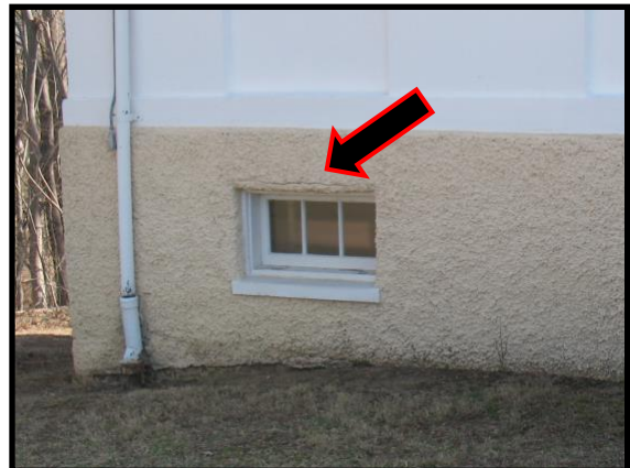
Photo P-20: Crack above window – west building elevation
