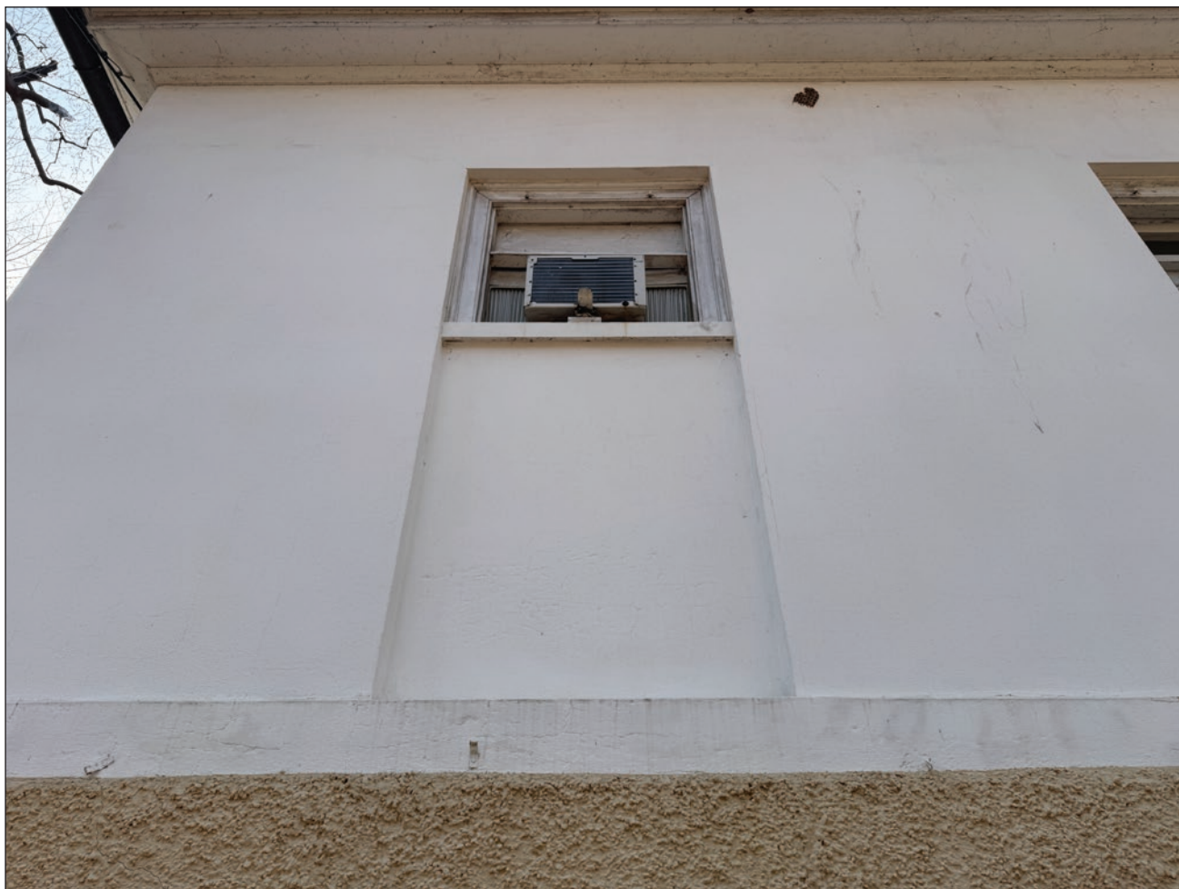
Figure 150. Window A/C unit installed in the east first floor window on the north elevation. Building Conservation Associates, 2025.
