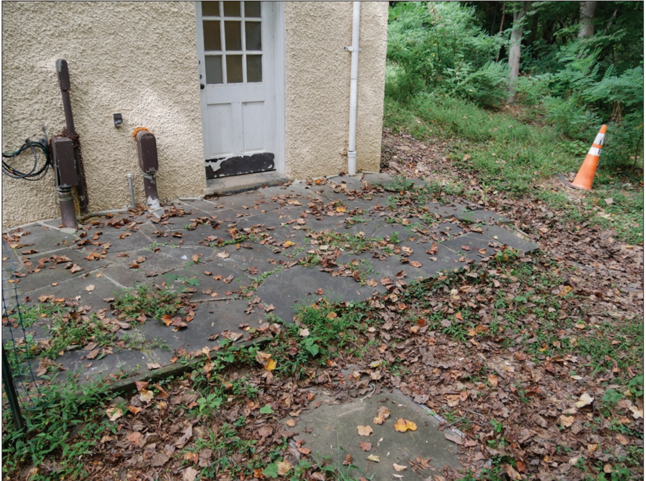
Figure 226. Missing wood edging at east patio. Building Conservation Associates, 2025.
