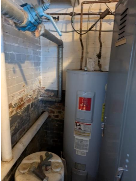
Photo P 003: Domestic Water Heater
