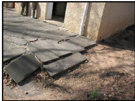
Photo P-22: Deterioration at rear flagstone patio
