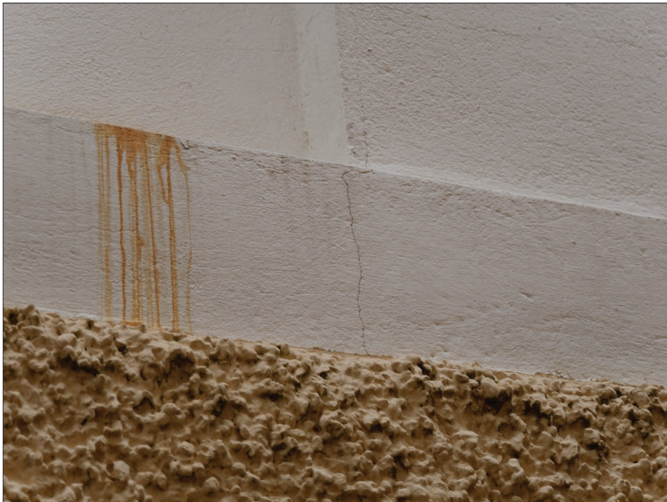
Figure 211. Rust staining at the flat stucco on the south elevation. Also note the narrow crack. Building Conservation Associates, 2025.
