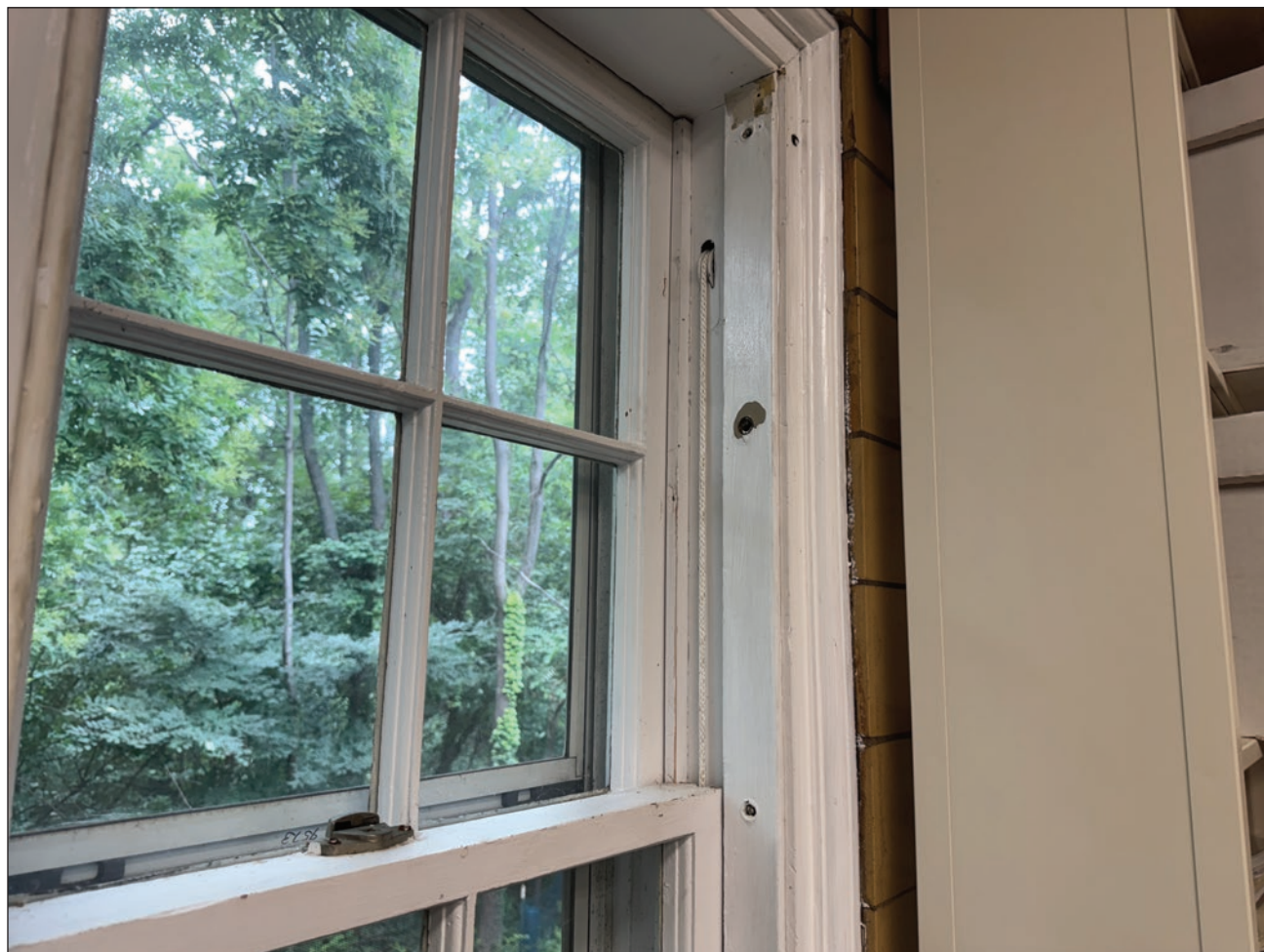
Figure 199. Abandoned anchors in the east room's tripartite window frame. Building Conservation Associates, 2025.
