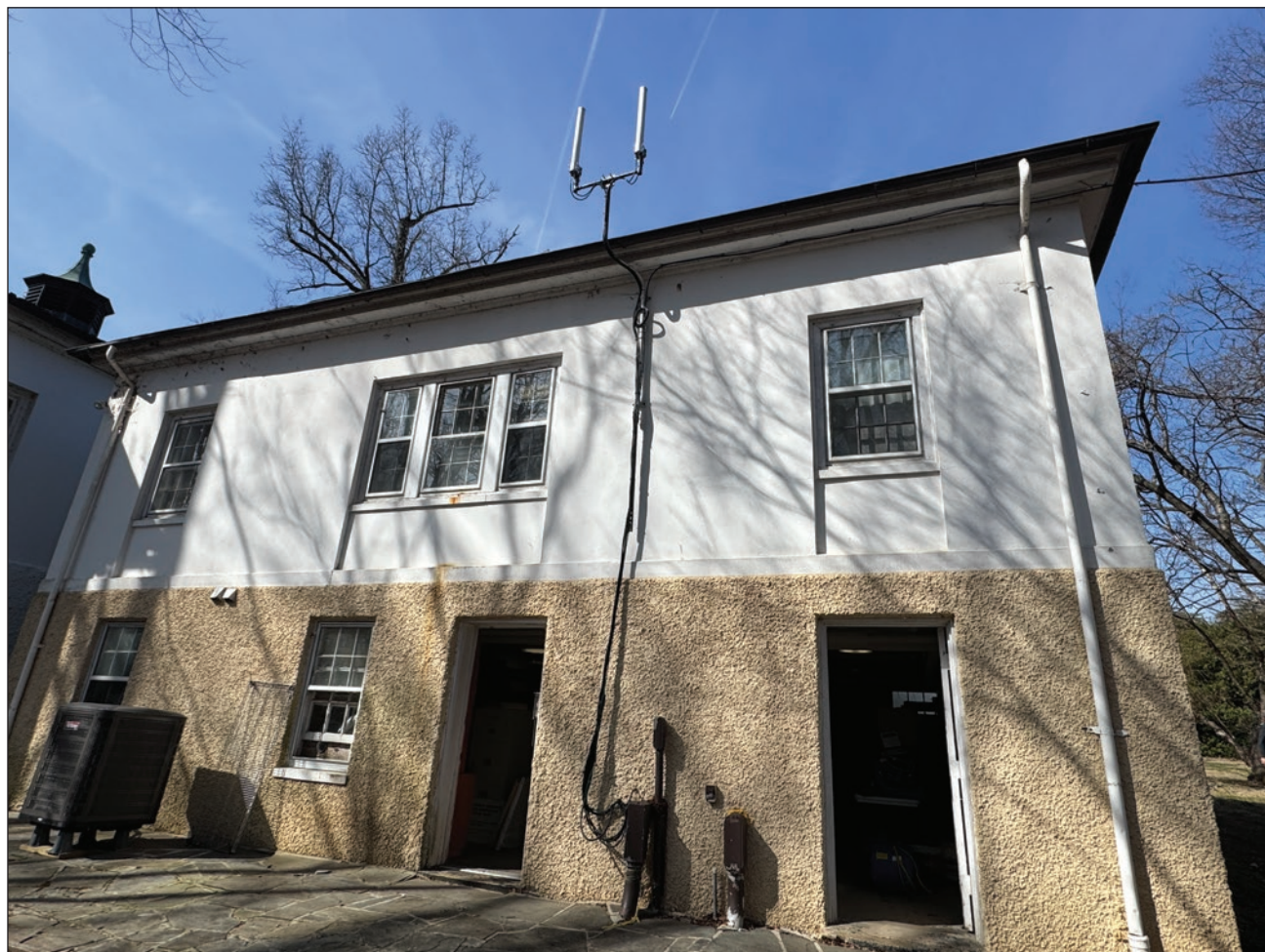
Figure 162. Electrical boxes, conduit, wiring, and an antenna on the east elevation. Building Conservation Associates, 2025.
