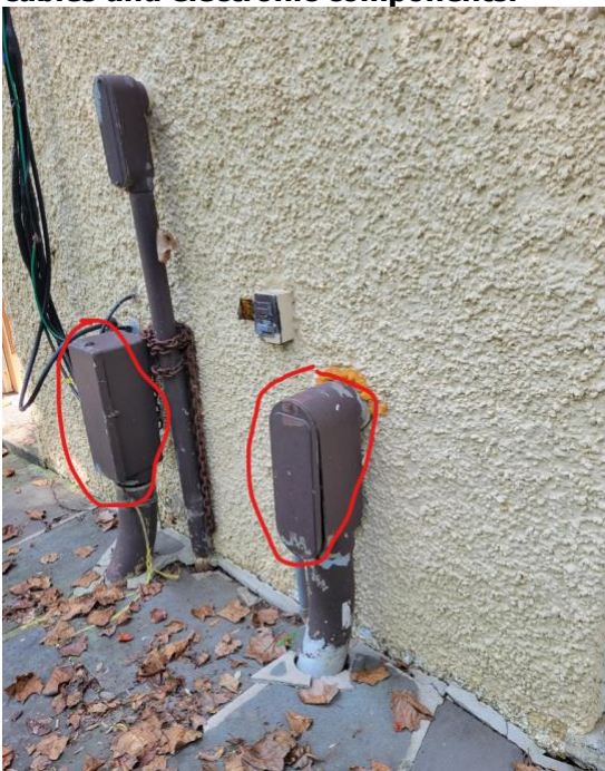
Photo E23: Underground conduit for inactive data service entry.
