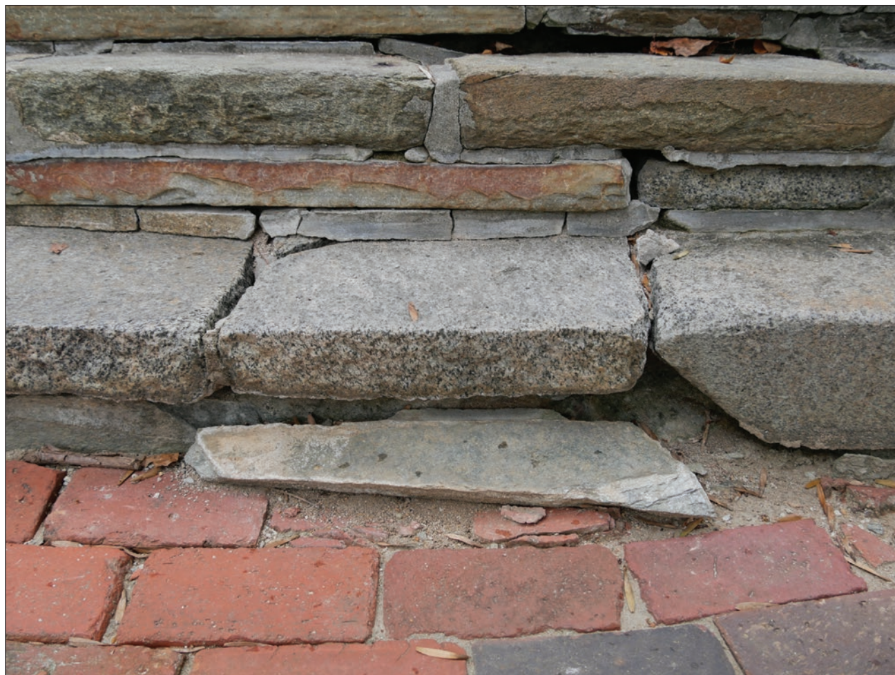
Figure 245. Displaced stone and mortar loss at main entry steps. Building Conservation Associates, 2025.
