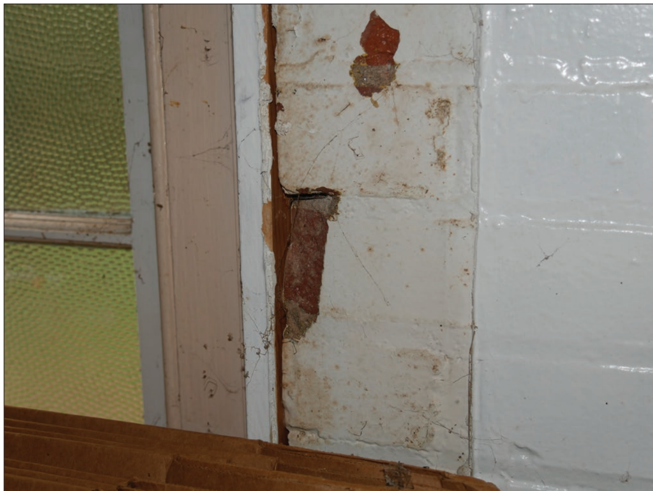
Figure 253. Brick spall at southeast basement room. Building Conservation Associates, 2025.
