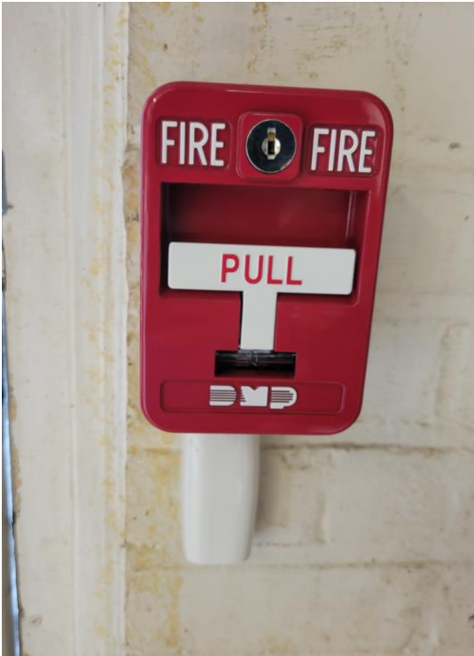
Photo E19: Manual fire alarm pull station mounted near exit door.
