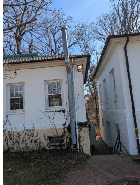
Photo M 012: Boiler Flue
