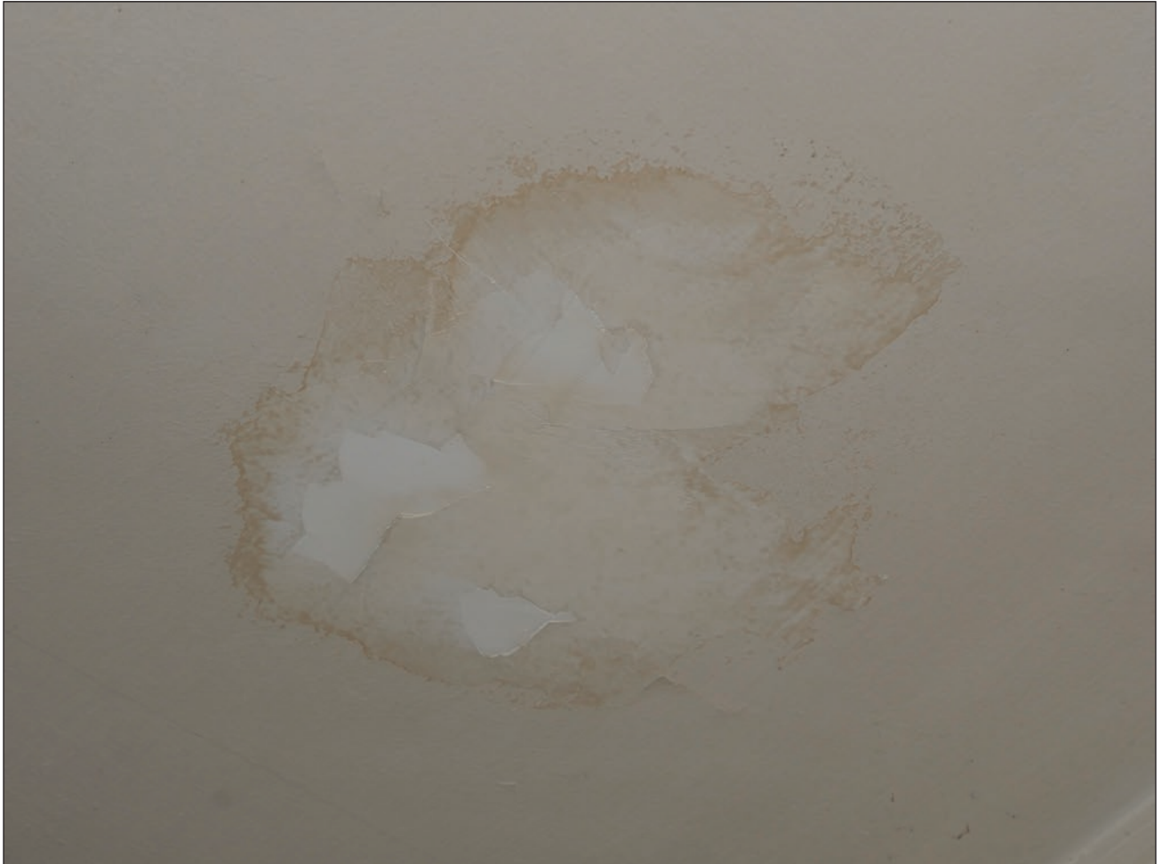
Figure 268. Detail of water damage and paint loss at vestibule ceiling. Building Conservation Associates, 2025.
