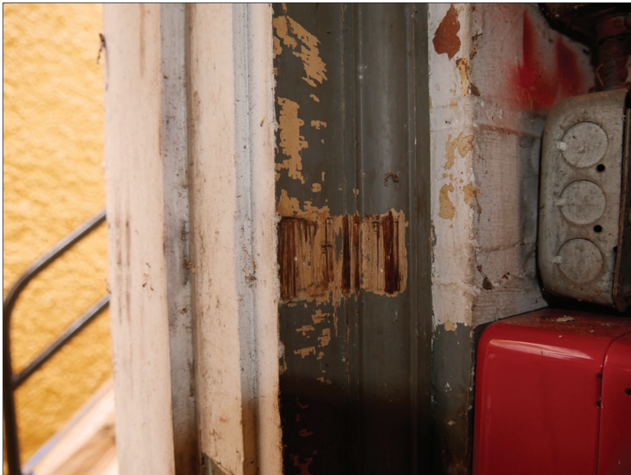
Figure 231. Wood damage and paint loss at interior of southwest basement door. Building Conservation Associates, 2025.
