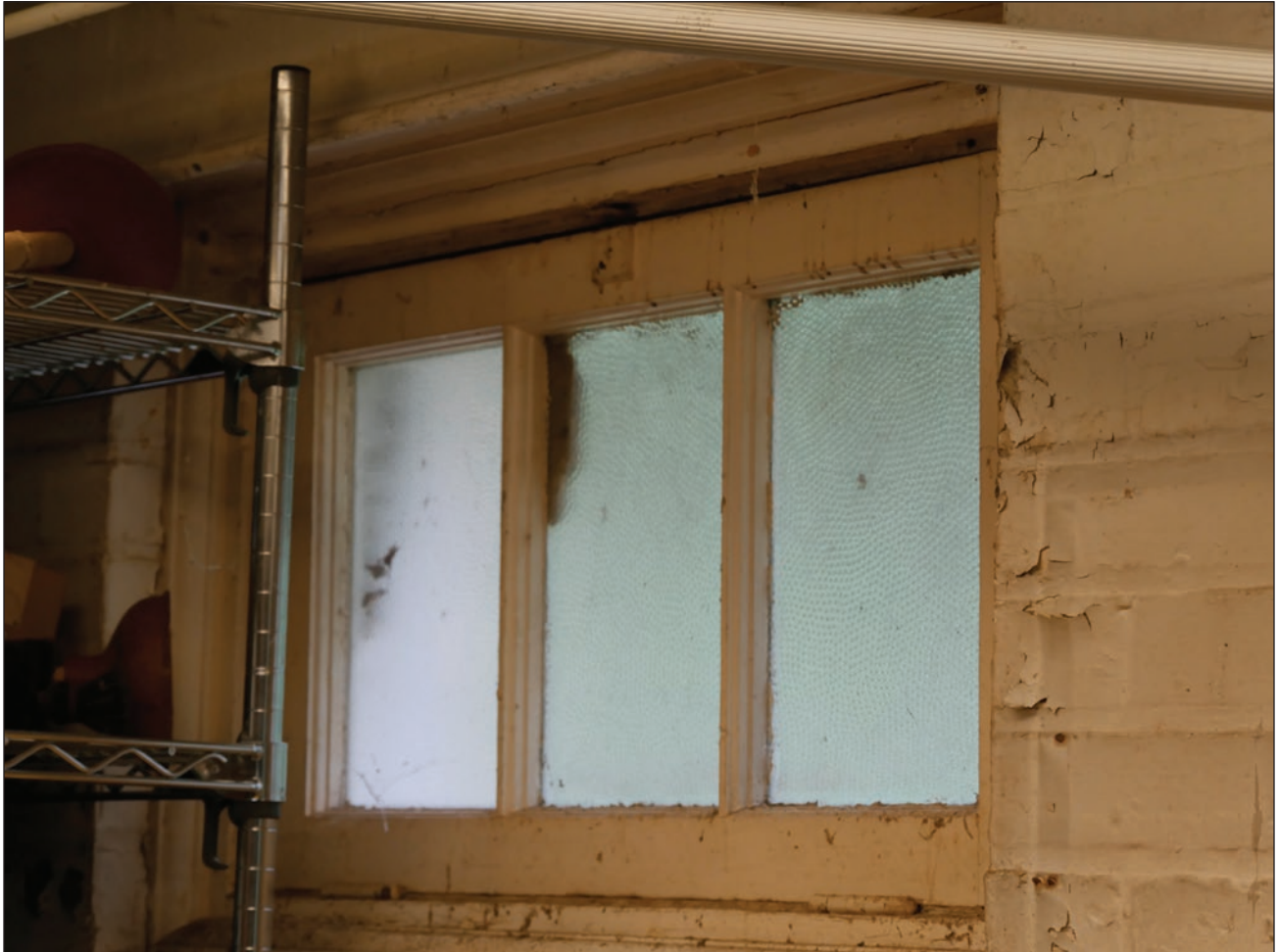
Figure 218. Basement hopper window with general soiling, a replacement glass pane, and missing hardware. Building Conservation Associates, 2025.
