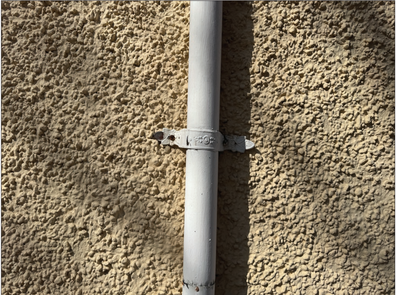
Figure 240. Rusting downspout band at east elevation. Building Conservation Associates, 2025.
