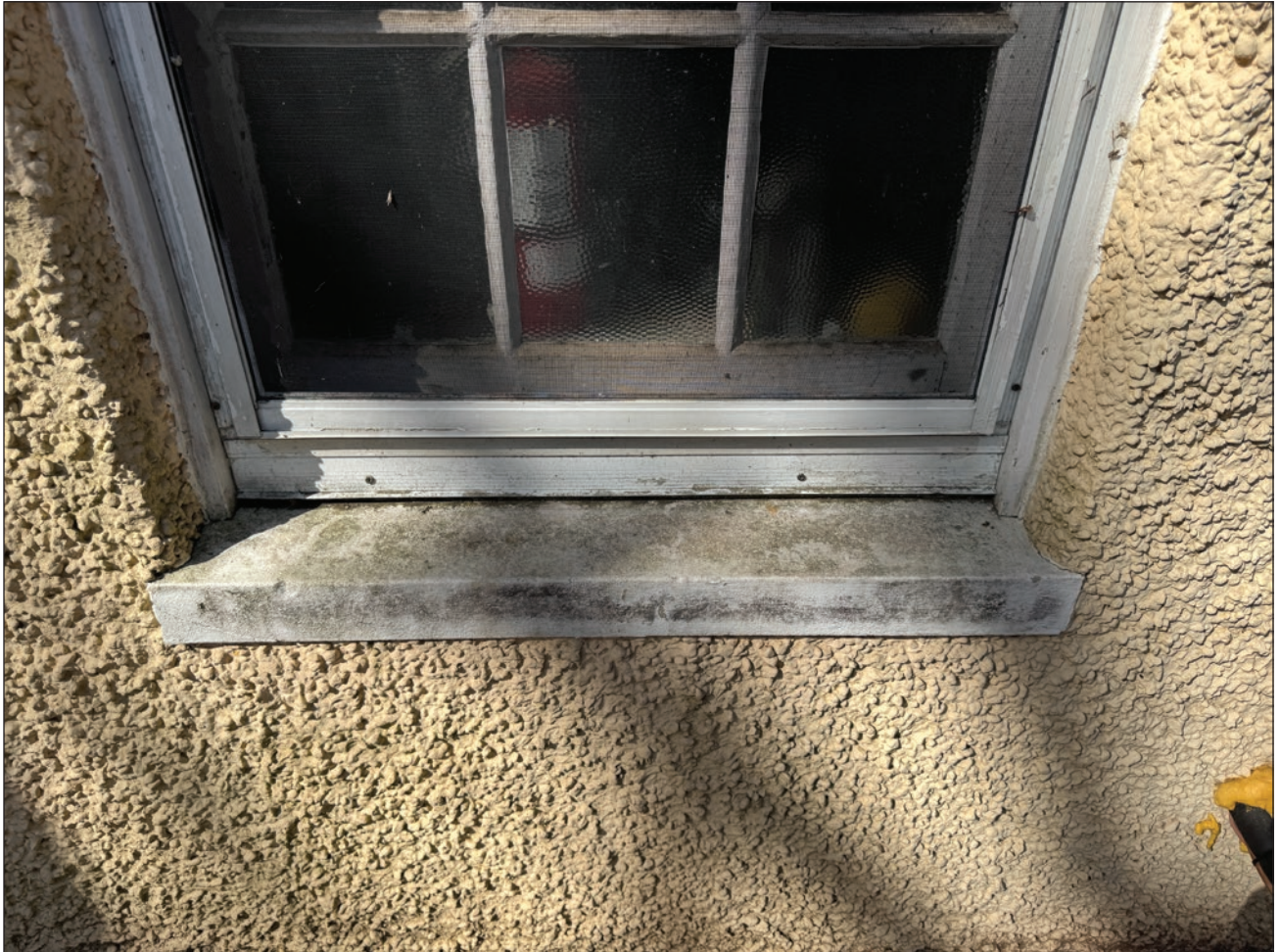
Figure 216. Biological growth and soiling at a window sill on the east elevation. Building Conservation Associates, 2025.
