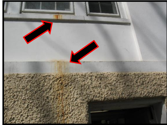
Photo P-18: East building elevation water stains
