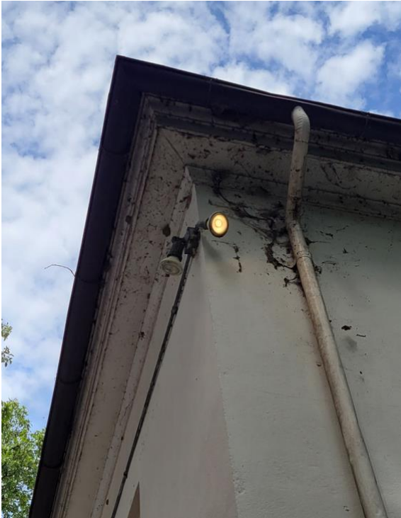
Photo E27: Rear wall security light without motion or photocell control.
