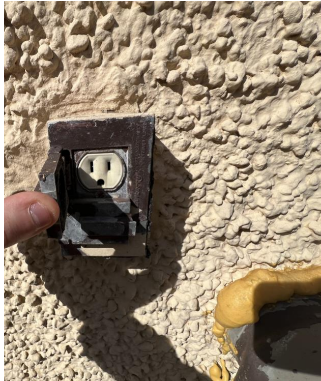
Photo E28: Rear exterior wall receptacle lacking GFCI protection.
