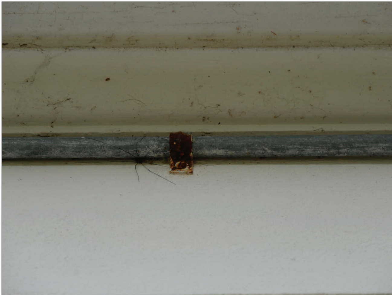
Figure 215. Rusted conduit bracket at the west elevation. Building Conservation Associates, 2025.
