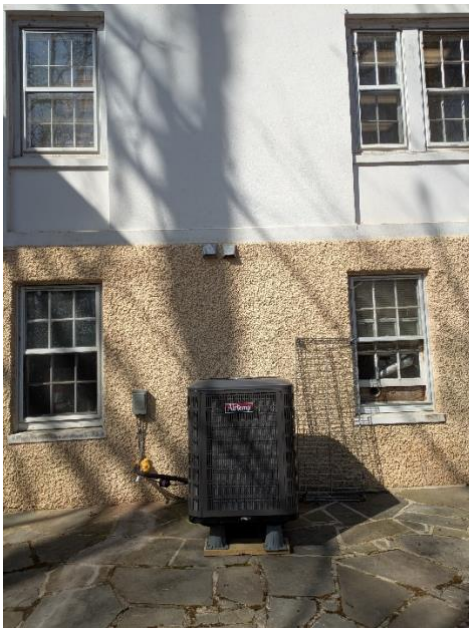
Photo M 001: Heat Pump Unit
