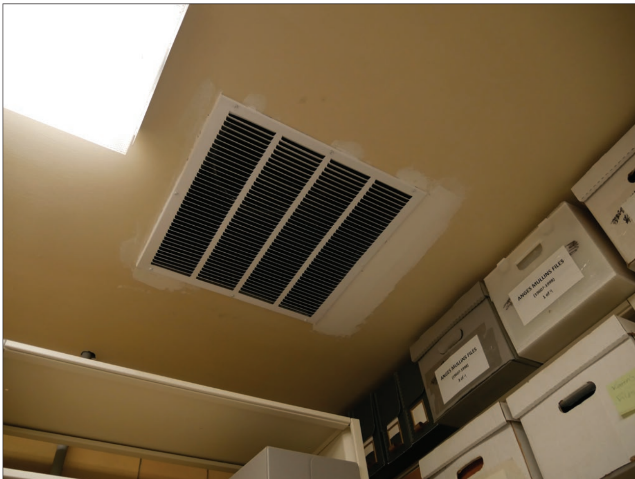
Figure 269. Modern air return in first floor east room. Building Conservation Associates, 2025.
