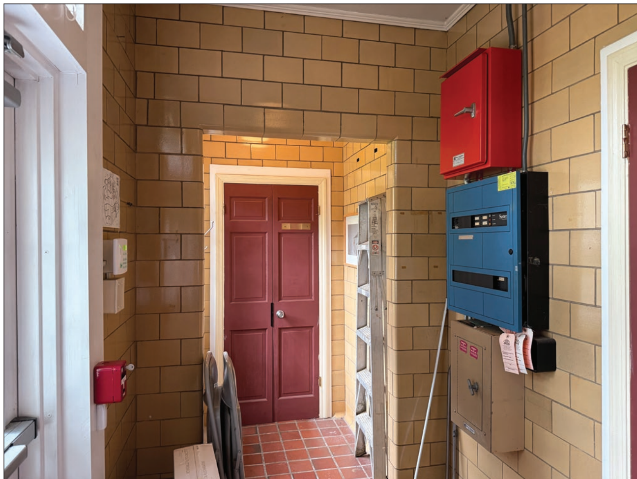
Figure 189. Vestibule looking north. Note the modern electrical and telecommunications equipment. Building Conservation Associates, 2025.
