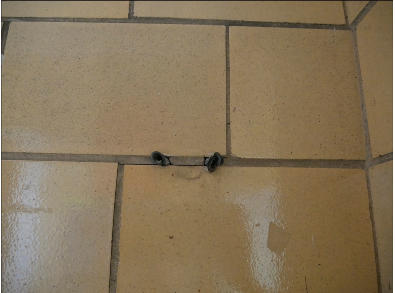
Figure 260. Abandoned anchors in vestibule glazed tile wall. Building Conservation Associates, 2025.
