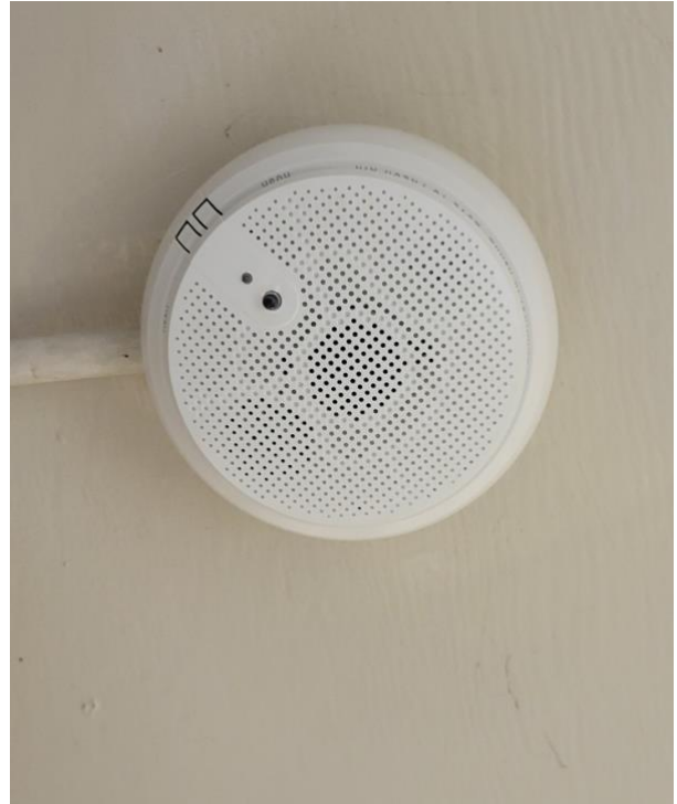
Photo E20: Ceiling-mounted smoke detector with integrated sounder.
