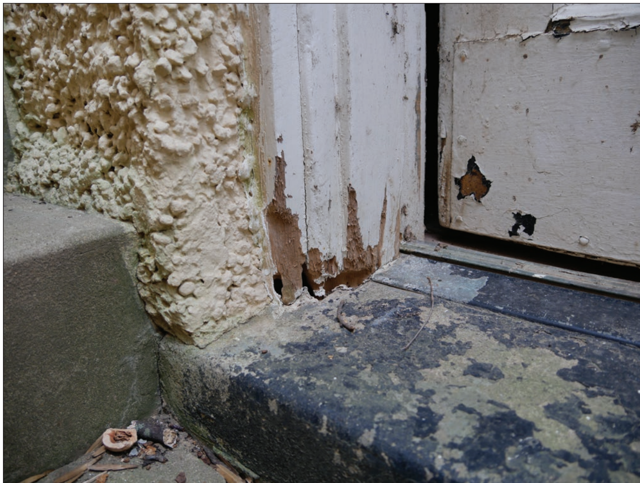
Figure 207. Heavy paint at pebble dash and wood loss at southwest basement door surround. Building Conservation Associates, 2025.
