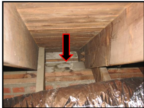
Photo P-16: Water stains on framing at location of repaired roof
