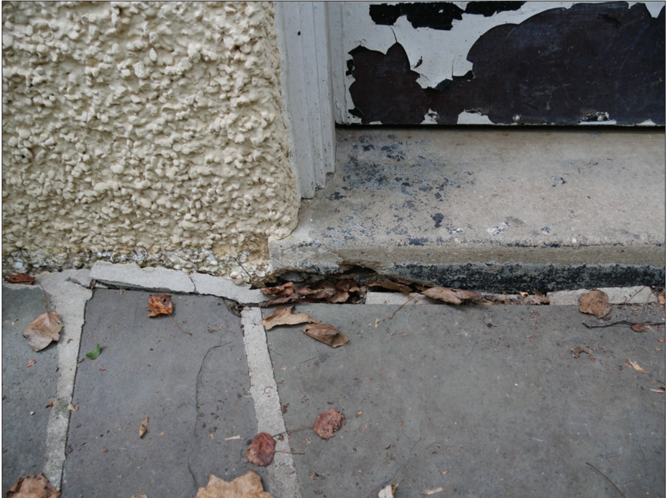
Figure 224. Displaced flagstones and damaged mortar at the east patio. Building Conservation Associates, 2025.
