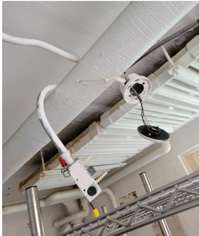
Photo E09: Loose junction boxes with visible conductors.
