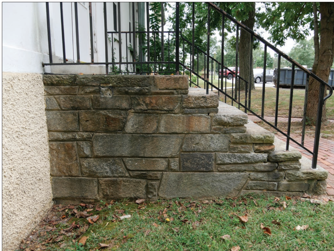
Figure 247. Heavy soiling at north side of main entry steps. Building Conservation Associates, 2025.
