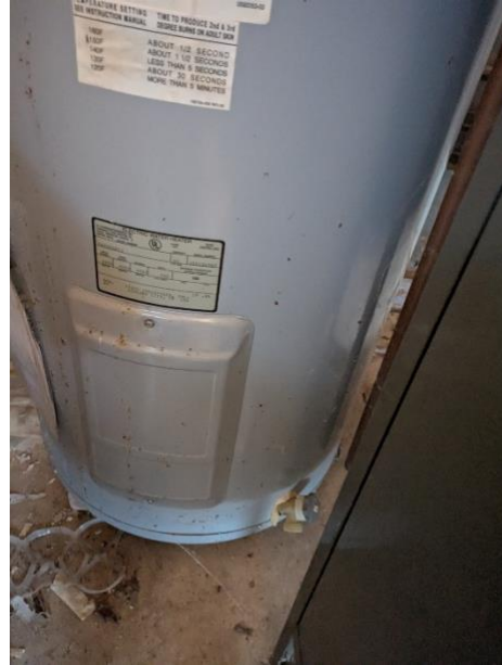
Photo P 004: Domestic Water Heater
