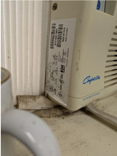
Photo M 007: Window AC Unit
