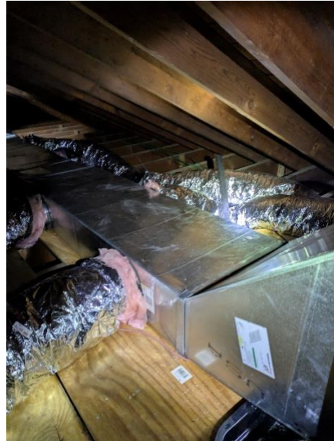
Photo M 004: Ductwork
