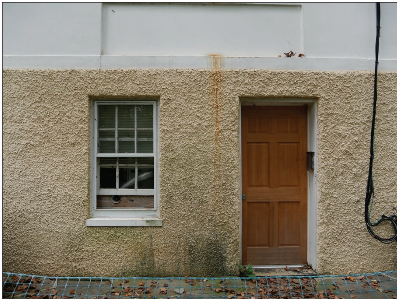
Figure 205. General soiling, biological growth, and rust staining on the pebble dash stucco at the east elevation. Building Conservation Associates, 2025.
