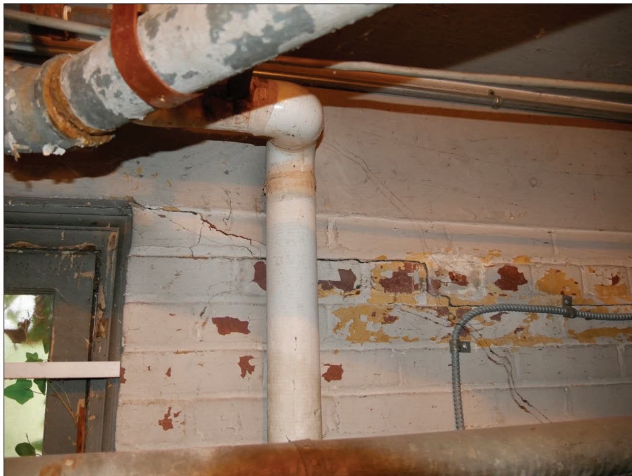
Figure 251. Brick cracking at southwest basement room. Building Conservation Associates, 2025.
