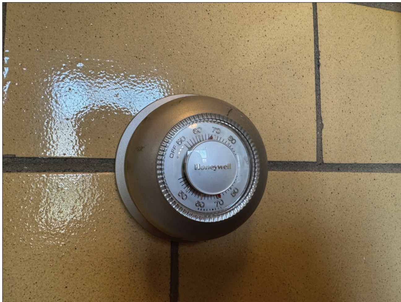
Figure 187. Honeywell T87 thermostat in vestibule. Building Conservation Associates, 2025.
