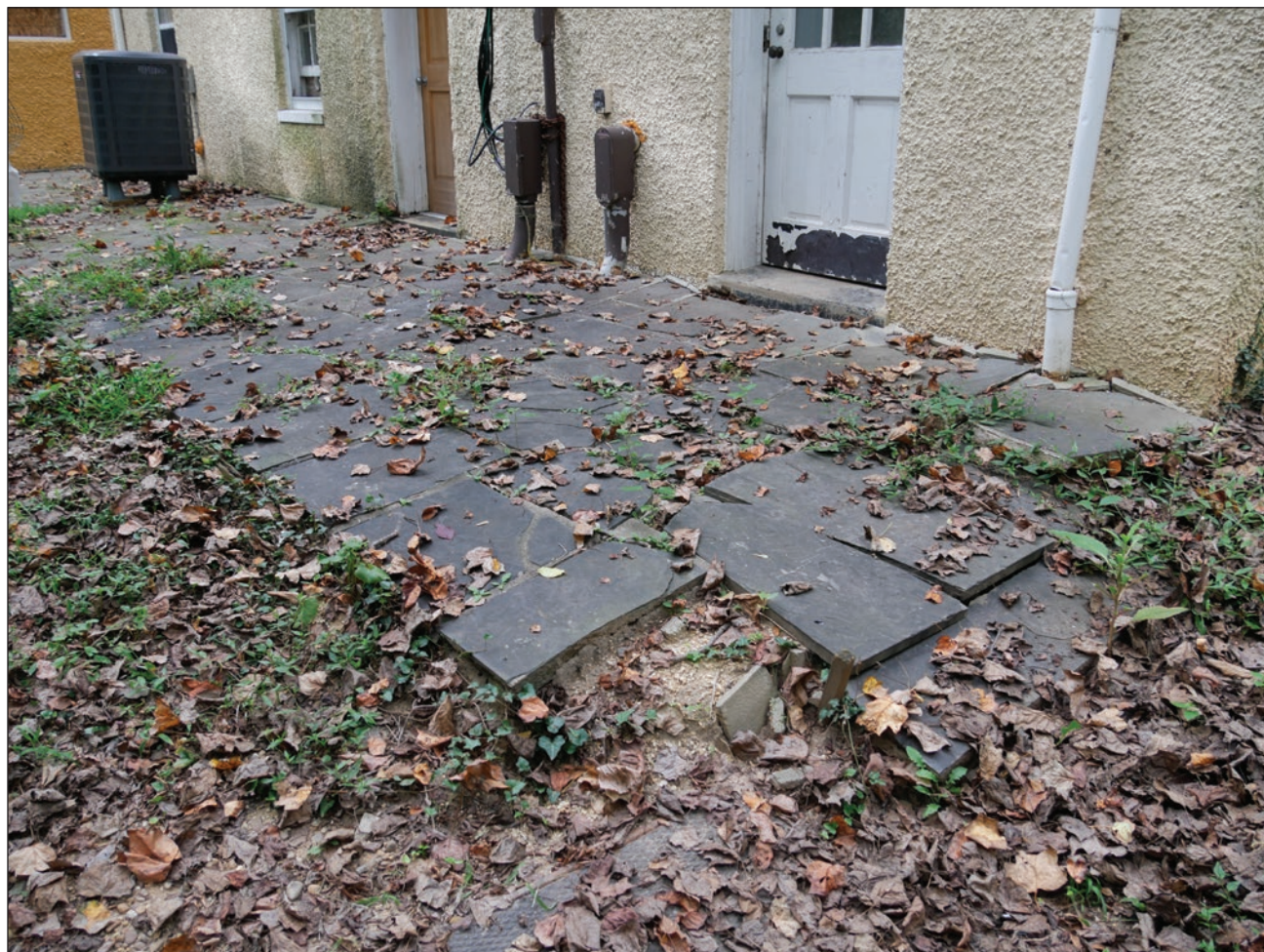
Figure 223. Displaced flagstones at the east patio. Building Conservation Associates, 2025.
