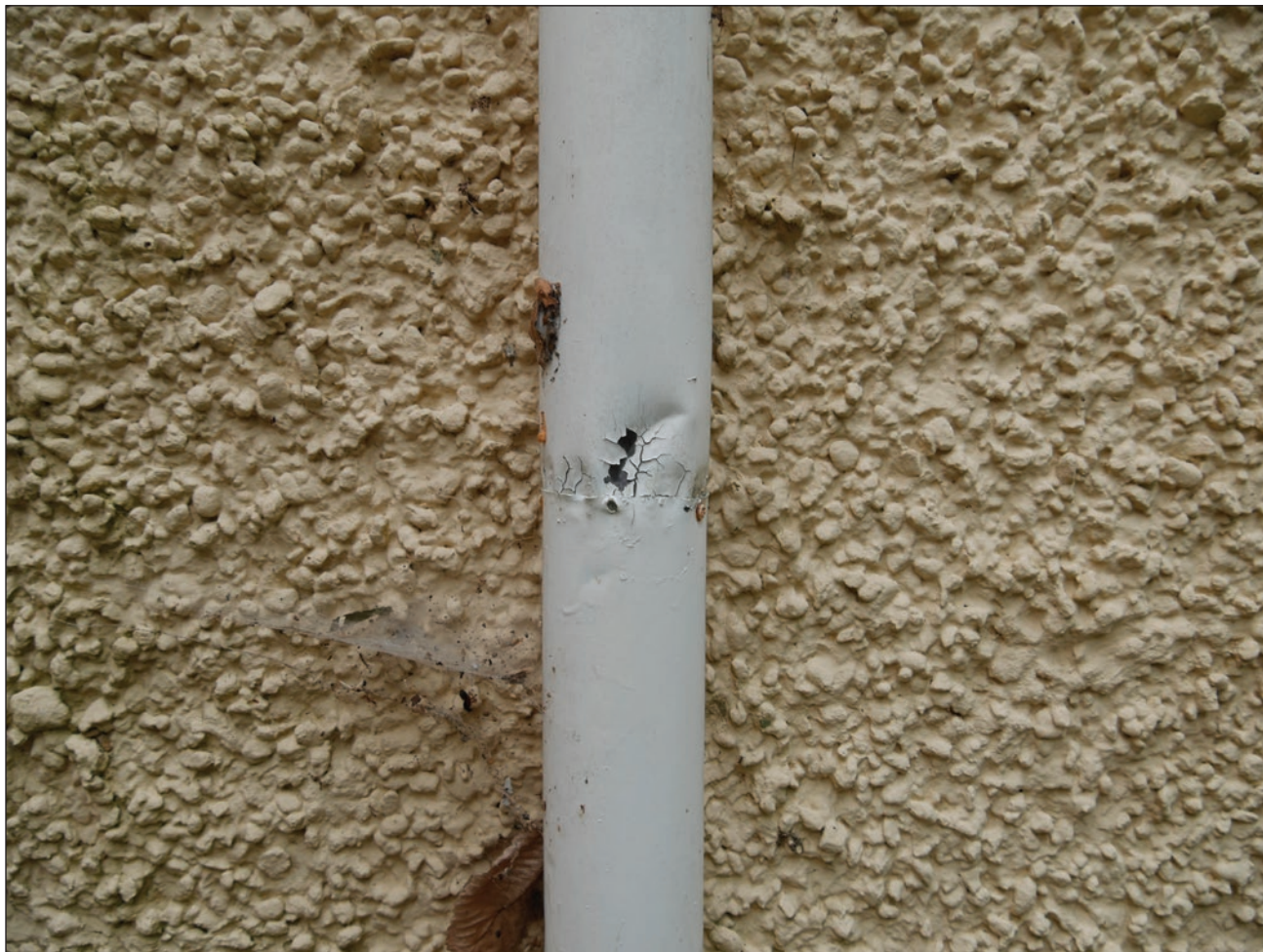
Figure 239. Dent and paint loss at downspout. Building Conservation Associates, 2025.
