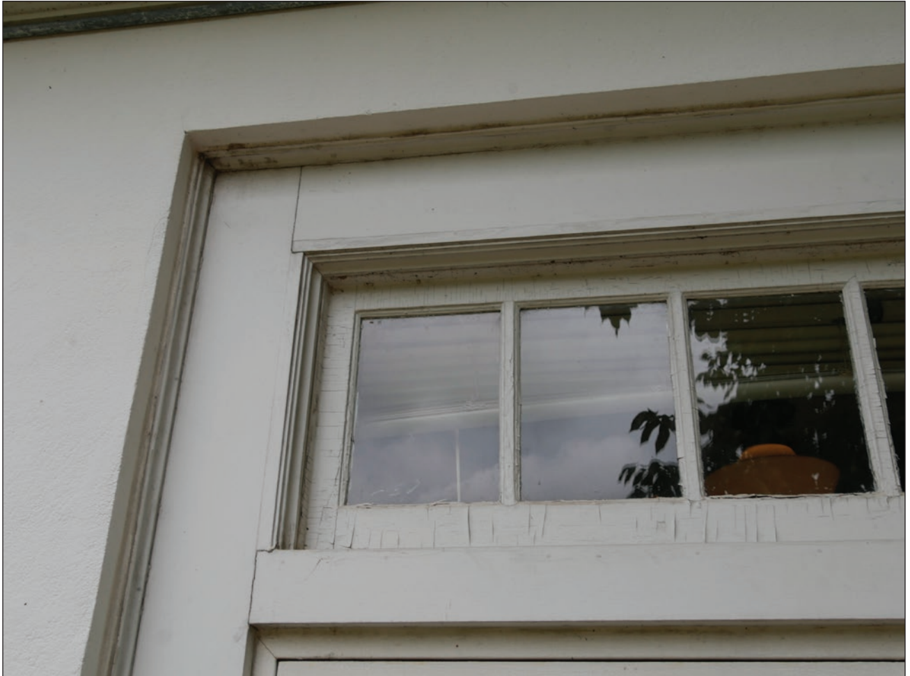
Figure 222. Failing paint at the west transom window. Building Conservation Associates, 2025.
