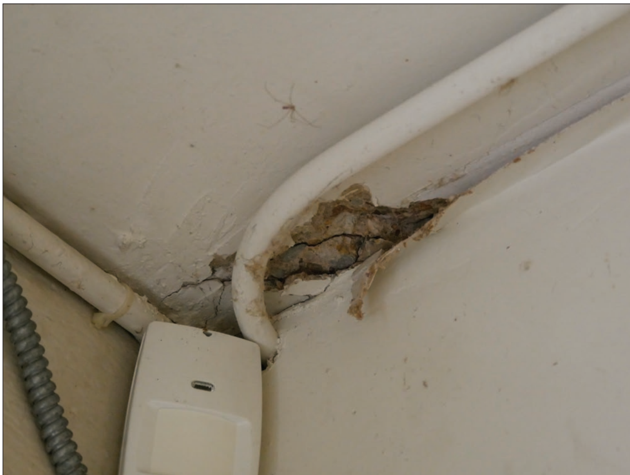
Figure 265. Cracked plaster ceiling in basement. Building Conservation Associates, 2025.
