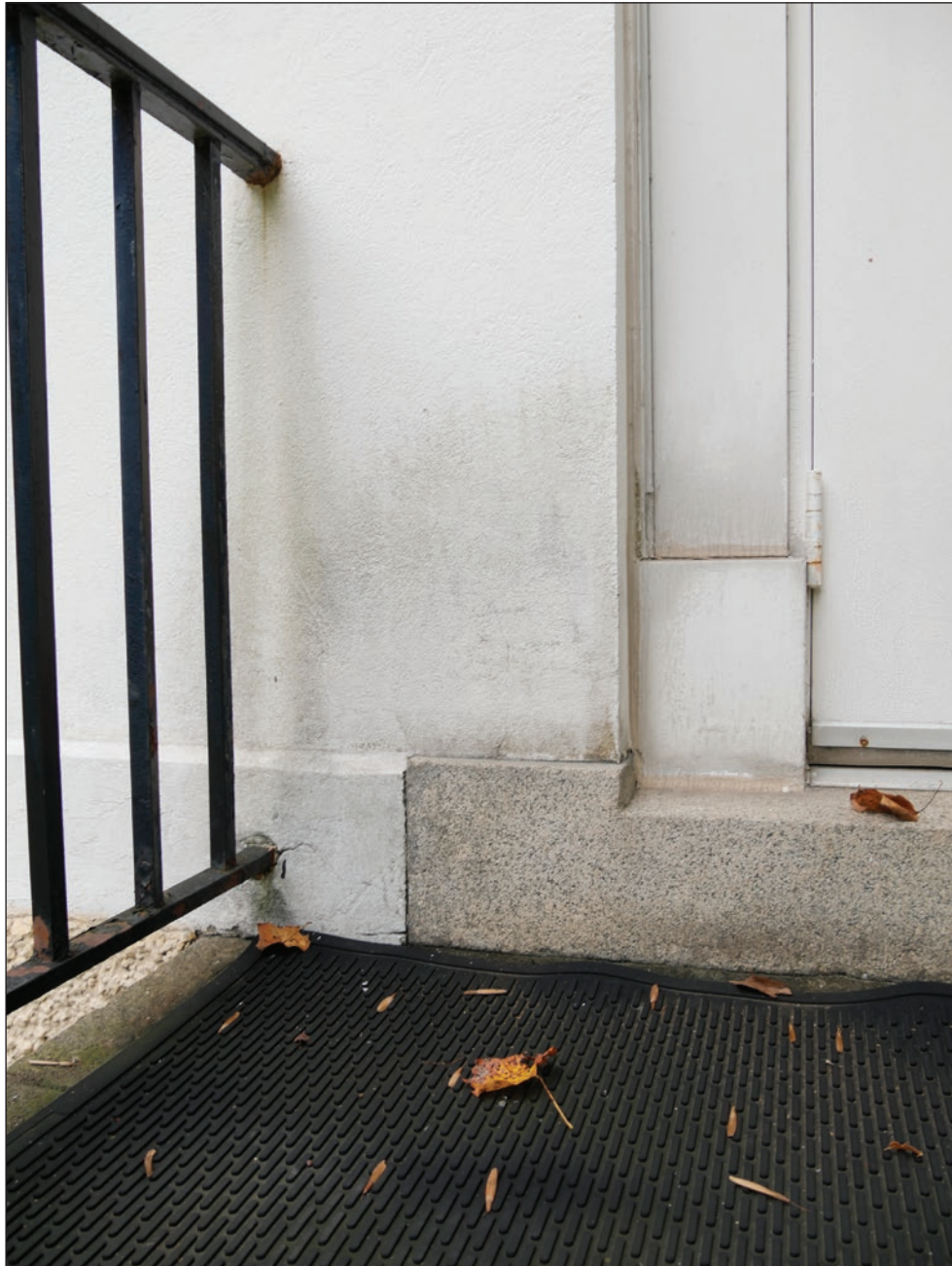
Figure 214. Cracking and rust staining at the railing penetration in the flat stucco on the west elevation. Building Conservation Associates, 2025.
