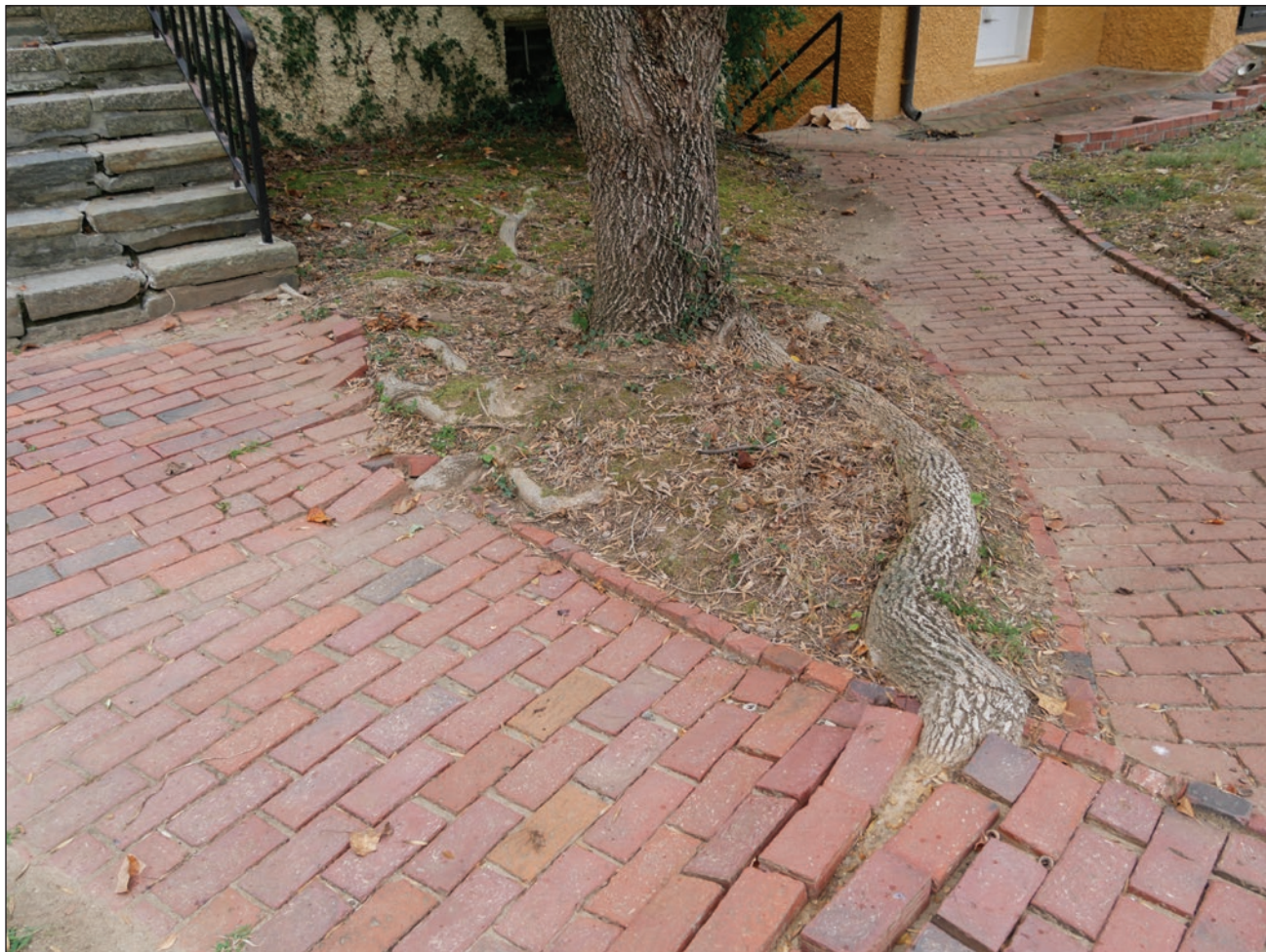
Figure 227. Displaced brick, lost edging, and mortar loss at brick path. Building Conservation Associates, 2025.
