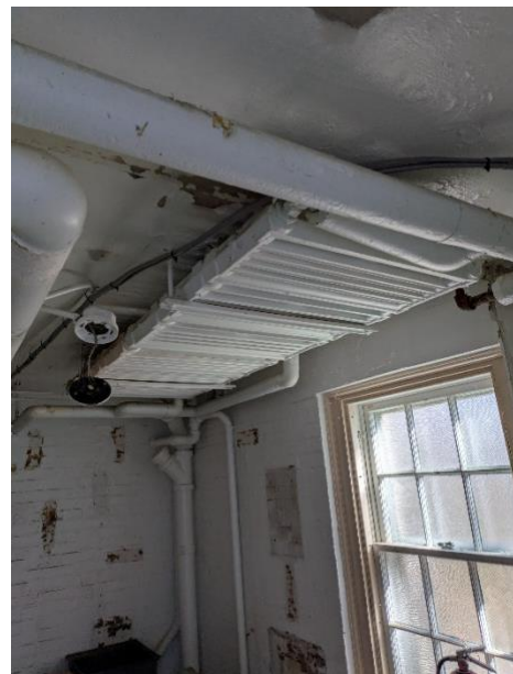
Photo M 014: Basement Radiator
