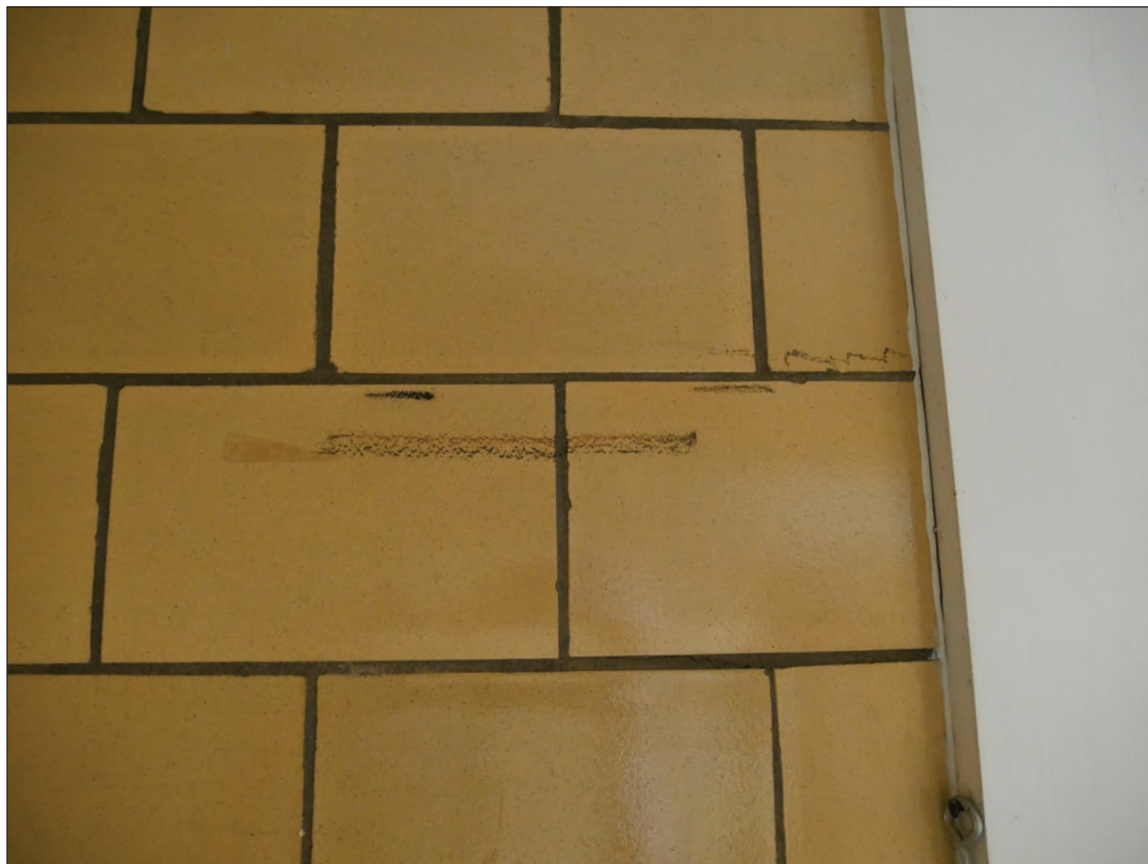
Figure 261. Surface marks and adhesive residue on glazed tile wall in vestibule. Building Conservation Associates, 2025.
