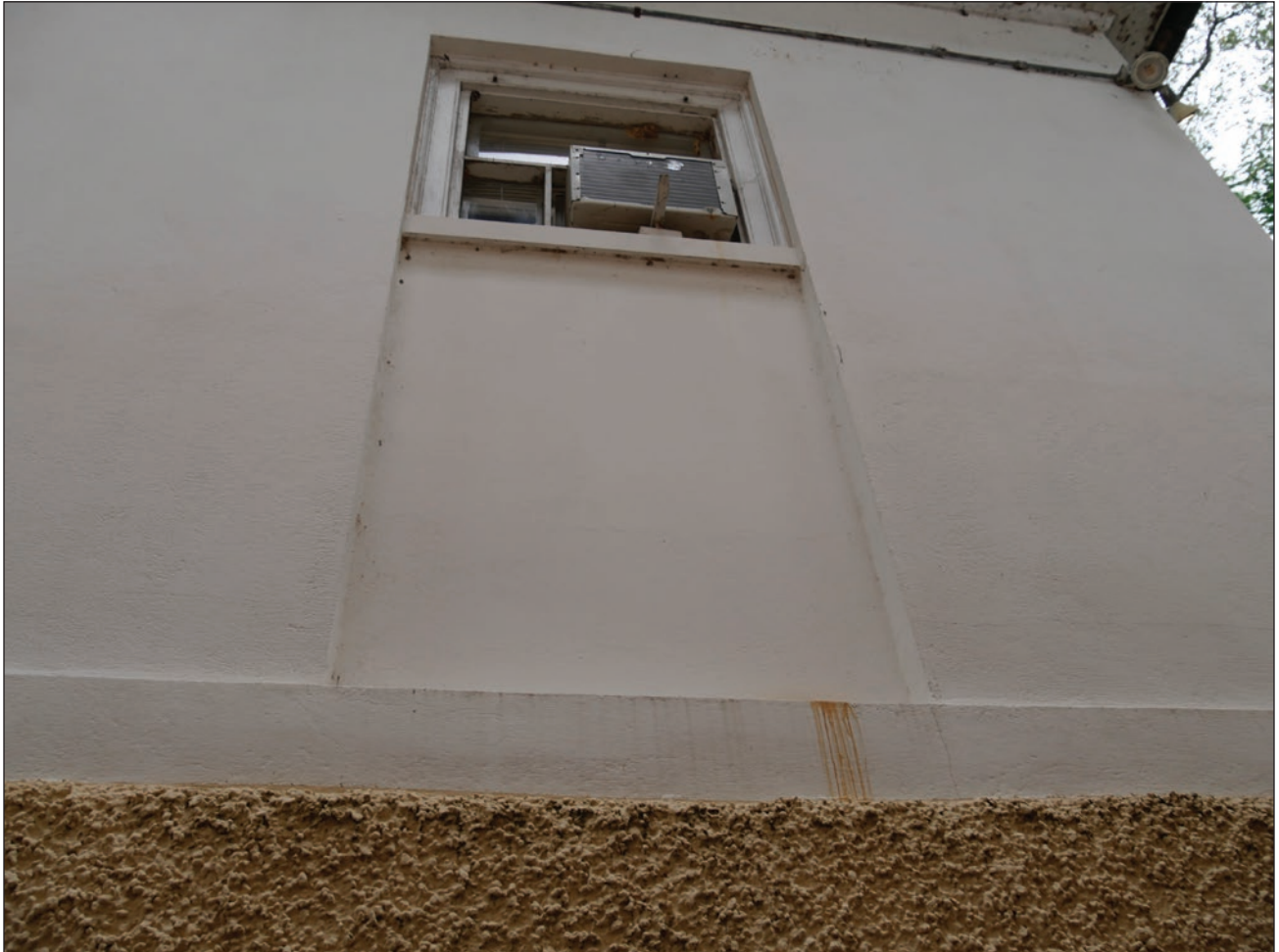
Figure 210. Rust staining on the flat stucco beneath a window A/C unit on the east elevation. Building Conservation Associates, 2025.
