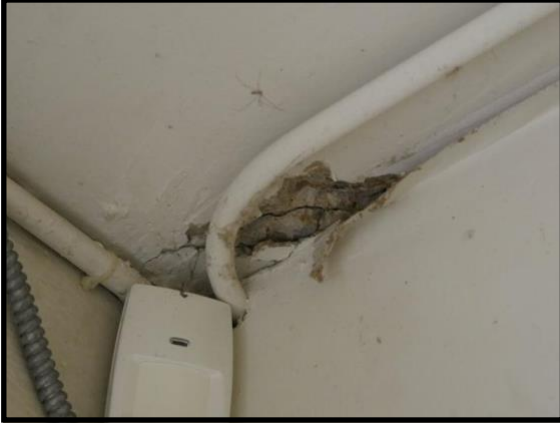
Photo P-23: First floor slab spall above north basement room
