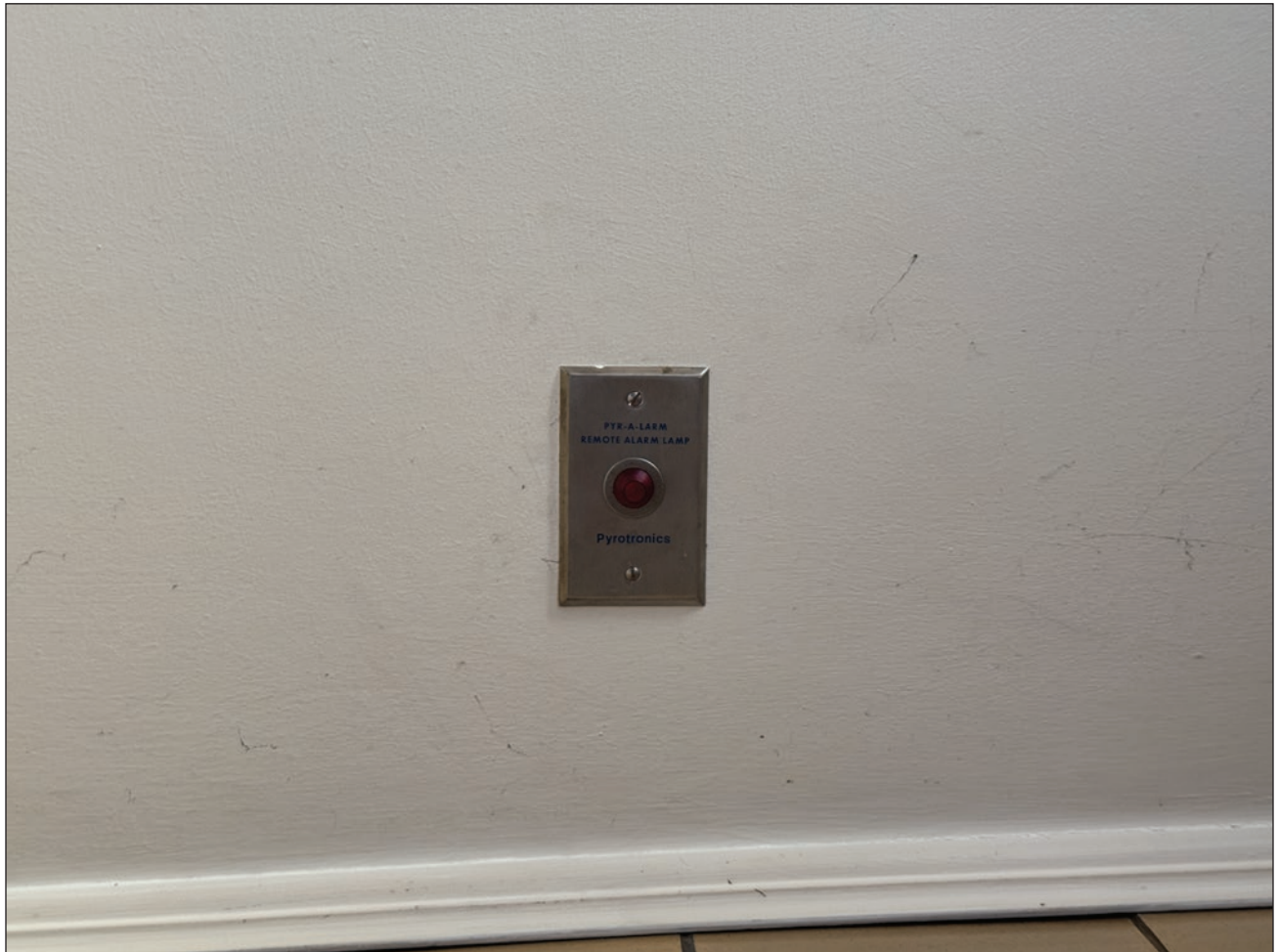
Figure 188. Pyrotechnics Pyr-a-larm in vestibule. Building Conservation Associates, 2025.
