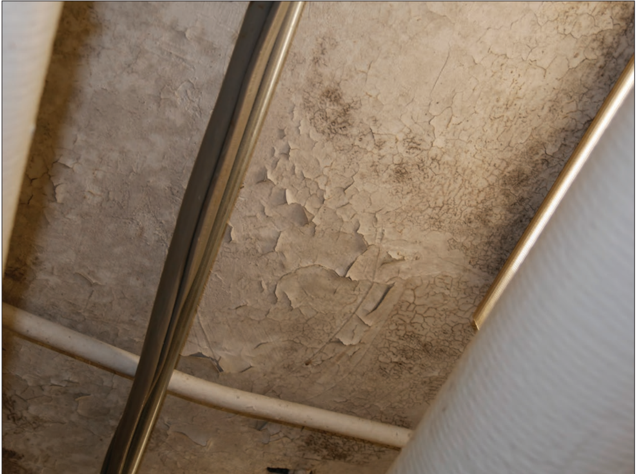
Figure 266. Flaking paint and mold at plaster ceiling in basement. Building Conservation Associates, 2025.
