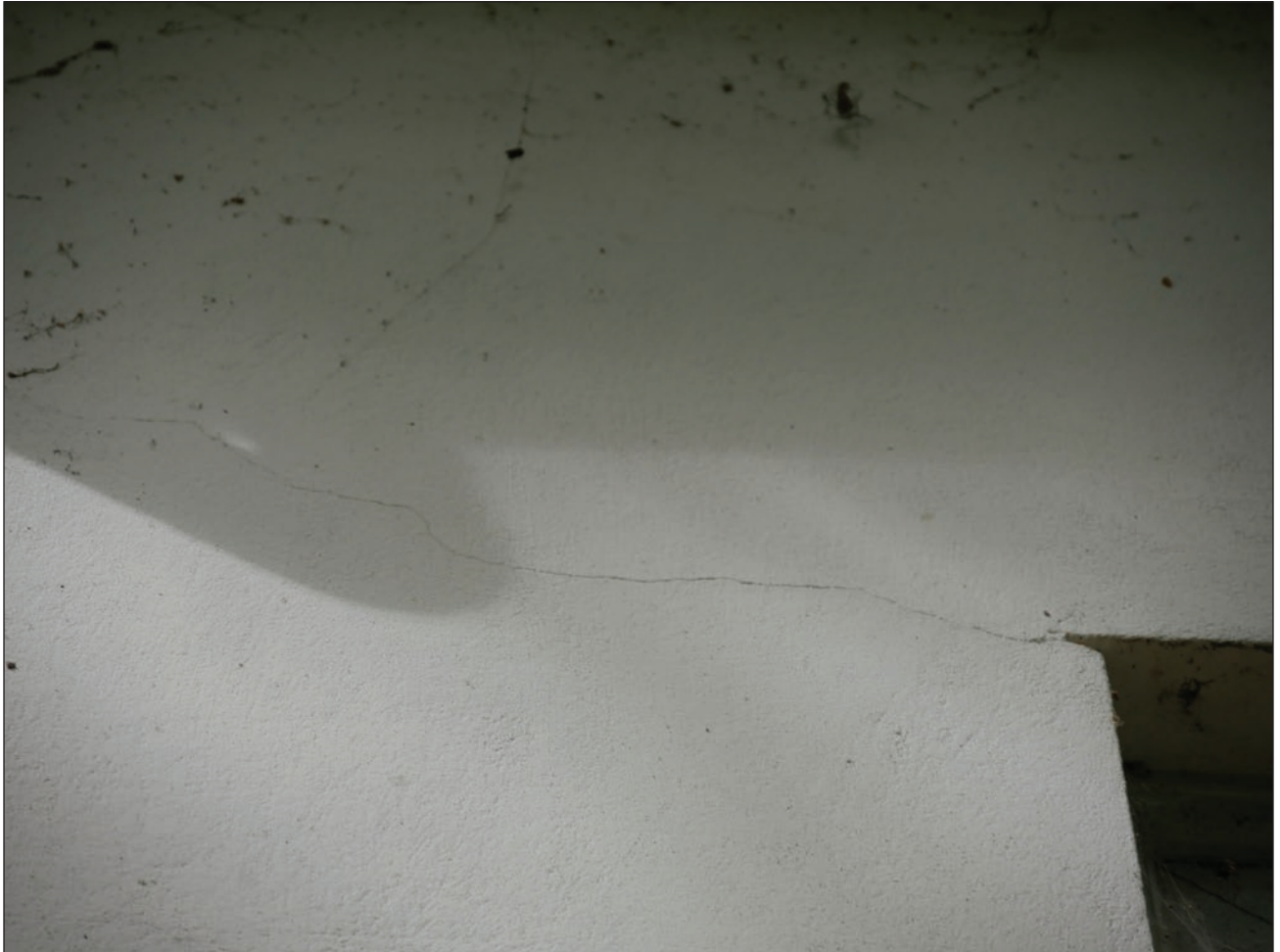
Figure 212. Narrow crack in the flat stucco on the east elevation. Building Conservation Associates, 2025.
