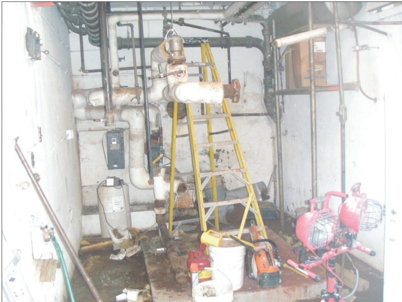
Figure 61. Mechanical equipment in the basement of the 1921 comfort station. ARHO Archives.
