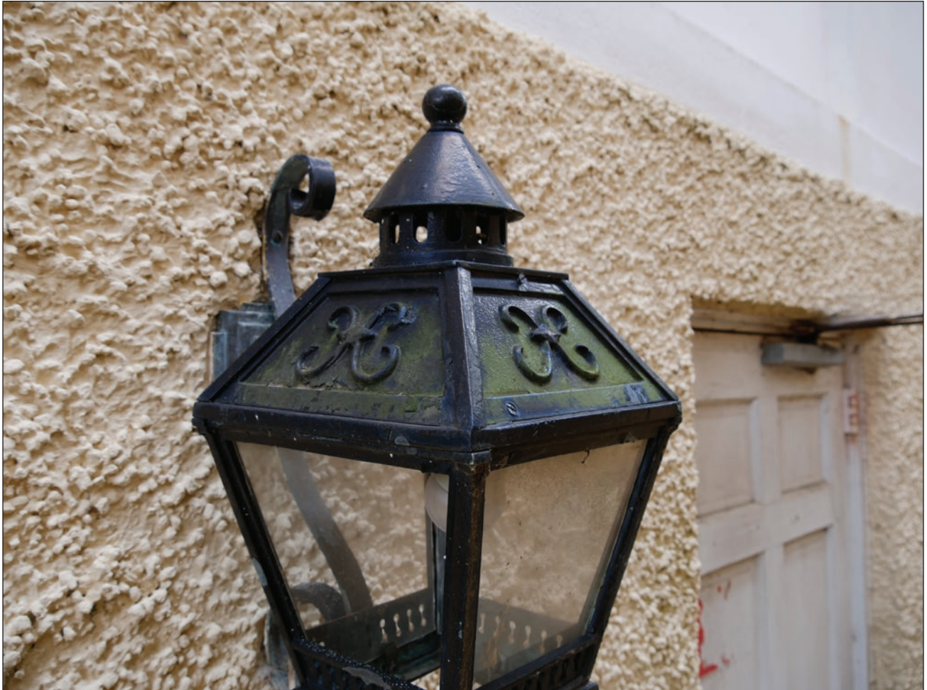
Figure 242. Biological growth on iron lantern sconce at south elevation. Building Conservation Associates, 2025.
