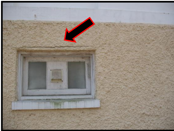
Photo P-19: Crack above window – north building elevation
