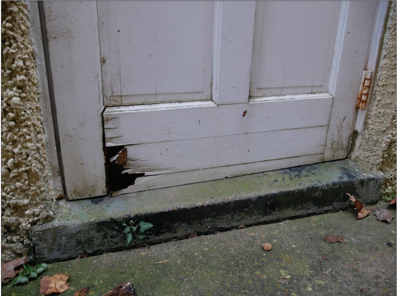
Figure 236. Damaged wood rail at southeast basement door. Building Conservation Associates, 2025.
