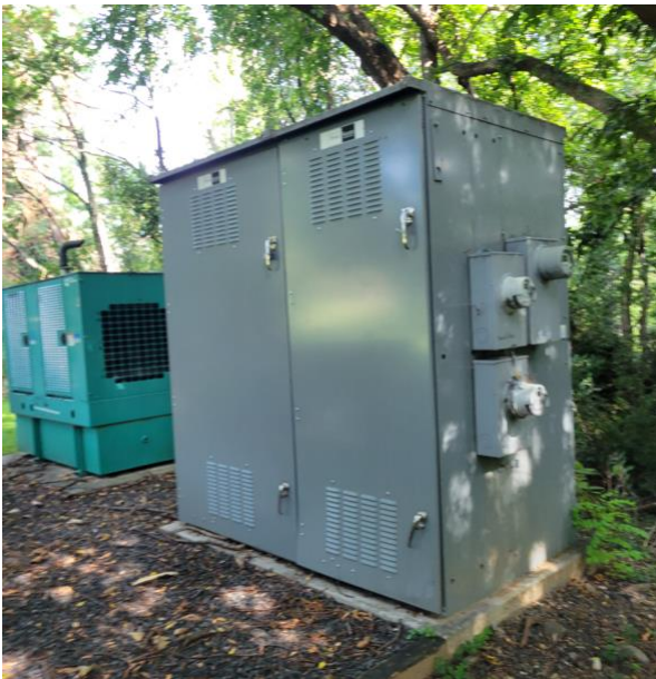
Photo E02: Generator and utility switchboard with attached electrical meters.
