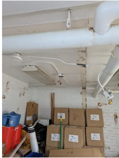
Photo M 016: Boiler Piping
