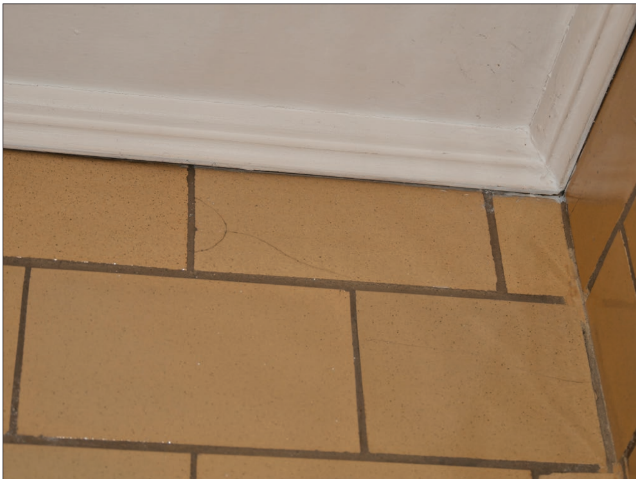
Figure 259. Crack in vestibule glazed tile wall. Building Conservation Associates, 2025.
