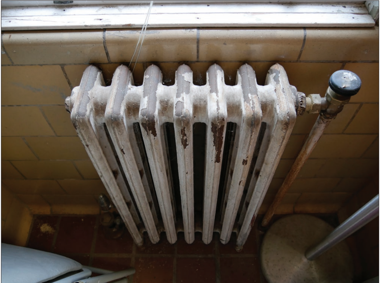
Figure 274. Paint loss at radiator in vestibule. Building Conservation Associates, 2025.
