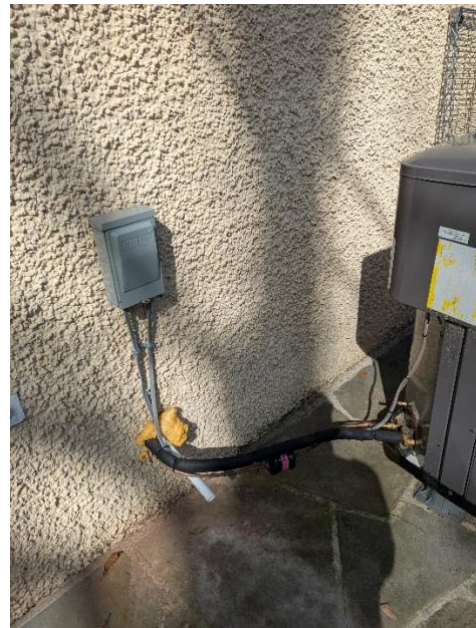
Photo M 002: Refrigerant Piping
