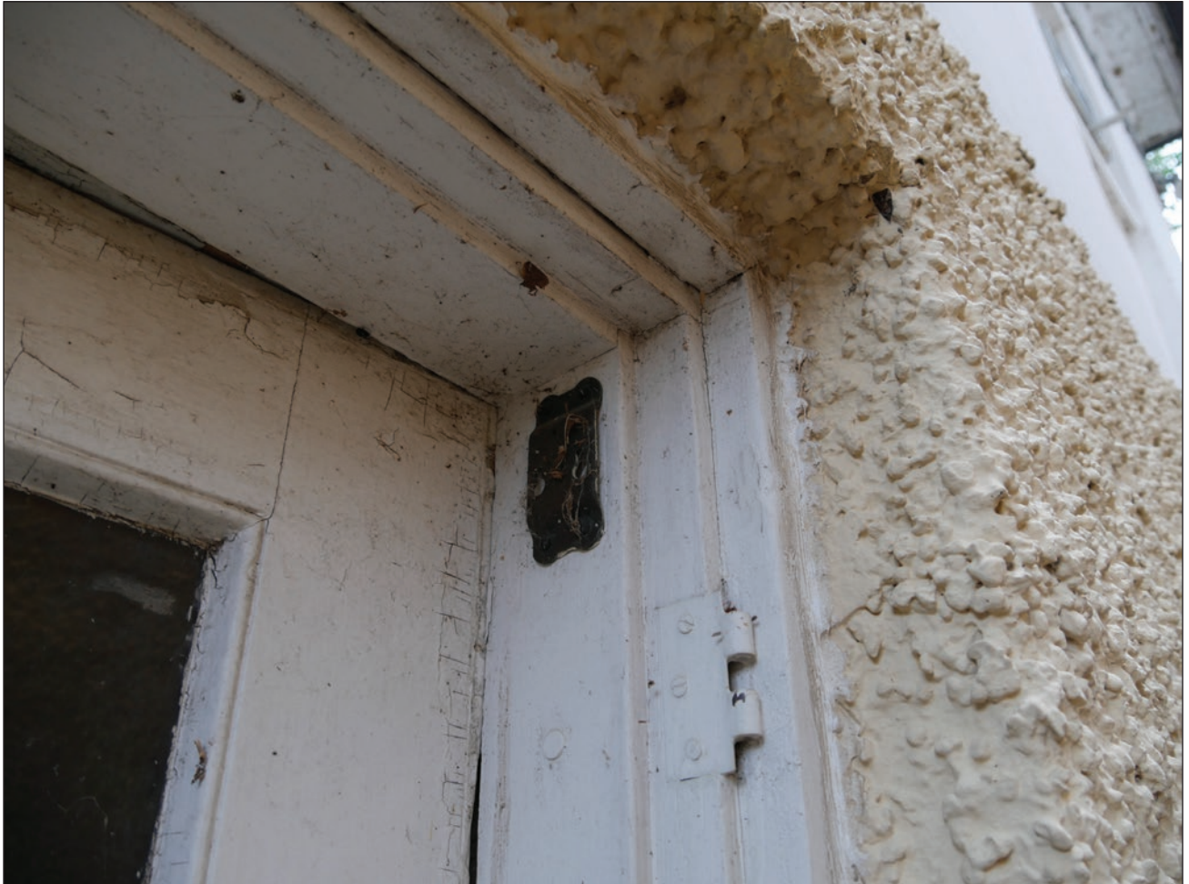
Figure 232. Abandoned historic and non-historic hardware at southwest basement door. Building Conservation Associates, 2025.
