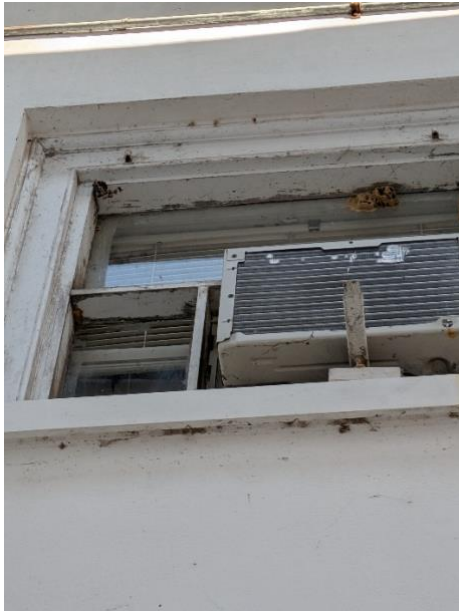
Photo M 009: Window AC Unit
