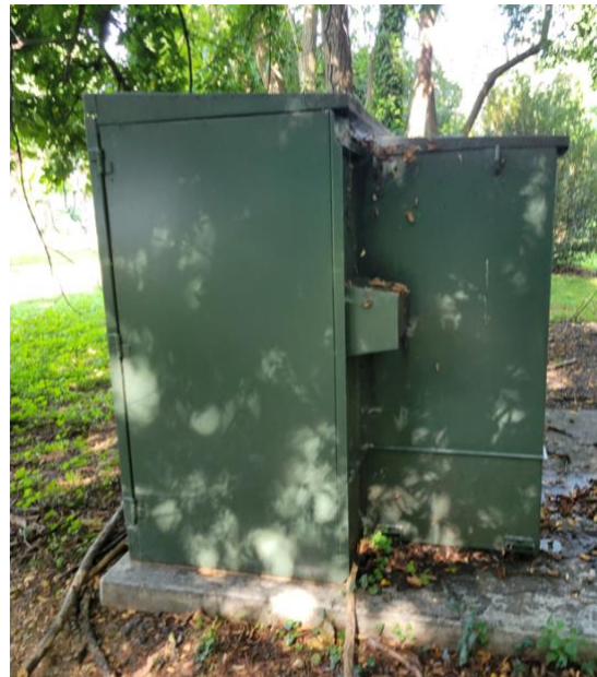
Photo E03: Dominion Energy pad-mounted transformer serving the building.
