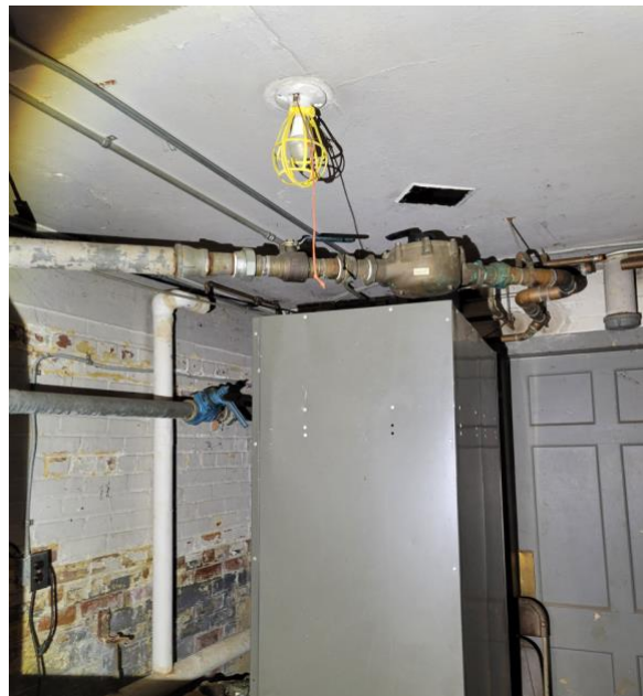
Photo E12: Mechanical room ceiling containing a single lamp-holder fixture.
