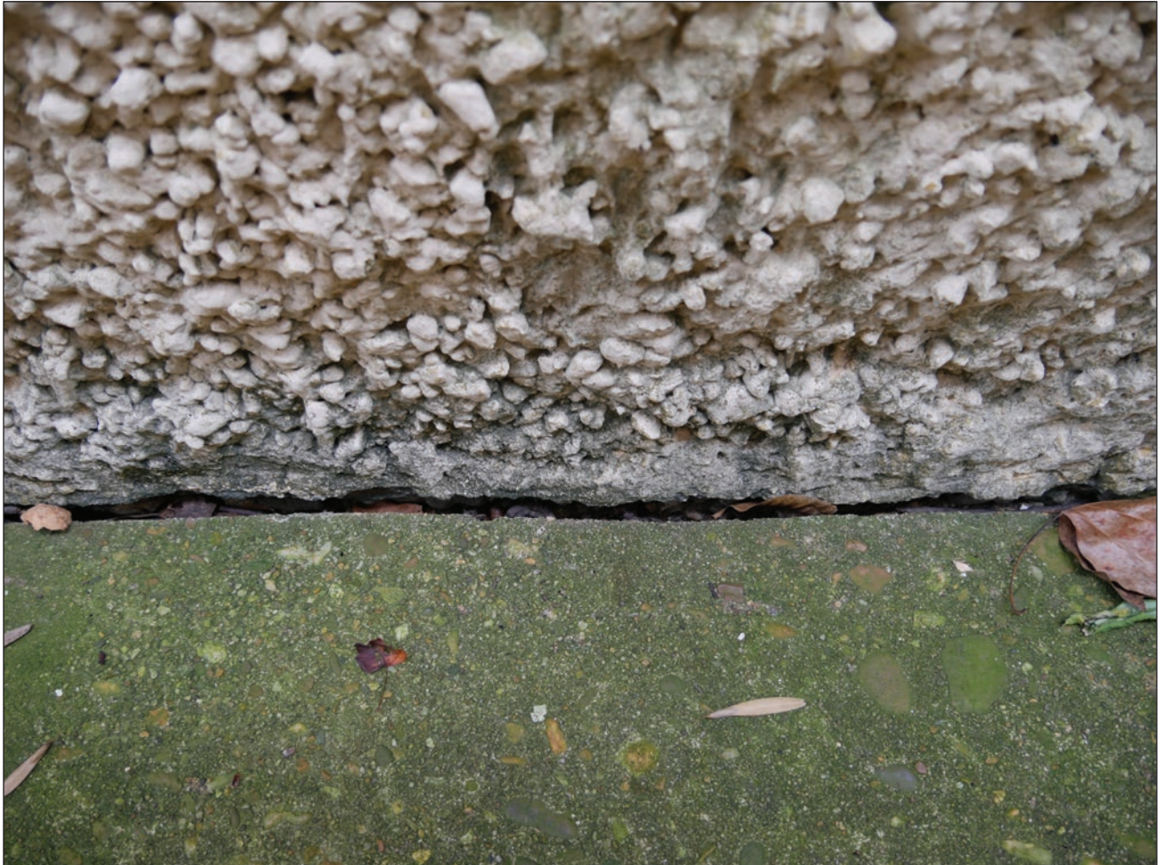
Figure 228. Sealant loss and stains from biological growth at concrete walkway on the south side of the building. Building Conservation Associates, 2025.
