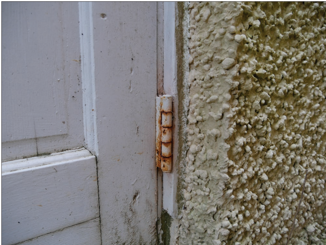
Figure 237. Rusting hinge at southeast basement door. Building Conservation Associates, 2025.
