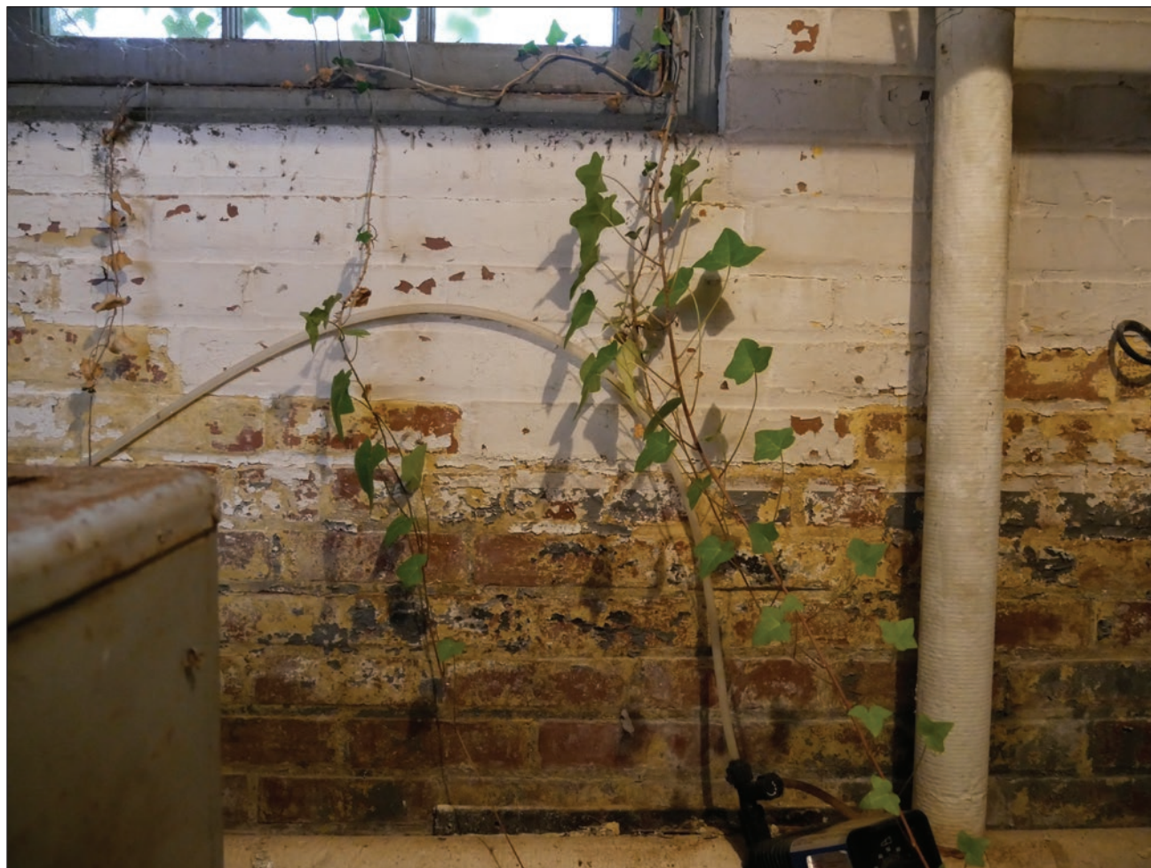
Figure 249. Water damage, mold, paint loss, and biological growth at southwest basement room. Building Conservation Associates, 2025.
