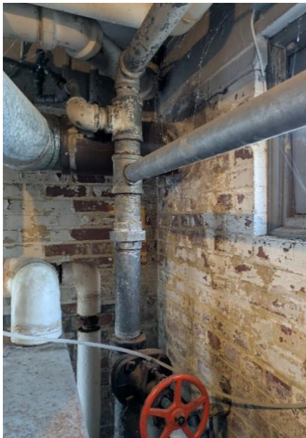
Photo P 001: Incoming Domestic Water Service
