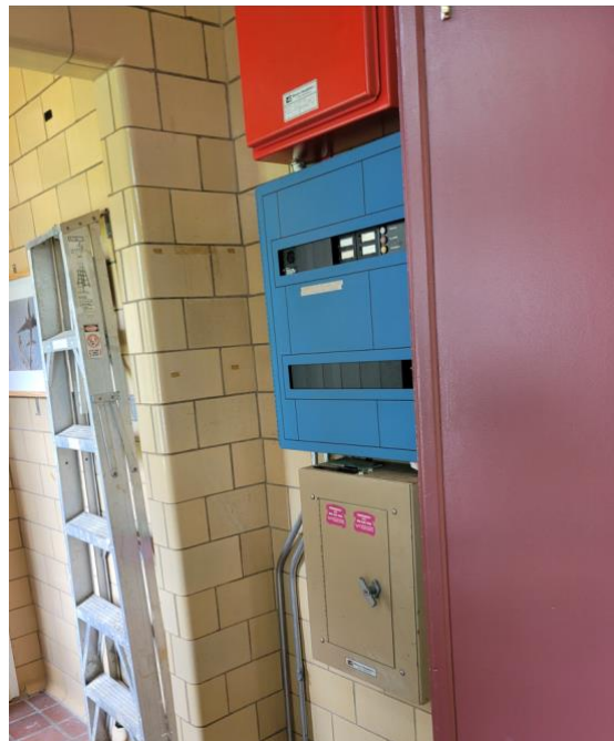
Photo E18: Vestibule wall with Monaco and Pyrotronics fire alarm cabinets.
