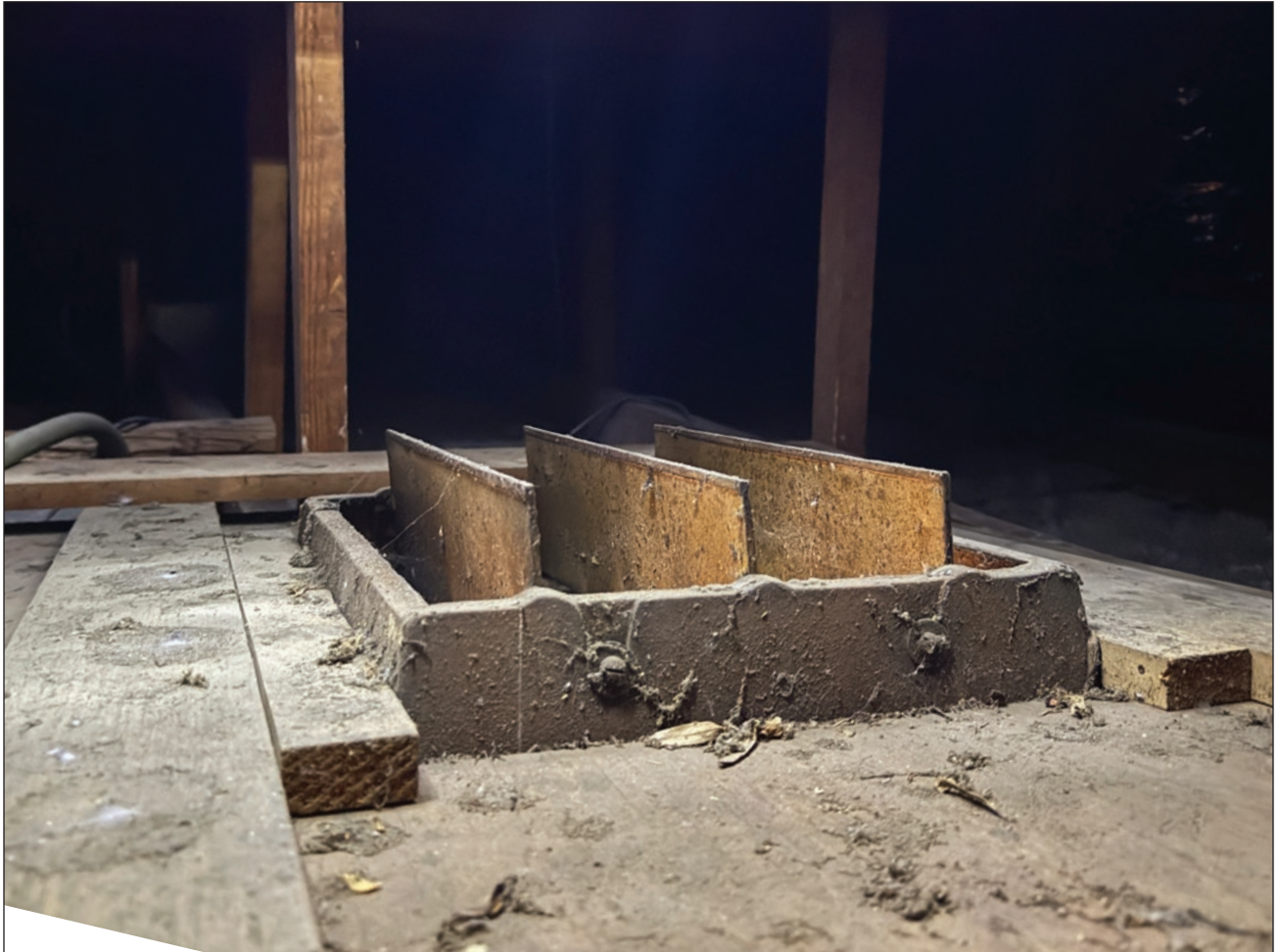
Figure 202. Cast iron vent dampers in the attic. Building Conservation Associates, 2025.
