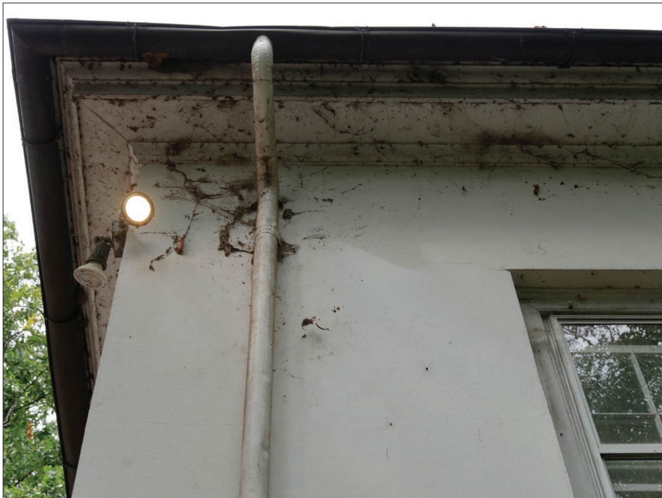
Figure 213. Insect activity at the cornice of the southeast corner. Building Conservation Associates, 2025.
