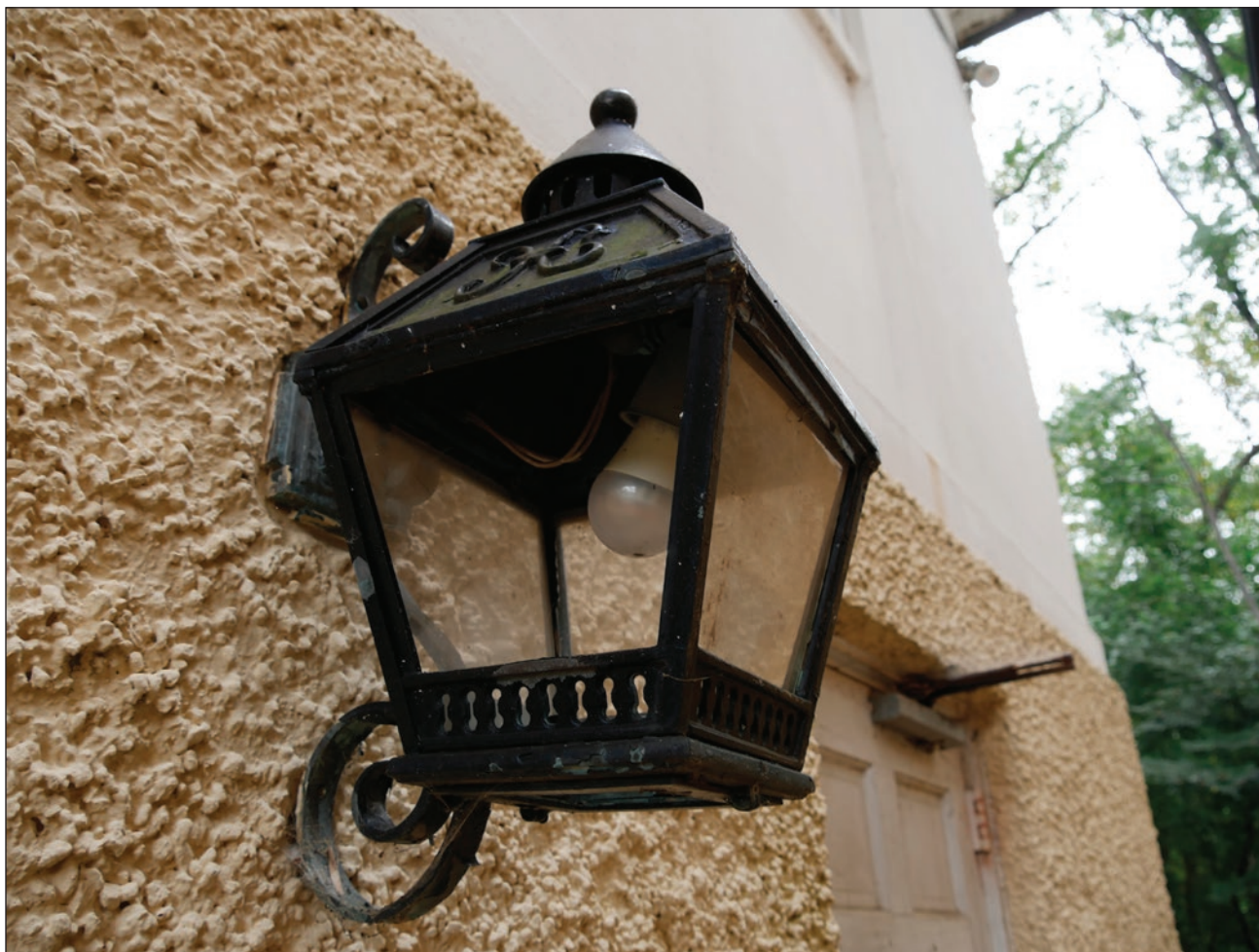
Figure 243. Missing glass pane at lantern sconce at south elevation. Building Conservation Associates, 2025.
