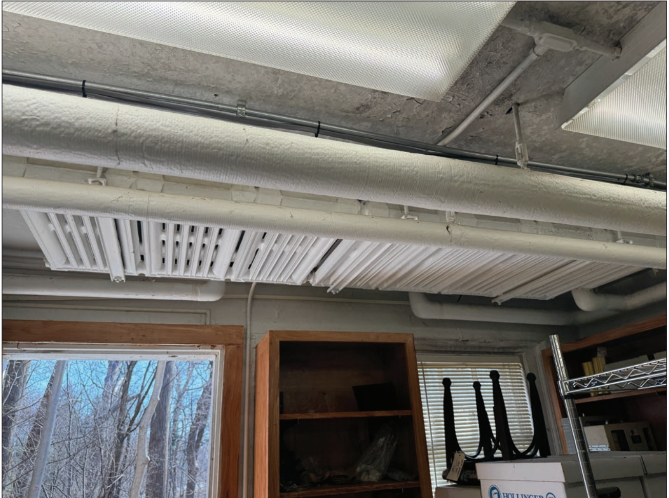
Figure 173. Overhead radiator in the center basement room. Building Conservation Associates, 2025.
