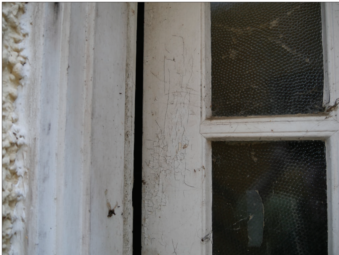
Figure 229. Paint flaking at southwest basement door. Building Conservation Associates, 2025.
