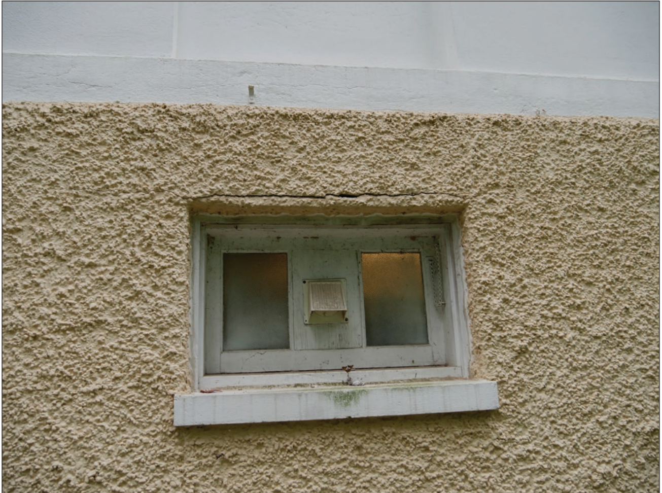
Figure 206. Horizontal crack in the pebble dash stucco at the lintel above a basement window on the north elevation. Also note the modification of the hopper window to accommodate a vent. Building Conservation Associates, 2025.
