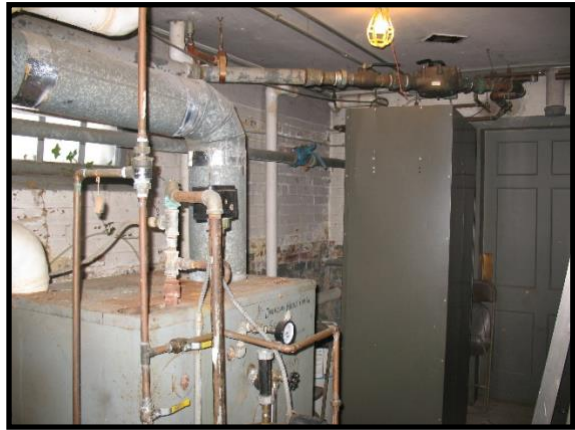
Photo P-12: Basement mechanical room looking northwest
