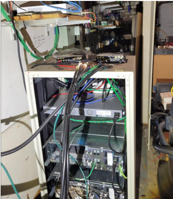
Photo E21: Data rack containing network cables and electronic components.
