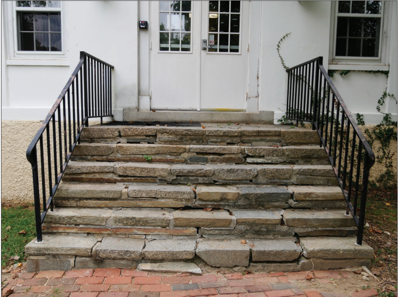
Figure 244. Displaced stones and mortar loss at main entry steps. Building Conservation Associates, 2025.
