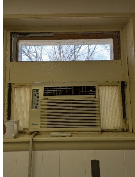
Photo M 008: Window AC Unit
