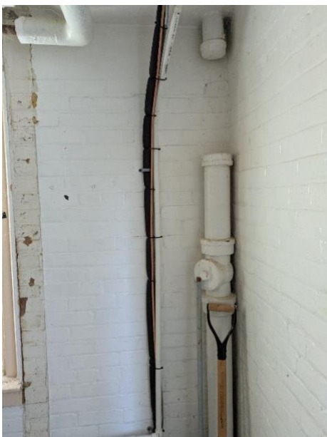
Photo P 005: Abandoned Sanitary Stack
