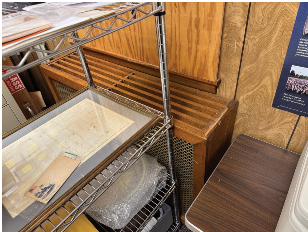
Figure 193. Radiator covered with a wood and metal mesh enclosure. Building Conservation Associates, 2025.
