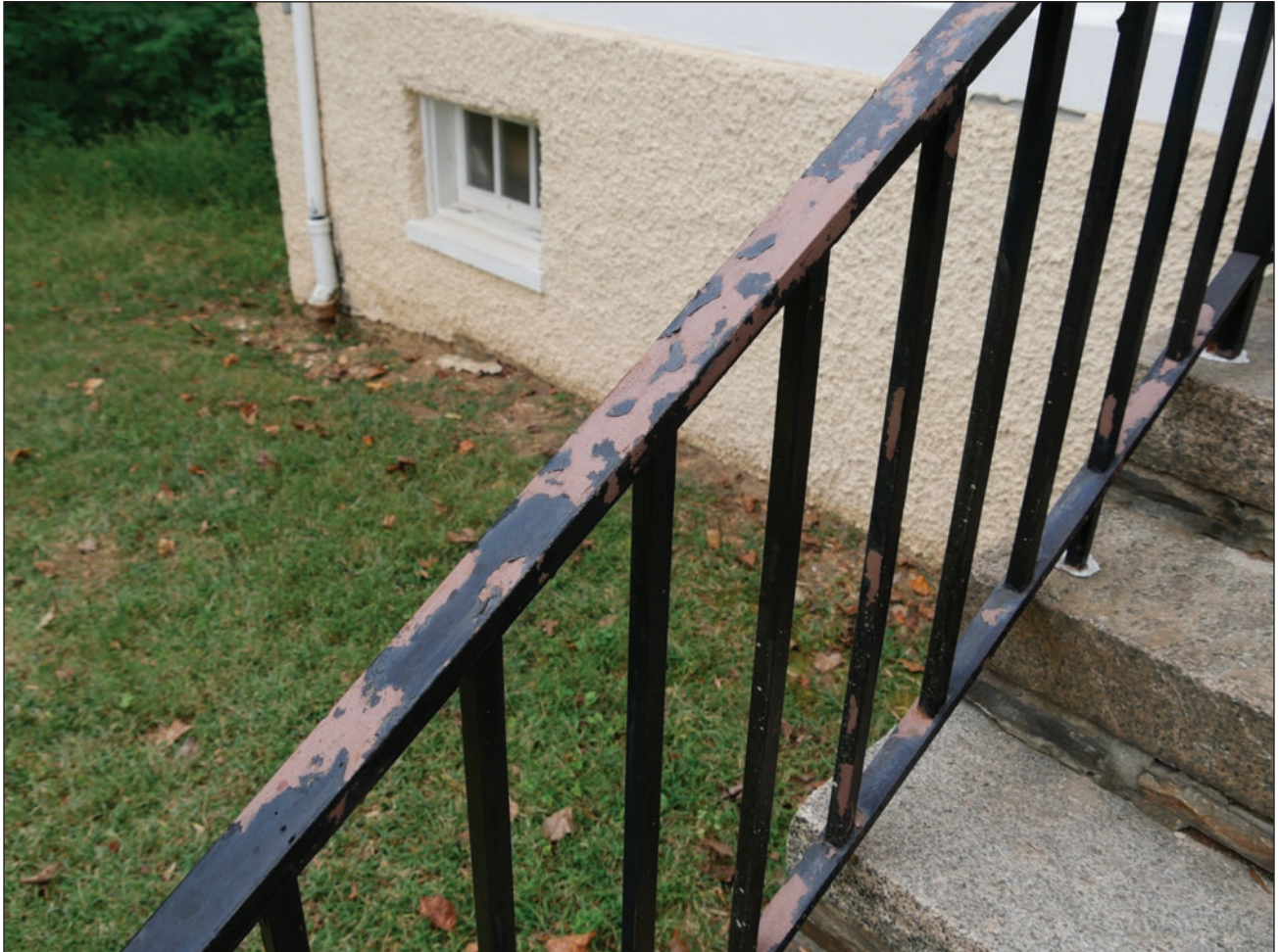
Figure 248. Paint loss and rust at wrought-iron handrail at main entry steps. Building Conservation Associates, 2025.
