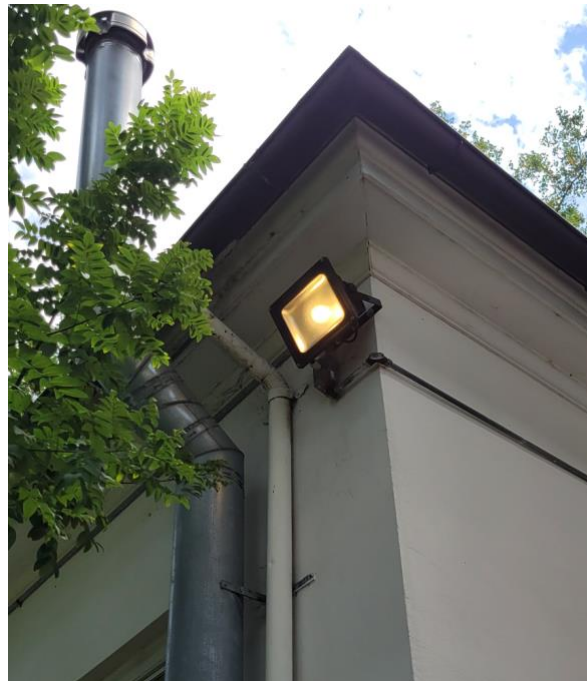
Photo E26: Exterior HID floodlights operating during daytime hours.
