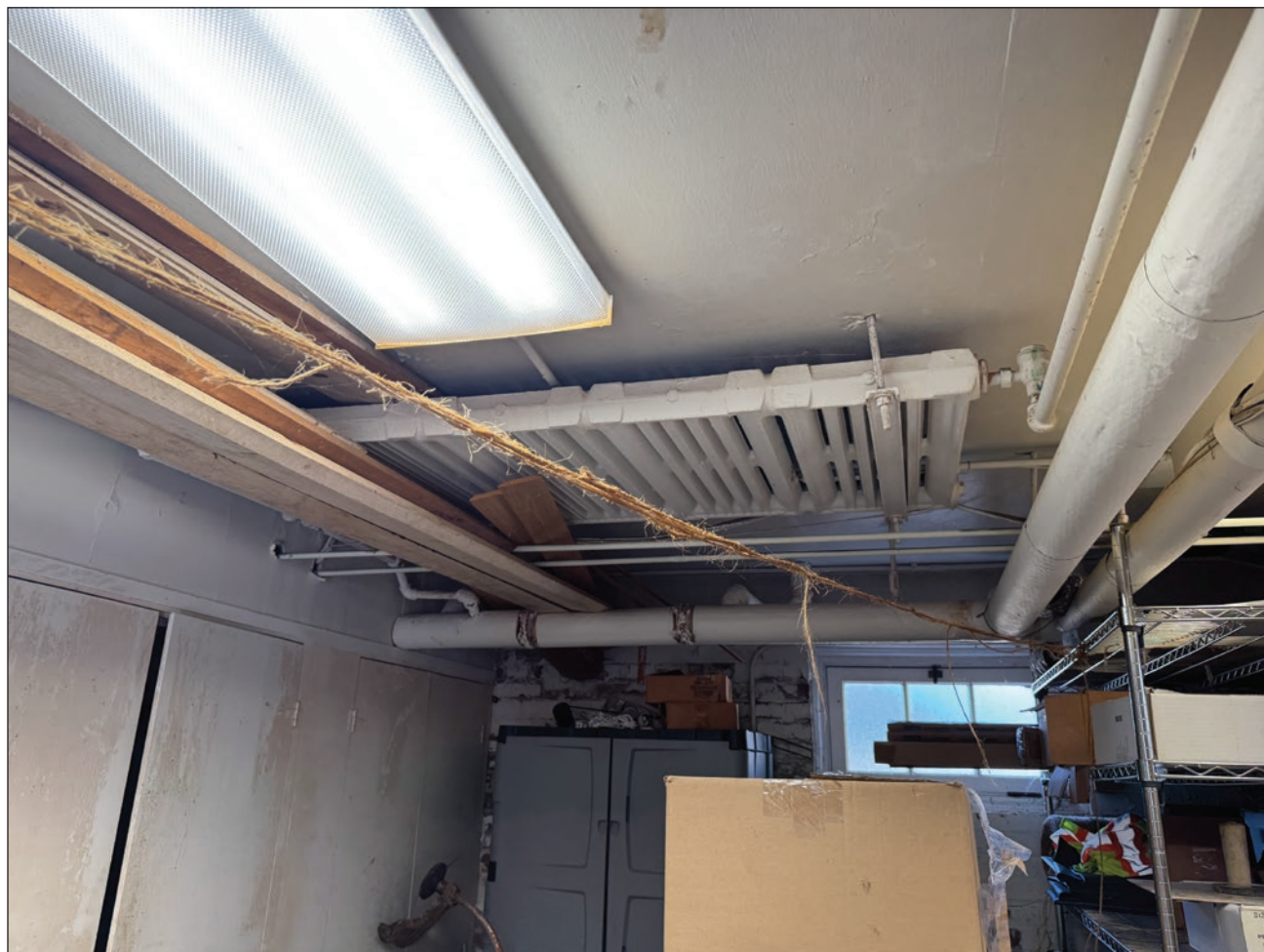
Figure 176. Overhead radiator in the north basement room. Building Conservation Associates, 2025.
