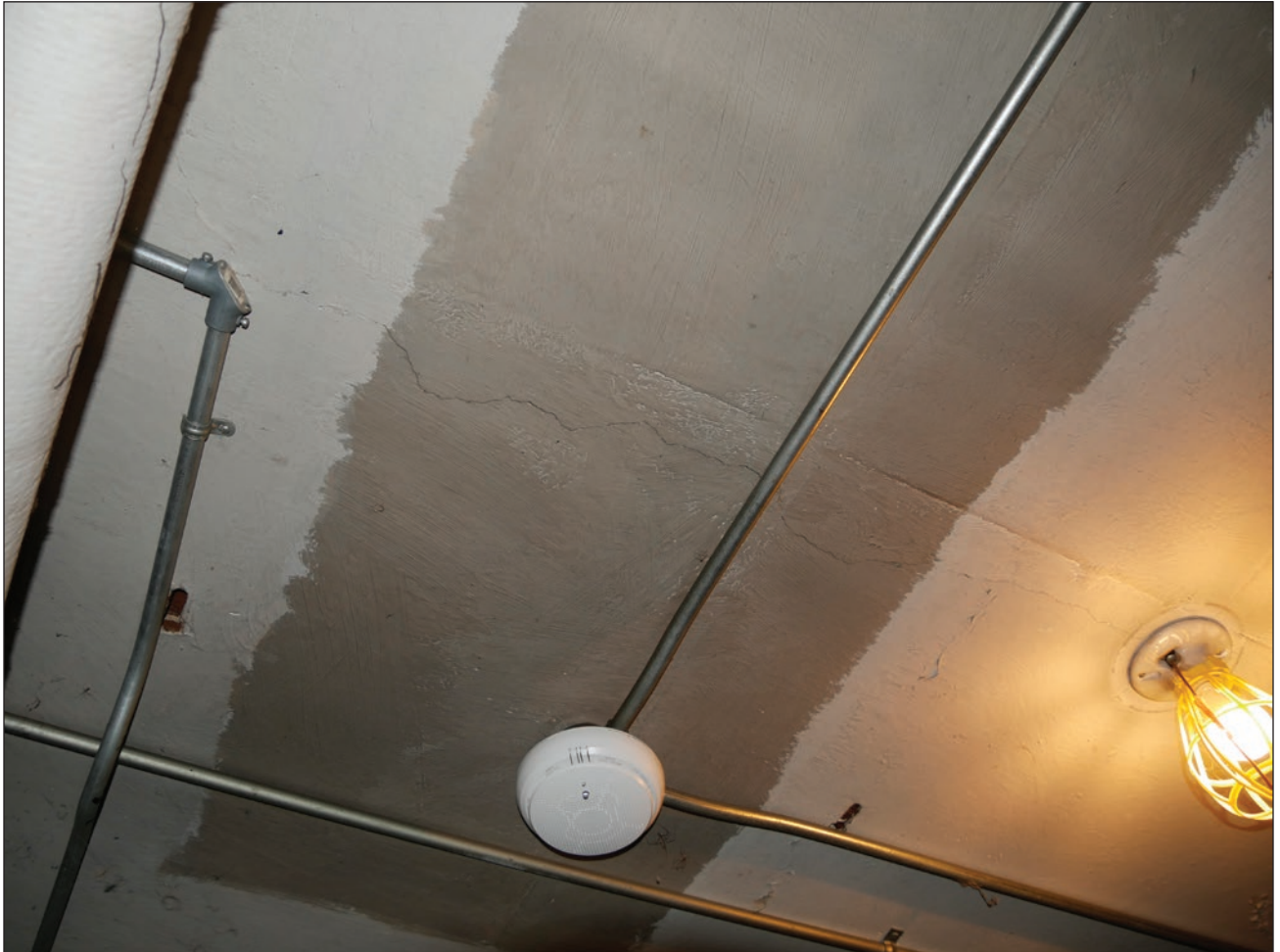
Figure 264. Cracks and penetrations in plaster ceiling in basement. Building Conservation Associates, 2025.
