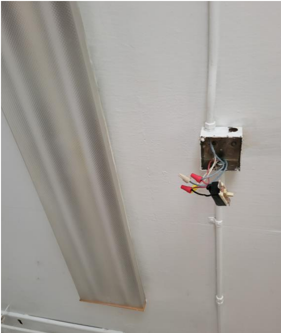
Photo E06: Storage room wall with exposed junction box and toggle switch.
