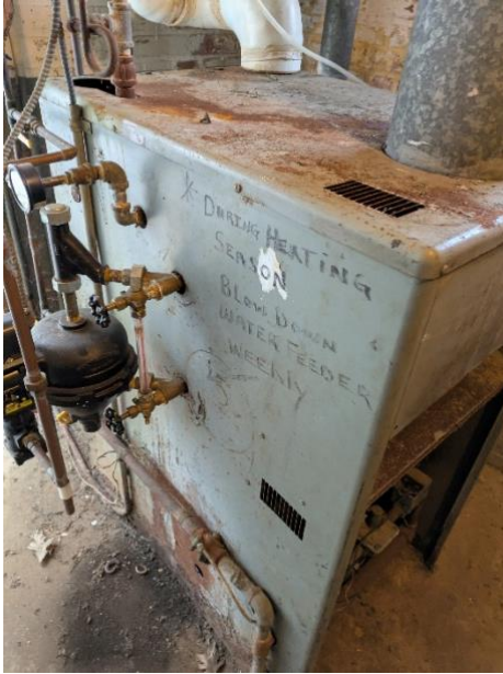
Photo M 011: Boiler
