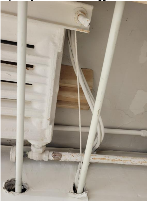
Photo E08: Painted non-metallic conductors along wall surface.
