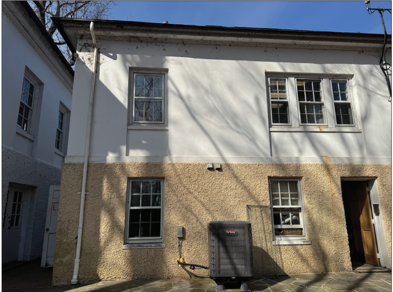
Figure 163. Air conditioning unit at east side of building. Building Conservation Associates, 2025.
