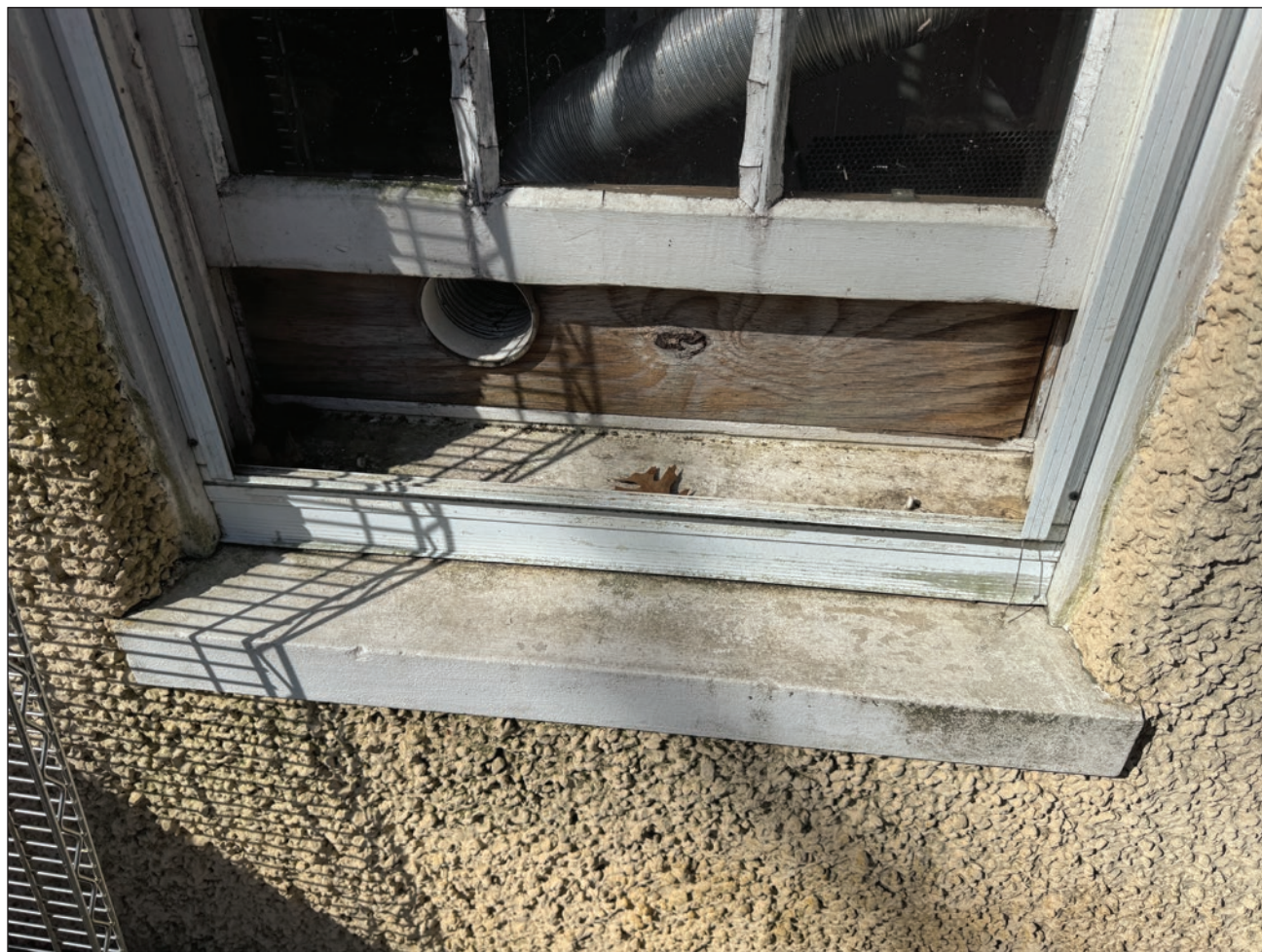
Figure 217. Failing sealant and paint at a sash window on the east elevation. Building Conservation Associates, 2025.
