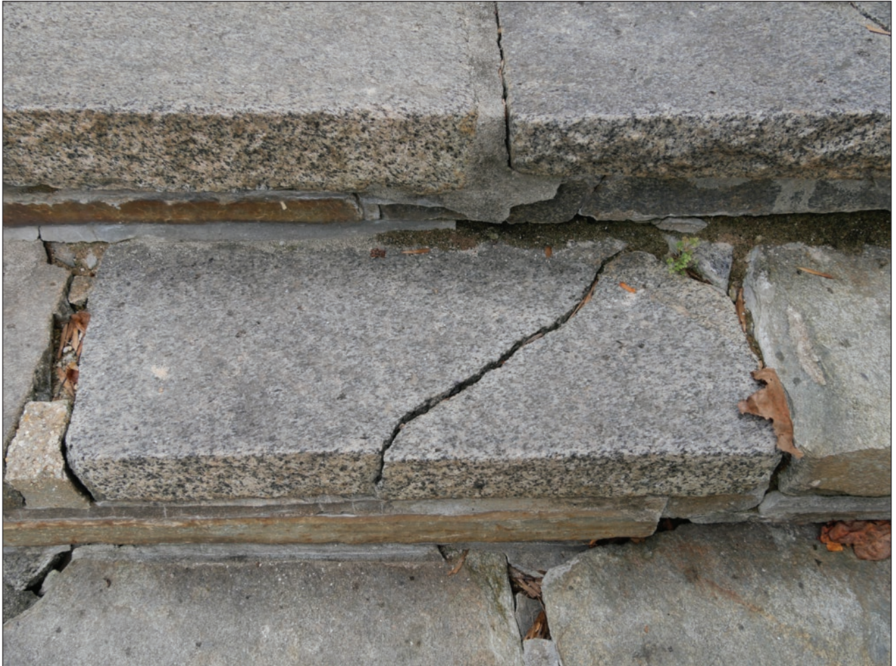
Figure 246. Cracked stone unit at main entry steps. Building Conservation Associates, 2025.
