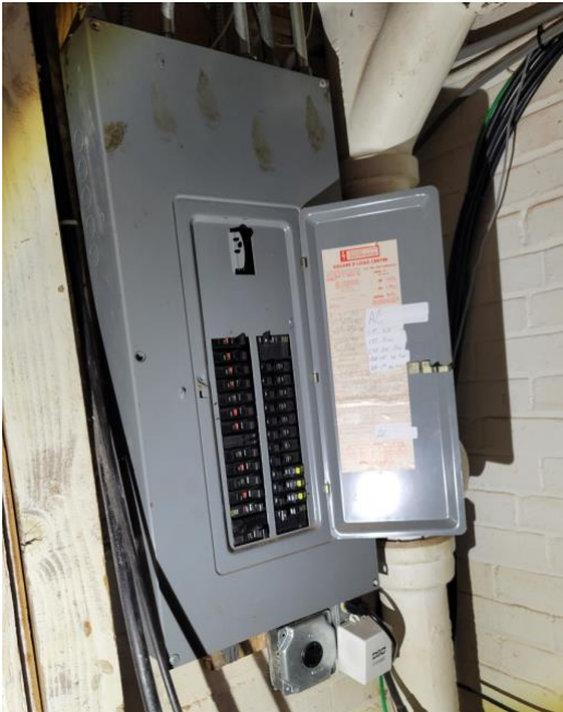
Photo E04: Interior equipment closet showing Square D 200-amp load center.
