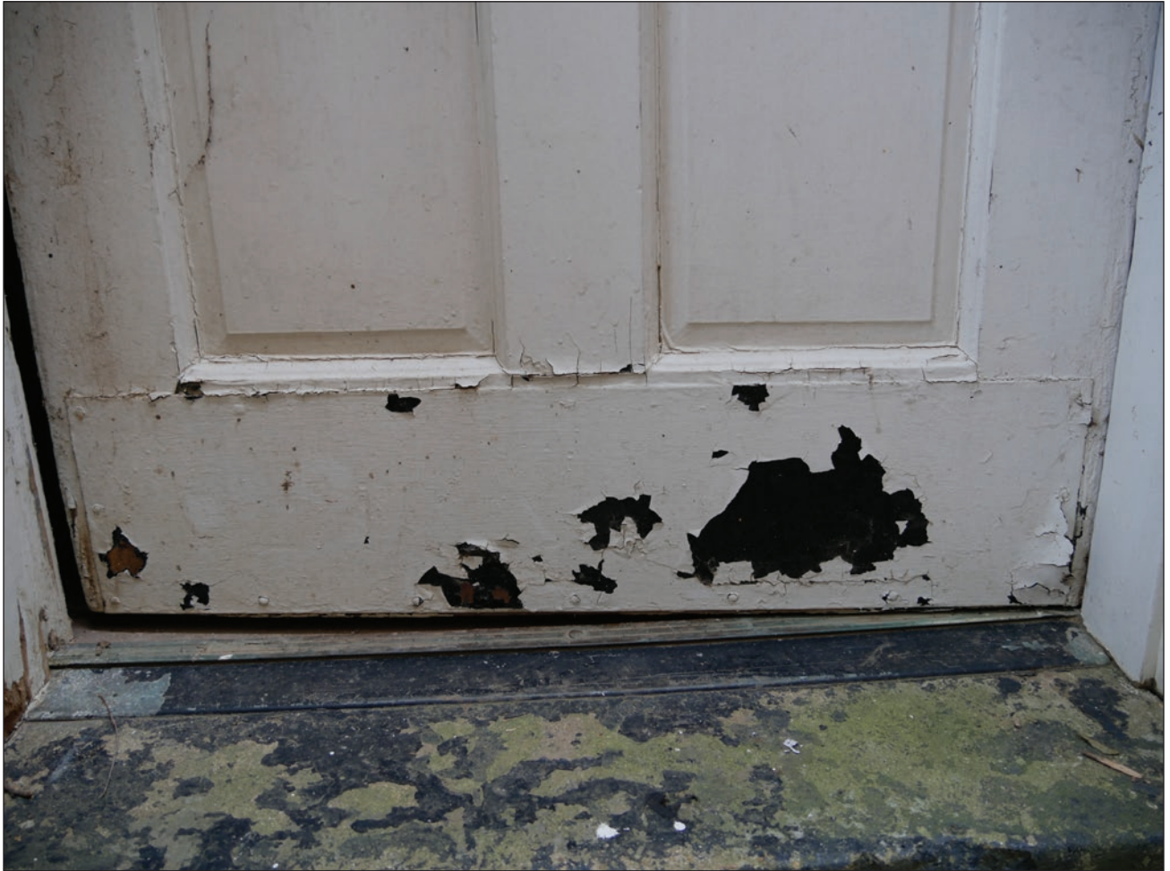
Figure 230. Paint loss and stains from biological growth at southwest basement door and threshold. Building Conservation Associates, 2025.
