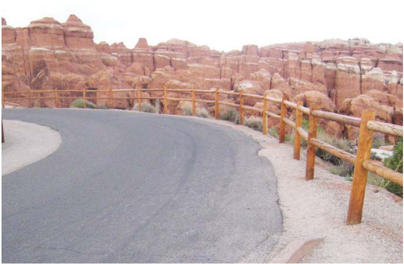
7 Asphalt edge showing damage
