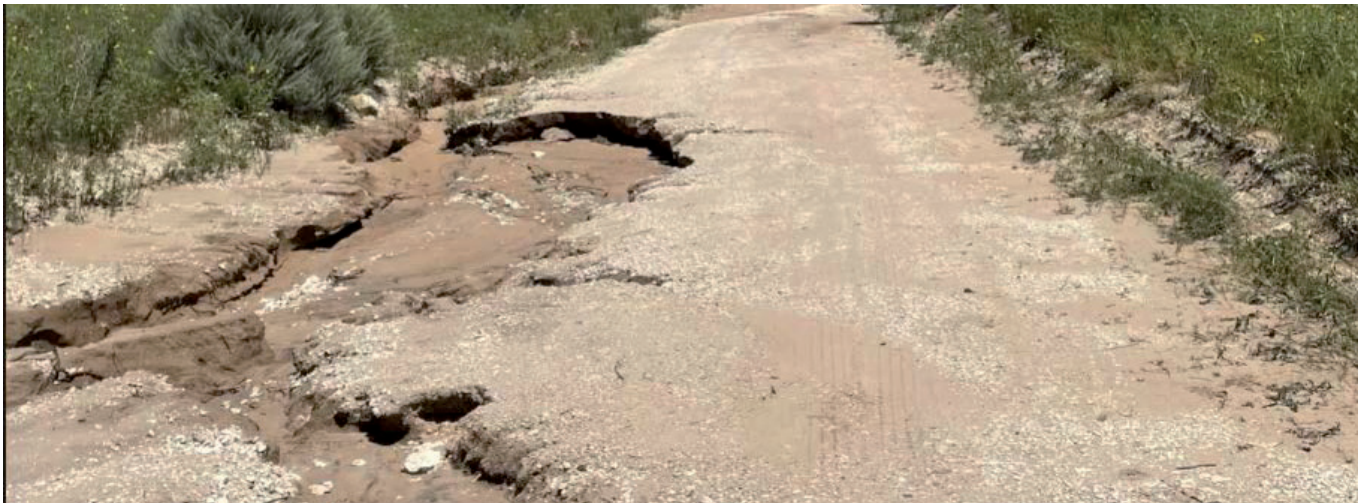
Road damage from last year's heavy rains.
