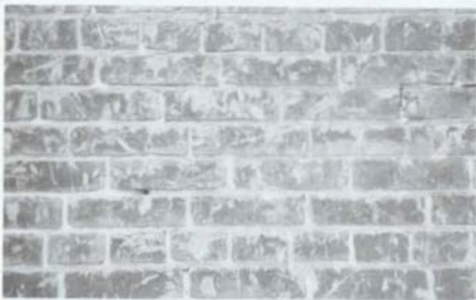
Figure 45. M'Clintock House: Damaged Bricks at Former East-Wall Trellis [1988].
