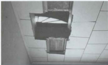
Figure 109. M'Clintock House: Room 203 (Southeast Bedroom), Ceiling at Attic Hatch [1988].
