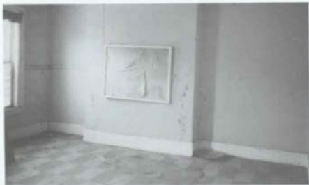
Figure 104. M'Clintock House: Room 202 (Northeast Bedroom), East Wall, Showing Chimney Breast Lacking Fireplace Mantel [1988].
