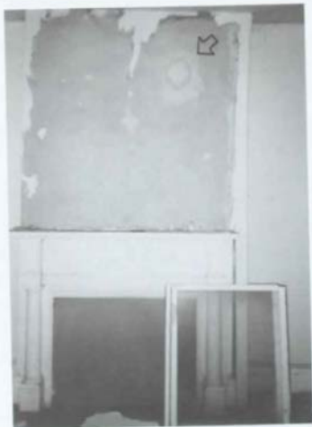
Figure 77. M'Clintock House: Room 102 (Parlor), Patch in Chimney Breast at Former Stovepipe Hole [1988].
