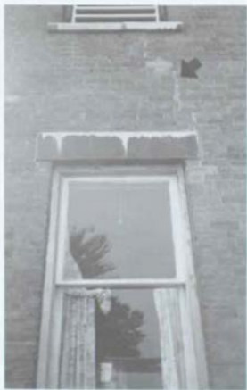
Figure 46. M'Clintock House: Vertical Crack Between Windows in the East Wall [1988].
