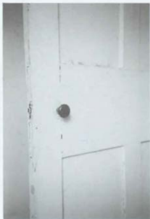
Figure 105. M'Clintock House: Room 202 (Northeast Bedroom), South Wall, Original Doorknob on East Door [1988].
