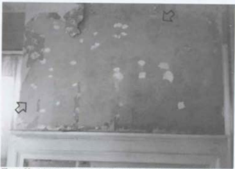
Figure 92. M'Clintock House: Room 104 (Kitchen/Dining Room), Chimney Breast; arrows indicate stovepipe patch and wallpaper note shown below [1988].
