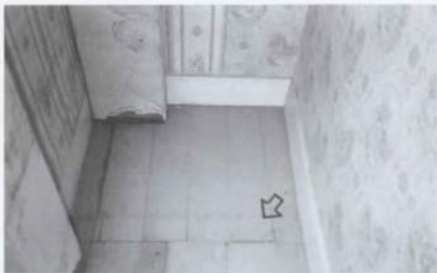
Figure 87. M'Clintock House: Room 103 (Southeast Room), Closet Floor at West End, Showing Location of Earlier Wall [1988].
