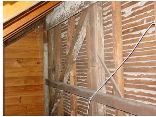
Figure 19: View of attic wall, west of Room 201. Note early siding board at top of photograph penetrated by circa 1880s rafters. (Photo by author.)
