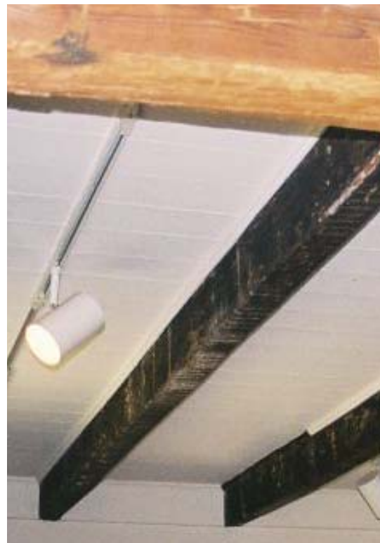
Figure 61: Exposed joists and beams at east end of Room 101. Note the ogee molding along the top. (Photo by author.)
