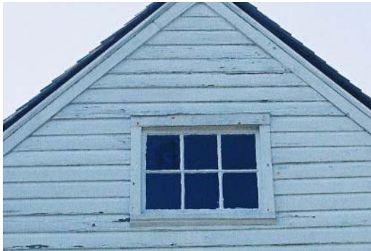
Figure 52: Window 16, fixed 6-light window at north end of attic. (Photo by author.)
