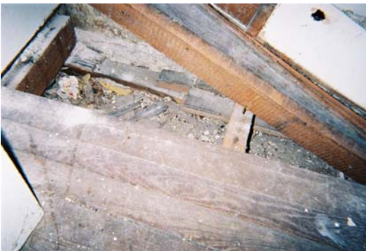
Figure 17: Floorboards and exposed joists over sand/shell grade in Room 103. (Photo by author.)
