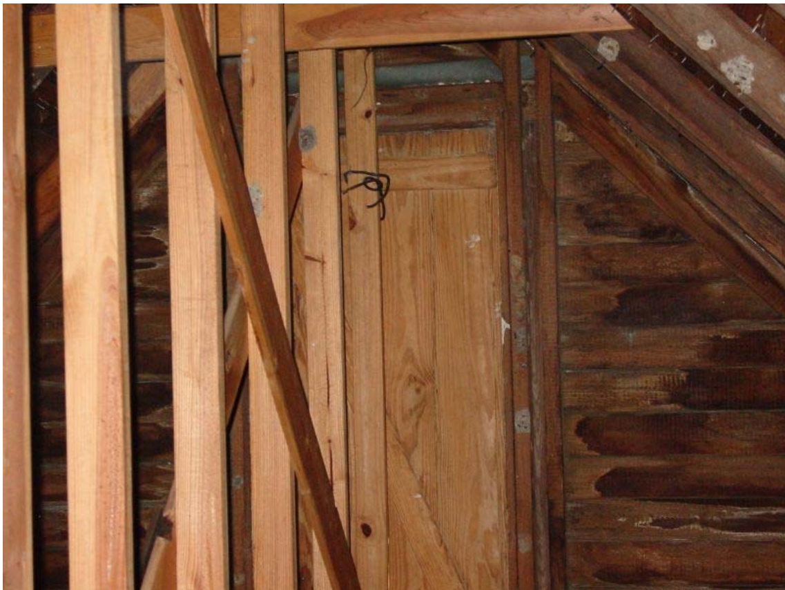
Figure 27: Load-bearing wall and roof framing at southern end of attic, above Room 203. Note Door 16 centered on wall. (Photo by author.)
