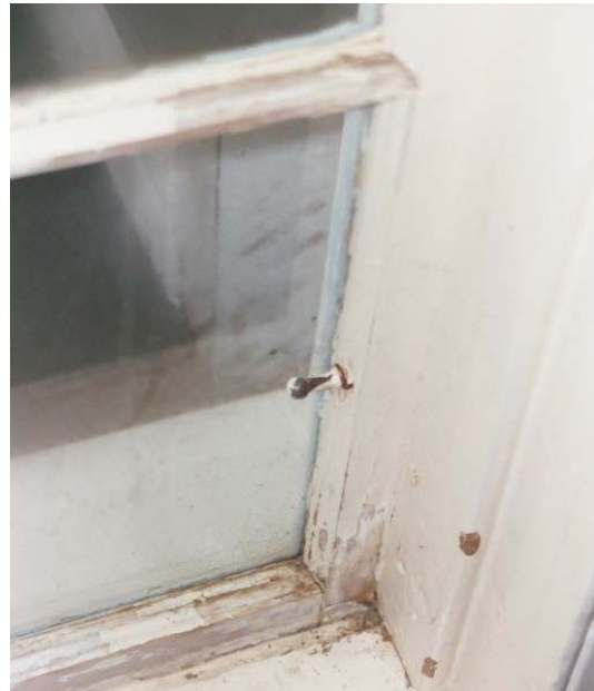
Figure 55: Typical window muntin. Note 20 th century sash lift. (Photo by author.)
