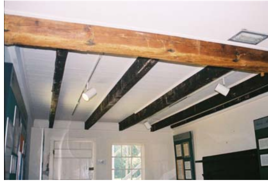
Figure 21: Floor joists of second floor exposed to east end of Room 101. (Photo by author.)
