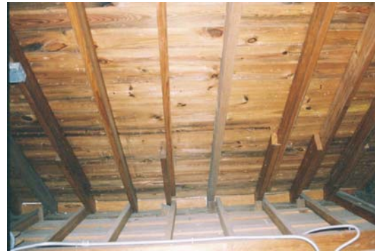
Figure 25: Attic space west of Room 201. Note the ceiling joists of the west end of Room 101. (Photo by author.)
