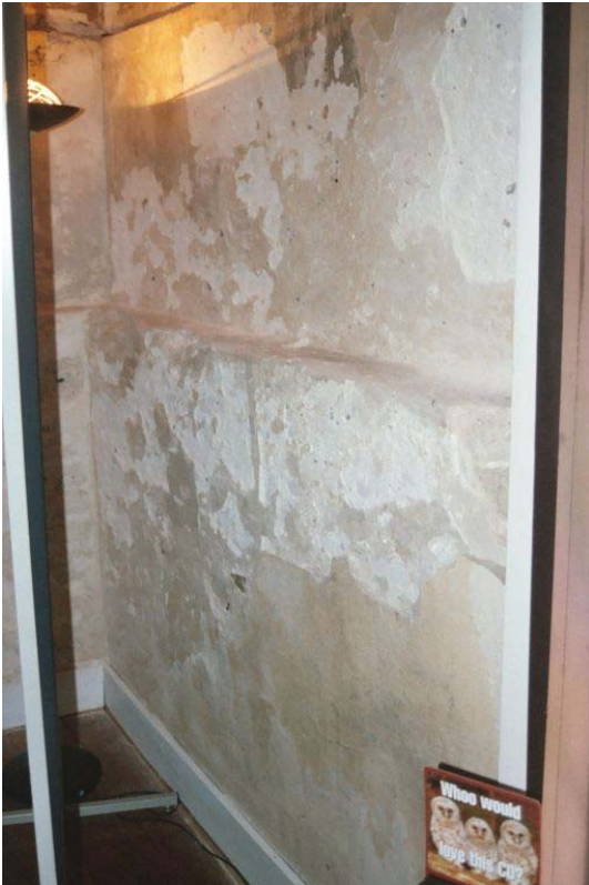
Figure 18: Detail of tabby wall of Room 104, looking southeast. Note the ledge formed by the earlier tabby brick portion of the wall. (Photo by author.)
