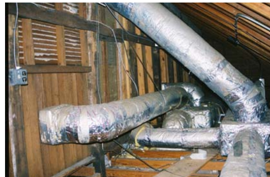
Figure 79: Southern view of attic space, west of Rooms 201, 202, and 203. Note the plaster keys in the left side of the photo and the gypsum board in the center. (Photo by author.)
