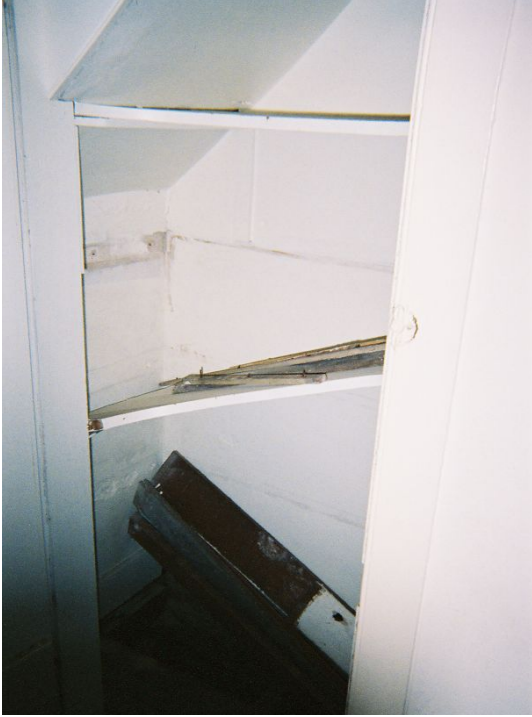
Figure 64: Room 103. Note slant in ceiling where exterior stairs penetrate the building. (Photo by author.)
