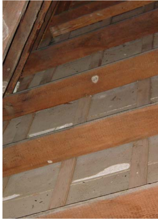
Figure 24: Ceiling joist of Room 201 exposed to east attic space. (Photo by author.)
