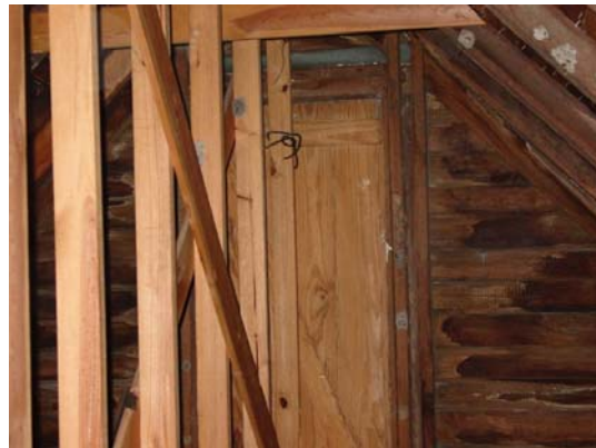
Figure 80: Southern view of attic space above Rooms 201, 202 and 203. Note the board and batten door in the center of the gable. (Photo by author.)
