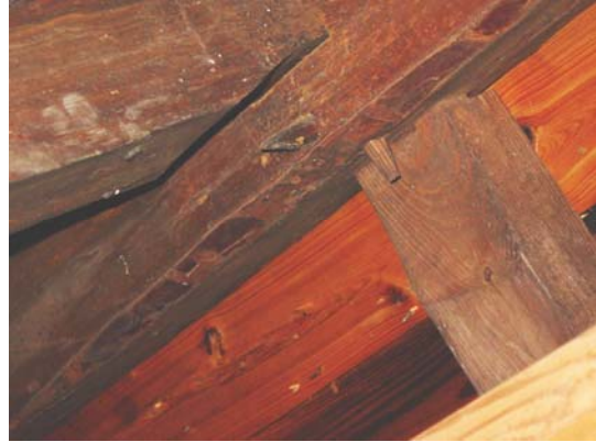
Figure 26: Hewn ridge beam in eastern attic. Note pegged connections. (Photo by author.)
