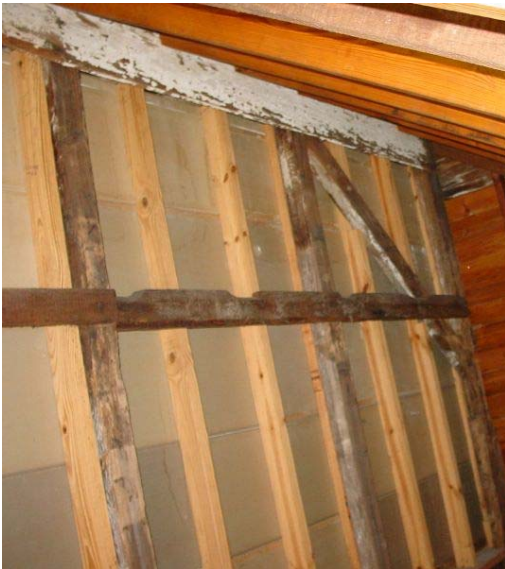
Figure 20: View of attic wall, west of Room 203. Note early siding board at top of photograph penetrated by circa 1880s rafters and notched beam below, possibly an earlier ridge beam. (Photo by author.)
