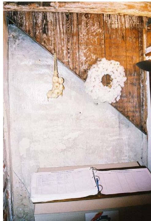
Figure 65: North wall of Room 104, east of fireplace. Note where exterior staircase penetrates the building. (Photo by author.)
