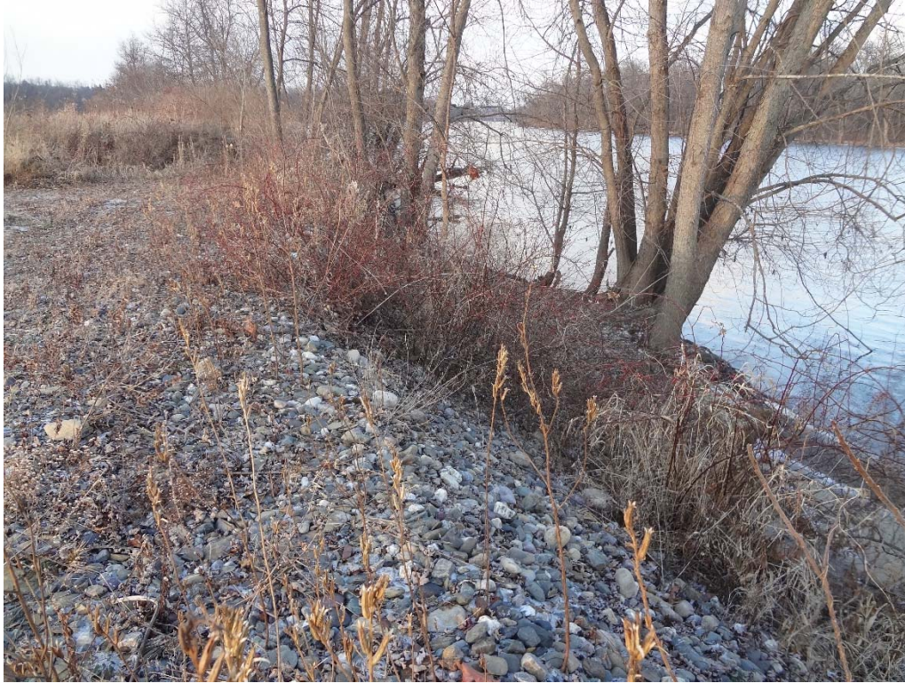
Photo 21. Photo shows imported stone fill located on the river bank directly south of the man-made drainage, to armor the bank from continued erosion.
