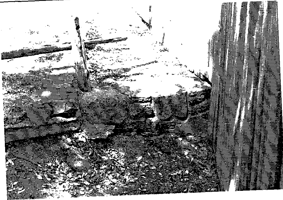
Figure 3-142 June 1996. Detail of a section of the wall which goes under the board fence into the amphitheater. This area needs backfilling and possibly some stabilization for the walkway.
