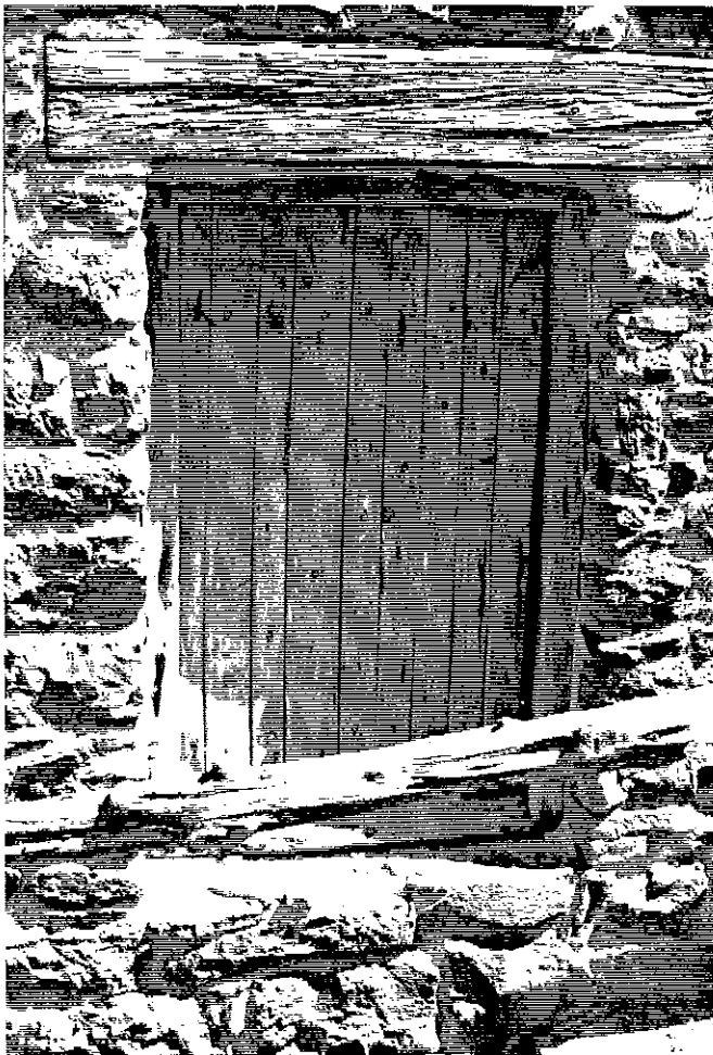
Figure 3-51 June 1996. Detail of the window in the west elevation. Condition of the masonry on the west elevation is excellent again with the exception of some pointing that needs to be done around the window.
