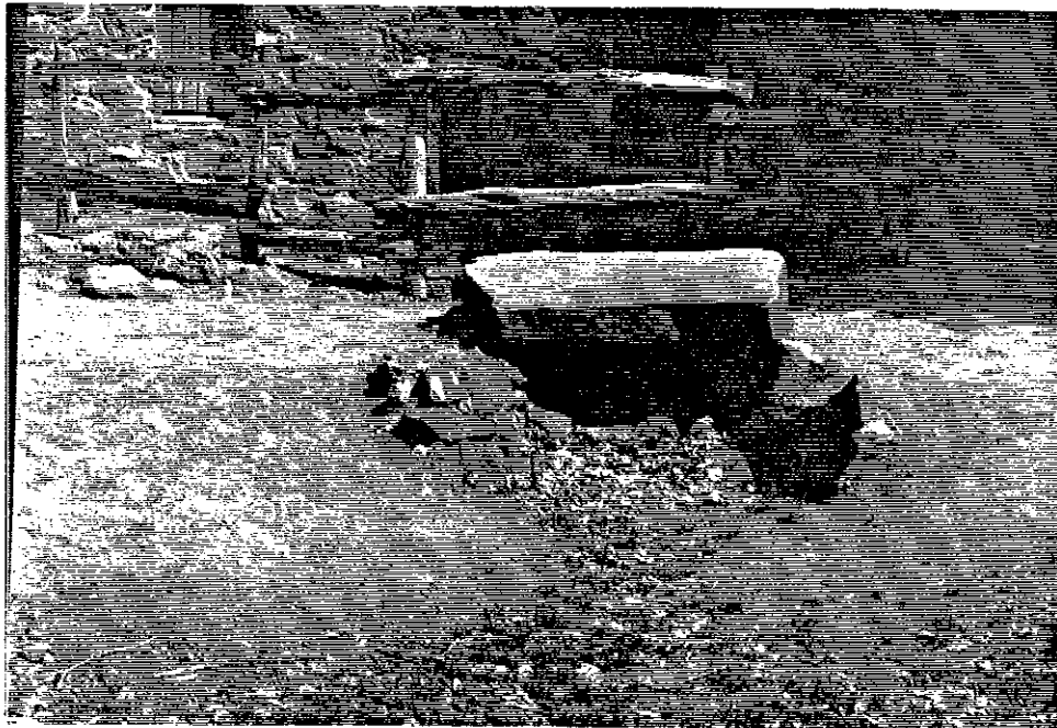
Figure 3-13 June 1996. Detail of the stone lined and stone covered sluice from the acequia to the forebay in front of the mill (prior to excavation).
