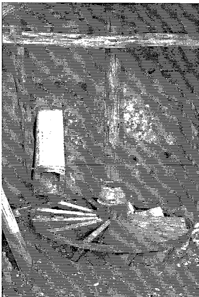
Figure 3-53 June 1996. Detail of the waterwheel, main shaft, and wooden water chute (at the left of the photograph). Remnant wooden pieces discovered at the beginning of the research for this report can also be seen. These wooden members were recorded in their found locations and were removed for safe-keeping and detailed measurements.
