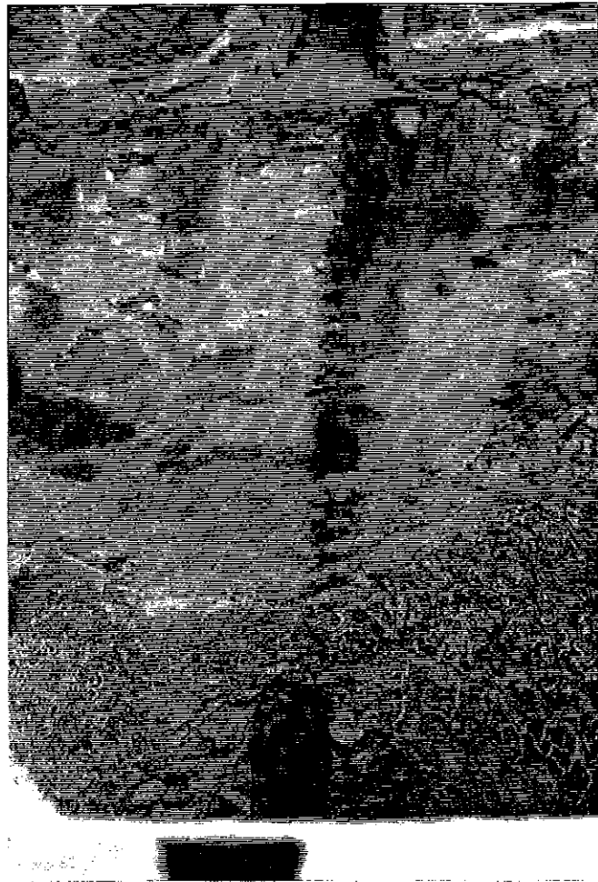
Figure 2-69 1981. Looking into the forebay. Note the presence of the forebay gate still in place.
