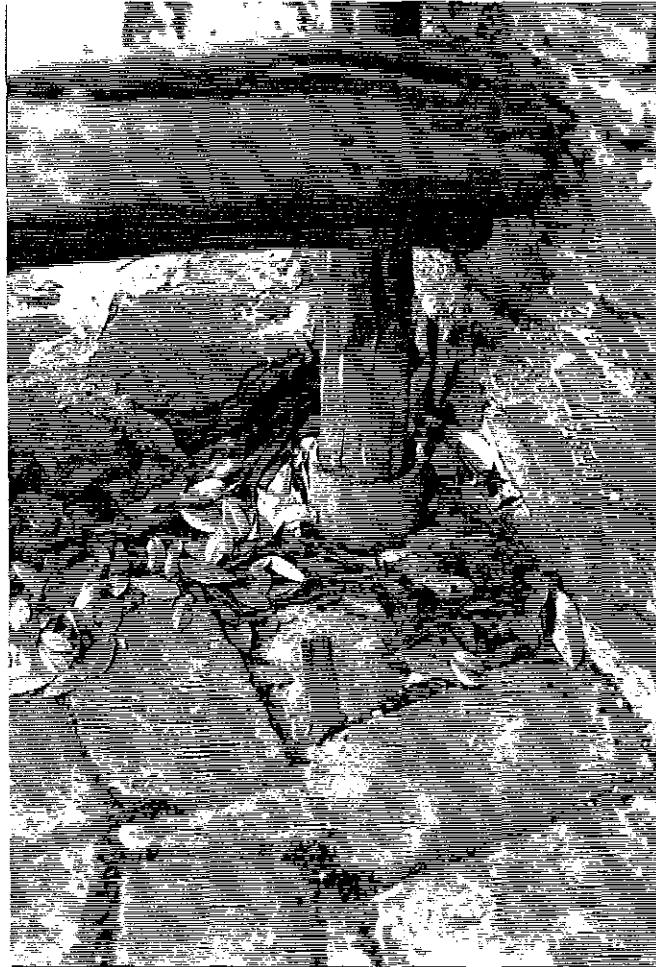
Figure 3-145 June 1996. Pipe embedded in pavement to support the cedar fence post for easy removal. This detail occurs at all posts surrounding the forebay.
