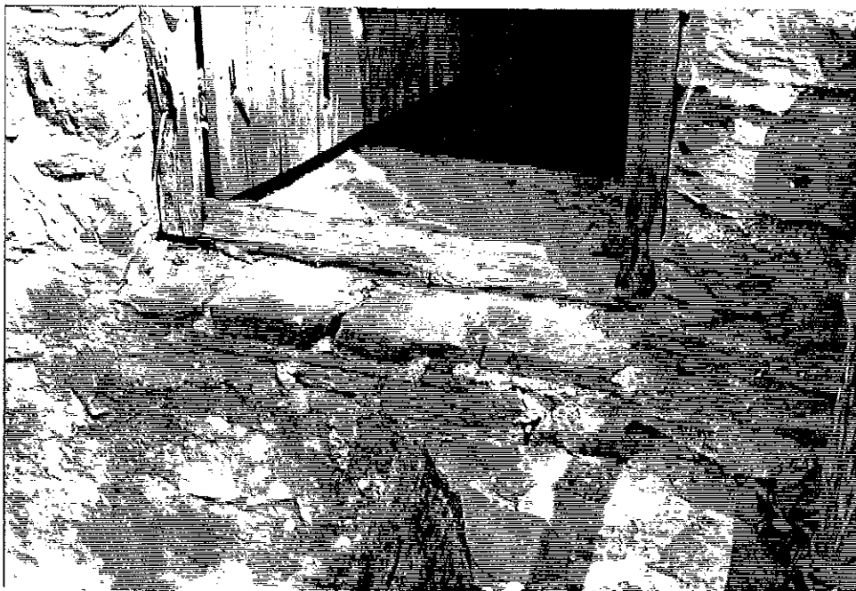
Figure 3-40 June 1996 Detail of the sill of the middle window in the south elevation (typical for all window sills). The condition of the sill is good, minor pointing is required.
