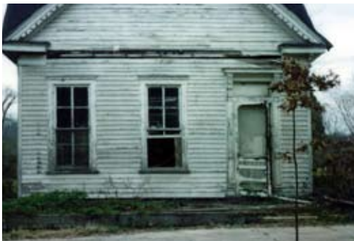
This 1880s cottage was in deteriorated condition prior to rehabilitation. Ghost marks of the missing porch are evident.
