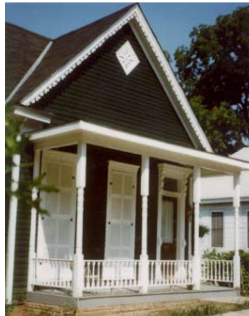
Left: In the course of rehabilitation, the owner installed new windows in a historic design, which extended to the first floor. Full-length blinds were also added.
