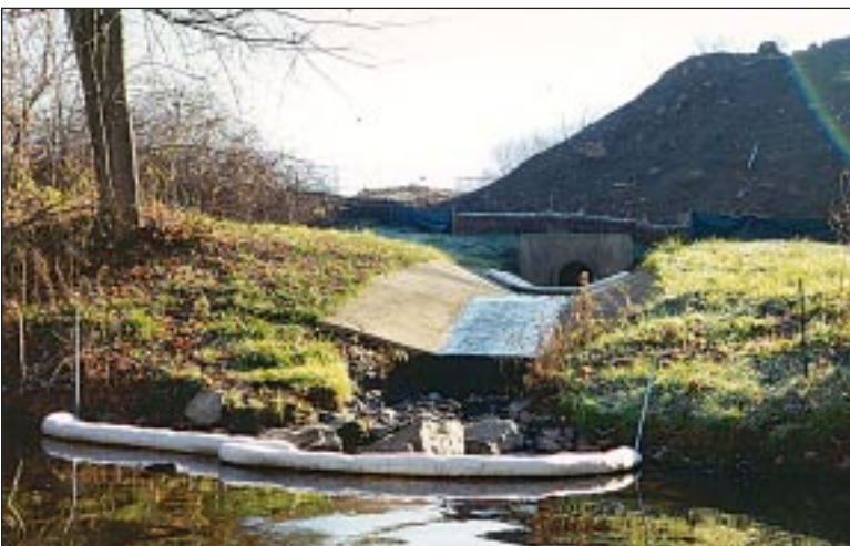
Stormwater outfall to the river
