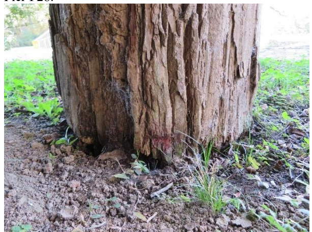
Photo 200. Deterioration and section loss at grade of Pier P29.
