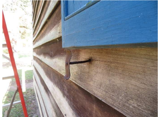
Photo 96. Shutter dog was present but did not engage shutter.
