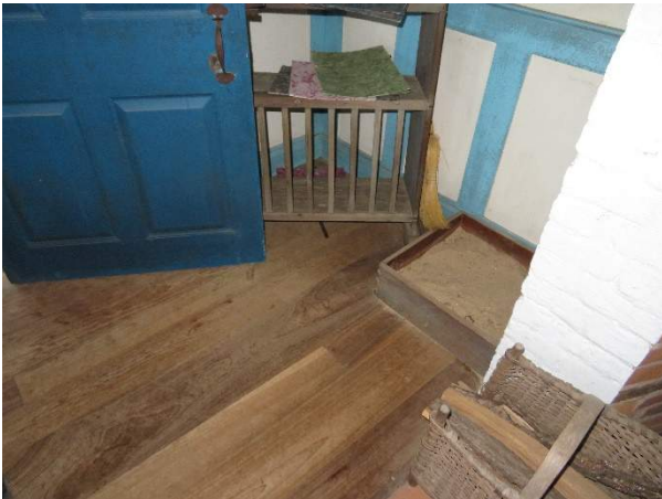
Photo 332. Wear to the flooring around Door D700.
