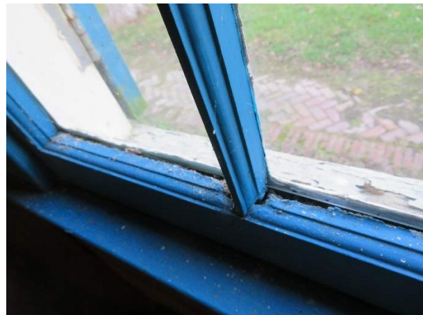
Photo 253. Deterioration of the interior muntin and rail of the lower sash.
