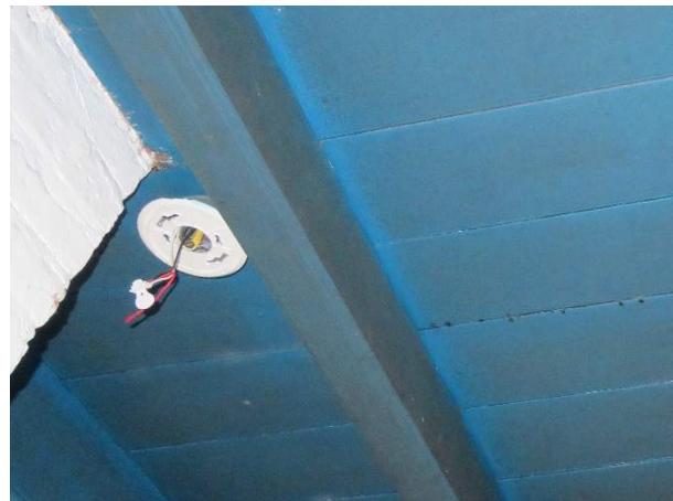
Photo 353. Damaged ceiling-mounted detector in Room 1 (101).
