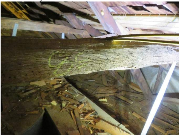
Photo 231. Wood boring insect damage to the collar tie in Rafter Bay R10.
