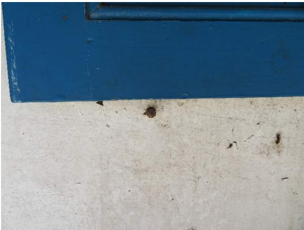
Photo 83. Missing shutter dog.
