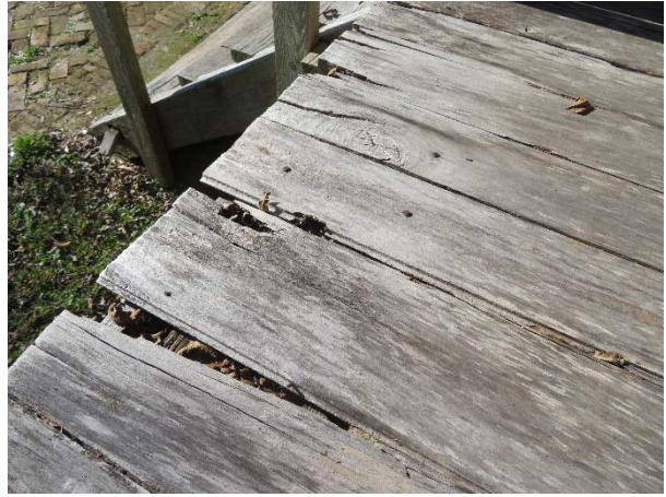
Photo 43. Deterioration of gallery decking.
