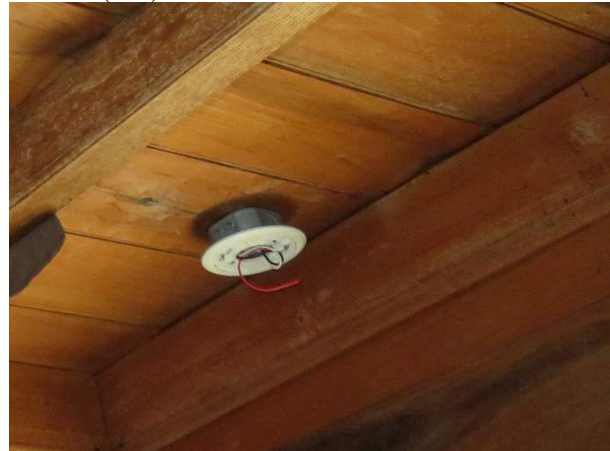
Photo 355. Damaged ceiling-mounted detector in Room 2 (102).
