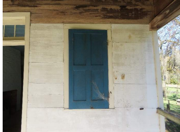
Photo 109. Window W700, overall with shutter closed, showing soiling from bats roosting behind shutter.
