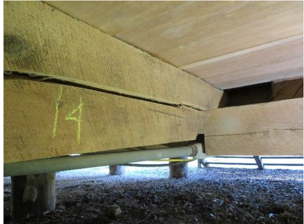
Photo 218. Beam B9 and Joist J24 modified for electrical conduit with distress at notch, looking south.
