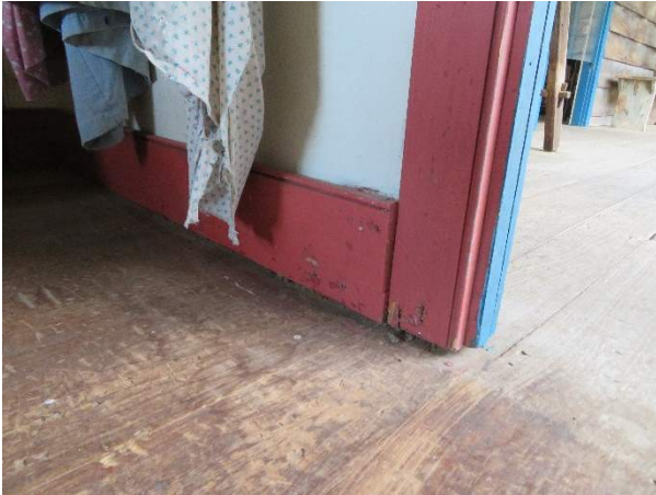
Photo 288. Minor deterioration of the bottom of the jamb trim, where the floor slope creates a gap at the base of the wall.
