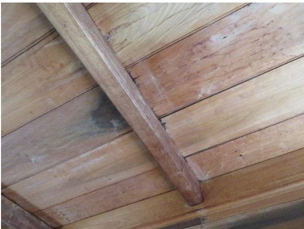
Photo 310. Unfinished ceiling planks with small area of discoloration, likely from water.
