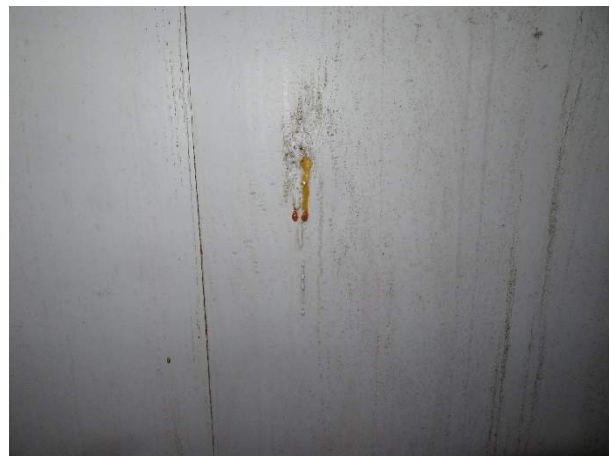
Photo 325. Sap seepage through wall board on the north wall.
