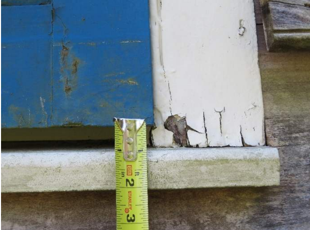
Photo 101. Deterioration of jamb.
