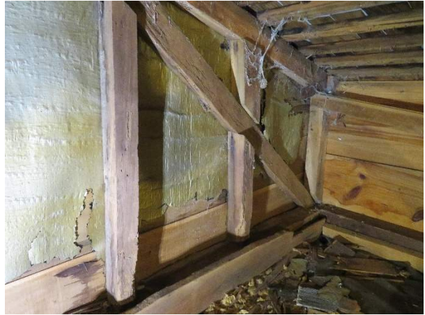
Photo 240. Squirrel damage to framing of east gable end wall.
