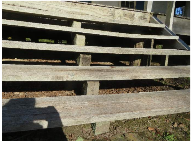
Photo 34. Displacement of center stringer and deflection of treads.
