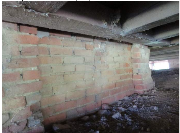
Photo 72. Foundation of central chimney, showing mortar loss and minor cracking.
