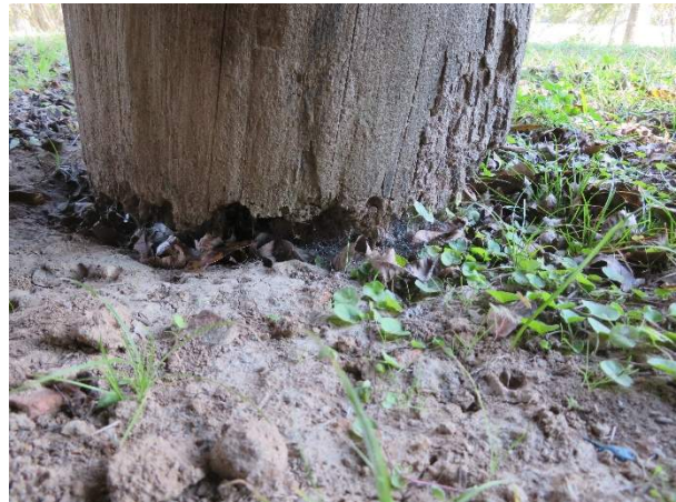
Photo 166. Deterioration at the base of Pier P6.
