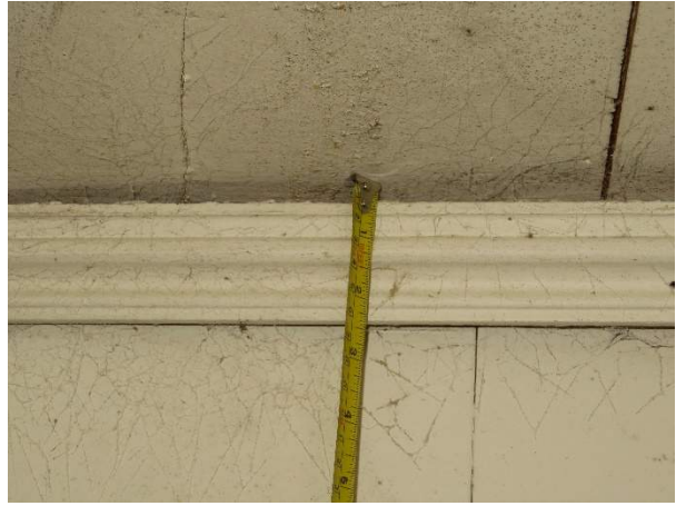
Photo 329. Displaced and loose ceiling moulding.
