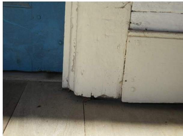
Photo 123. Minor weather-related deterioration of base of jamb trim.
