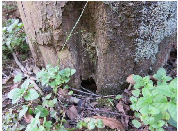
Photo 196. Deterioration of the core of Pier 27.
