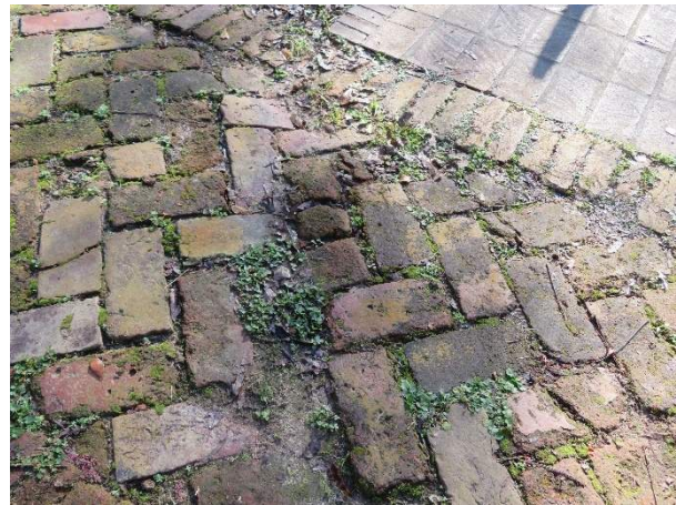
Photo 14. Displacement and deterioration of brick pavers.
