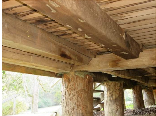
Photo 206. Floor framing system below the Front Gallery (108) at Pier P5, looking west showing joists running east-west.
