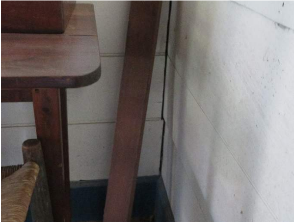
Photo 300. Separation of the wall boards at the southeast corner, likely due to natural expansion and contraction.
