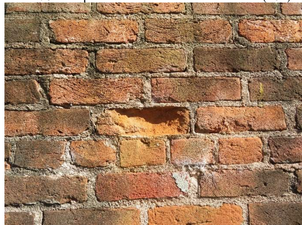
Photo 78. Localized deterioration of brick units at west chimney.
