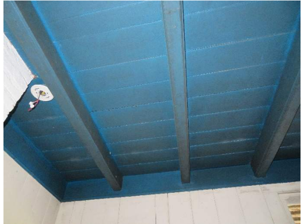
Photo 301. Ceiling planks, looking south, showing discoloration on the paint from mildew.
