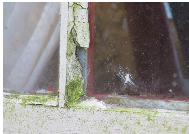
Photo 107. Failed glazing putty.
