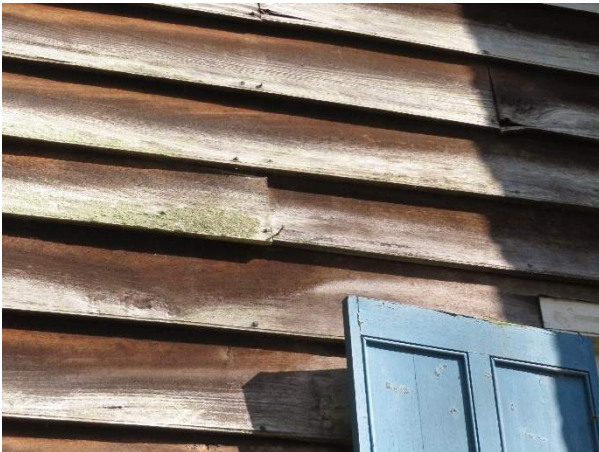
Photo 61. Warping and age-related deterioration of weatherboard siding at east wall.
