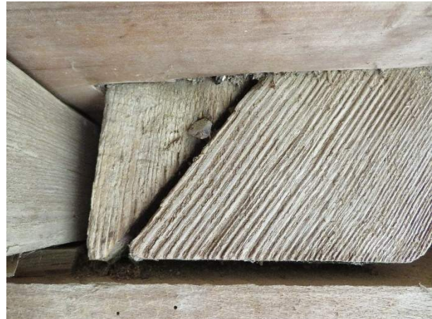
Photo 220. Wall members for north wall of Room 2 (102), near Joist J18 and bearing on Beam B15, with a forged nail.
