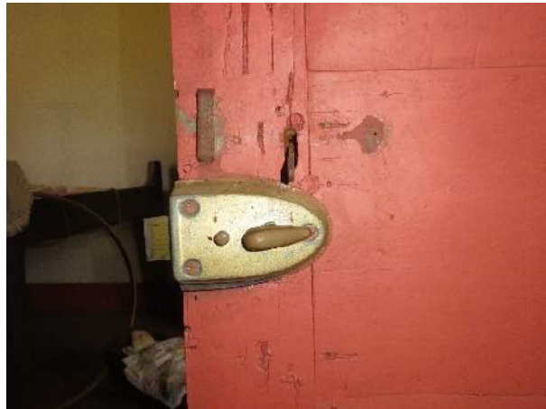
Photo 287. Lacquered metal rim lock, missing interior lift-latch components, and damage to the door stile.
