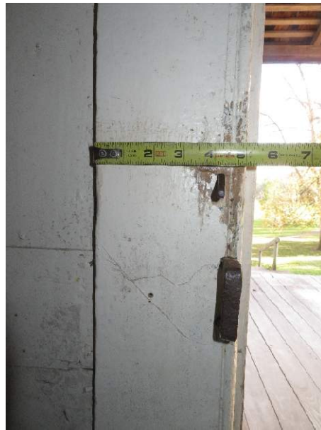
Photo 270. Jamb catch for the lift-latch and rim lock, showing damage to the finishes on the jamb trim.
