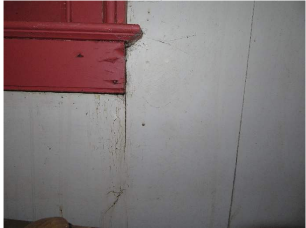
Photo 257. Evidence of water intrusion and water damage at the lower right corner of the window.
