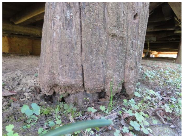
Photo 198. Deterioration and section loss at the base of Pier P28.
