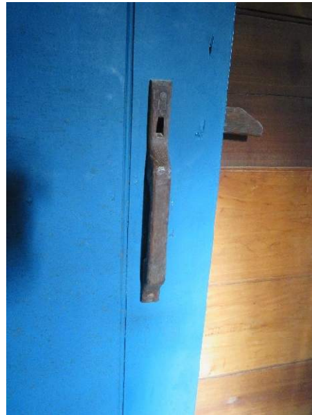
Photo 277. Damaged exterior handle of Door D201.
