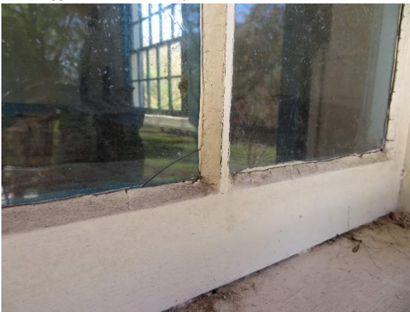
Photo 87. Small crack in glazing in lower sash.
