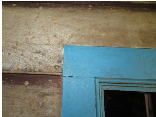
Photo 142. Minor separation of jamb and head trim.
