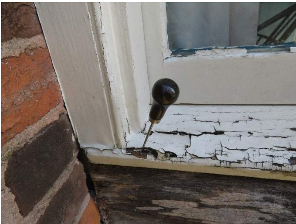
Photo 91. Severe deterioration of the sill.
