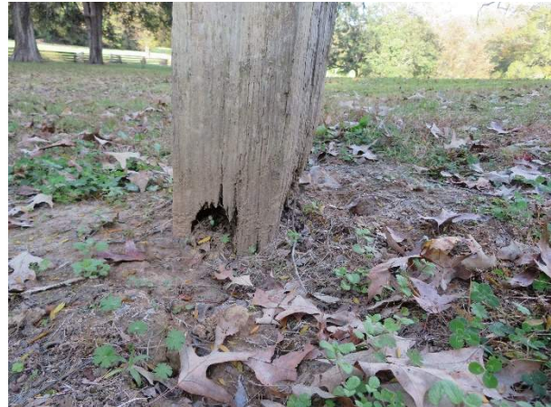
Photo 20. Deterioration of the wood post at grade.
