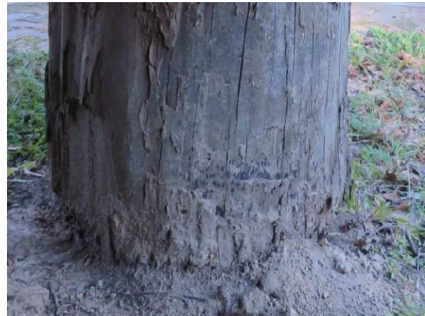
Photo 168. Deterioration at the base of Pier P7.
