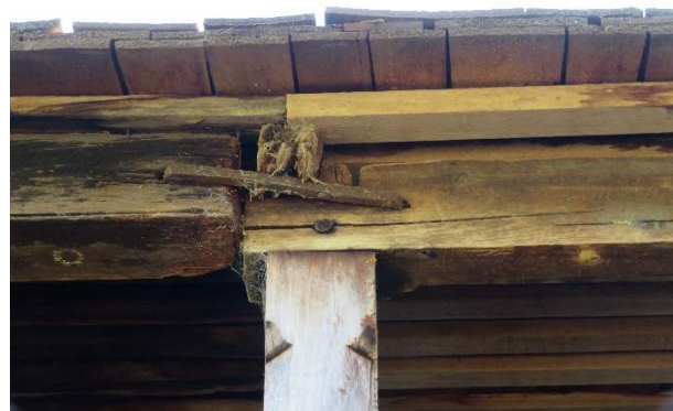
Photo 47. Distress to gallery top plate splice.
