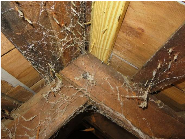
Photo 227. Distress and slight displacement at the ridge connection of Rafter Bay R8.
