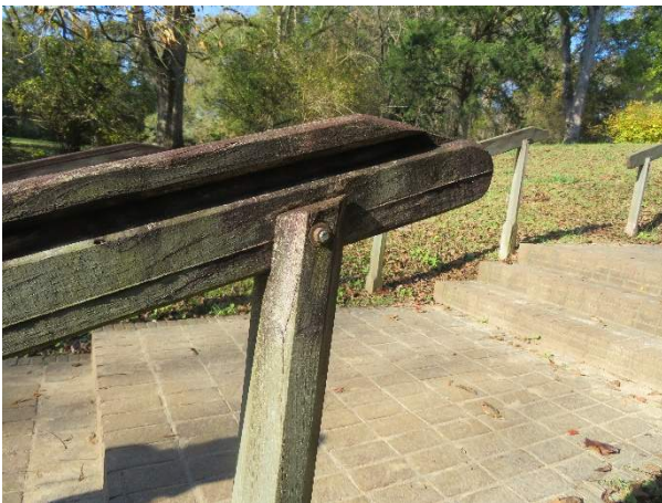
Photo 11. End of handrail at an intermediate landing, showing lack of extension and the “notch” for gripping.
