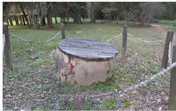
Photo 26. Cistern #1 to the northwest of the main house has failed.
