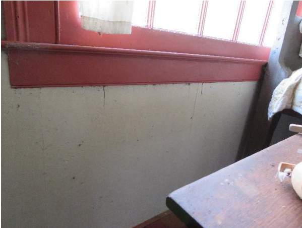
Photo 260. Evidence of water intrusion at the wood panels below the window.
