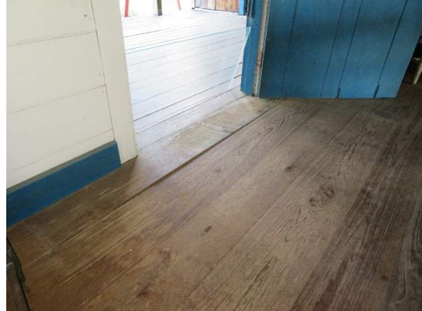
Photo 297. Heaving and abrasion of the floor boards at the threshold of Door D101.
