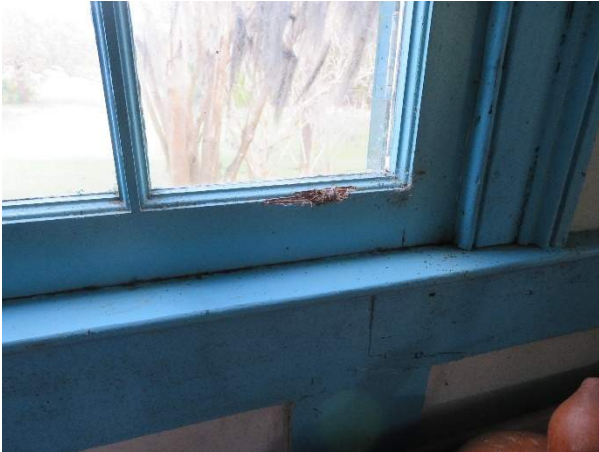
Photo 267. Damage to lower sash, potentially from squirrels.
