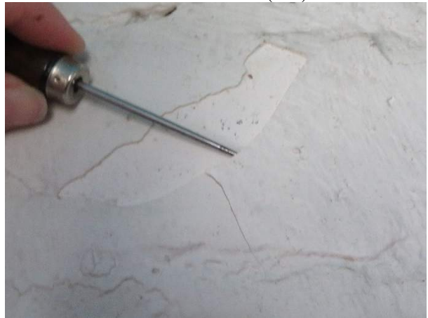
Photo 70. Paint surface failure, exposing lower layers of white paint in Room 7 (107).
