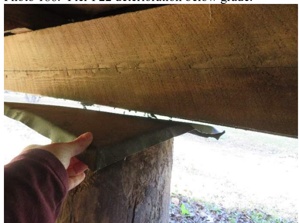
Photo 188. Pier P23 was no longer in contact with the perimeter beam.
