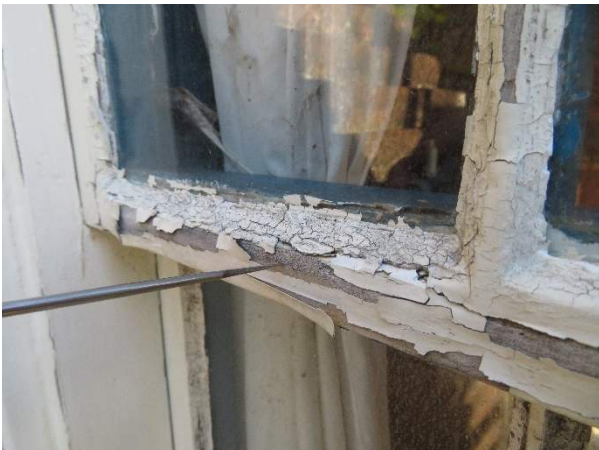
Photo 93. Failed glazing putty and minor deterioration of the upper sash meeting rail.
