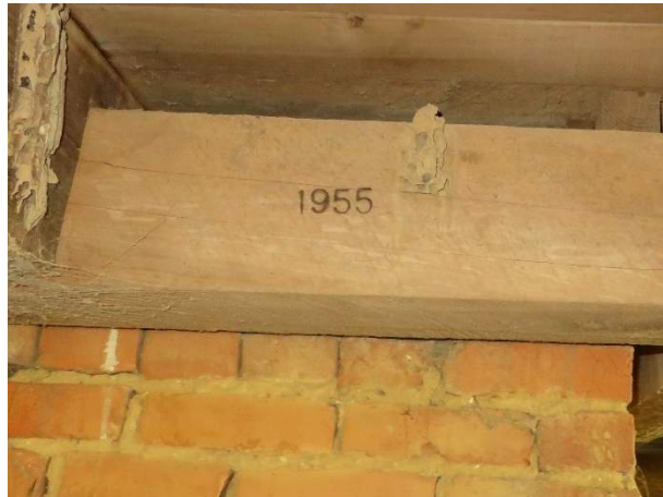
Photo 210. Typical identifying brand on Beam B11, indicating the member was replaced during the 1955 restoration.
