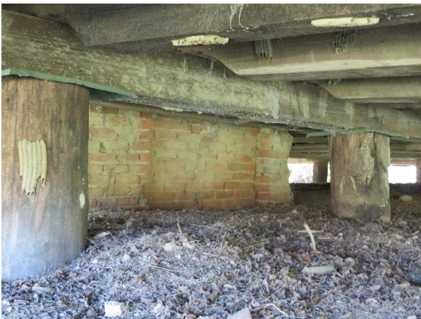
Photo 203. Floor framing system, showing foundation piers, beam, and joists, below Room 6 (106) looking south showing joists running north-south.
