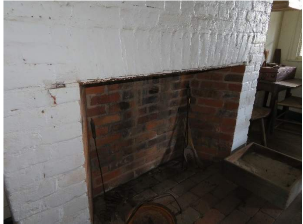
Photo 68. Distress and displacement of brick due to corrosion of steel lintel in Room 1 (101).
