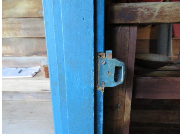
Photo 285. The strike plate at the jamb, showing abandoned screw holes from the strike plate being adjusted. The strike plate is original to the lock.
