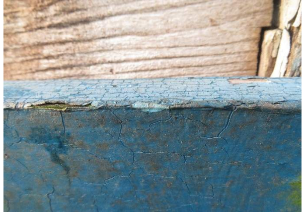
Photo 115. Failure of painted surfaces and minor deterioration of top rail of shutter.
