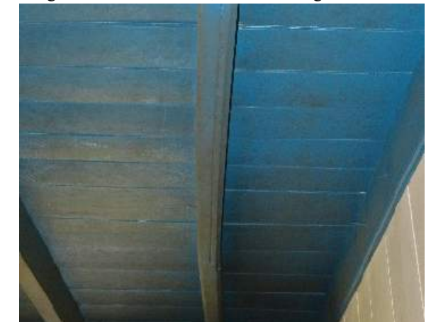
Photo 305. Out of plumb ceiling beam splice, as depicted on the 1940 HABS drawings.
