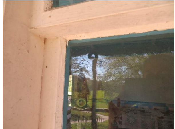
Photo 86. Imperfections in glazing.
