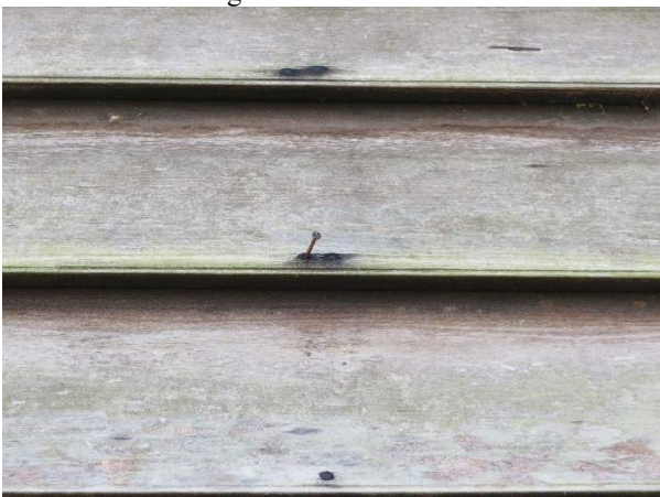
Photo 65. Warping and fastener backout of weatherboard siding.
