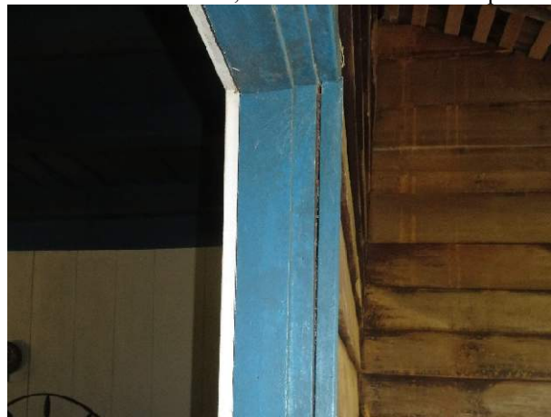
Photo 127. Minor separation of door stop and jamb.
