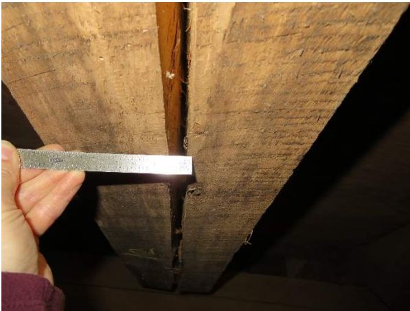
Photo 211. Deep checking of Joist J29.
