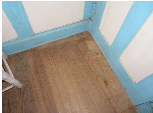
Photo 333. Wear to the flooring from abrasion by Door D701.
