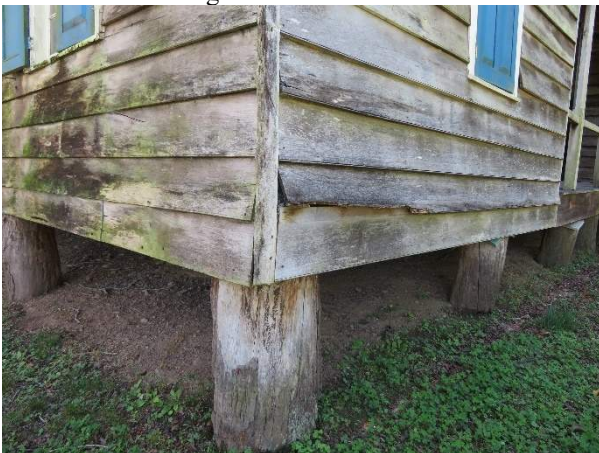
Photo 63. Biological growth and severe deterioration of weatherboard siding at northeast corner.
