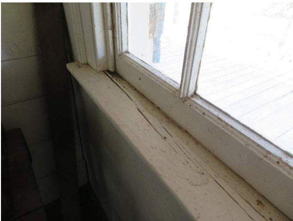
Photo 246. The interior sill had failed due to water damage.
