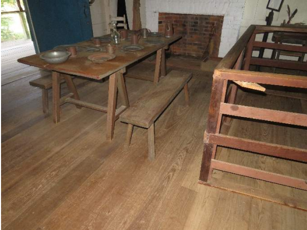
Photo 296. Wear of the flooring around the dining table, looking east.
