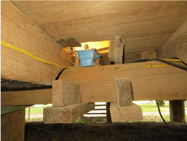
Photo 344. Romex and other unshielded electrical lines in the crawlspace, feeding the floor receptacle.
