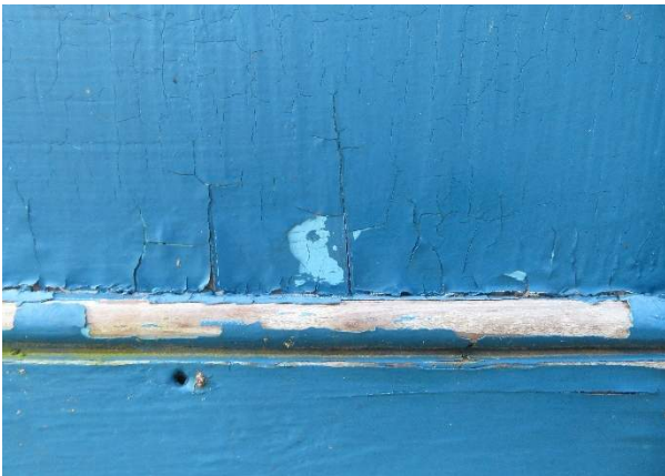
Photo 116. Failure of painted surfaces of shutter, showing multiply layers of blue paint.
