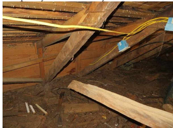
Photo 230. Failed collar tie at the south primary rafter in Rafter Bay R9.
