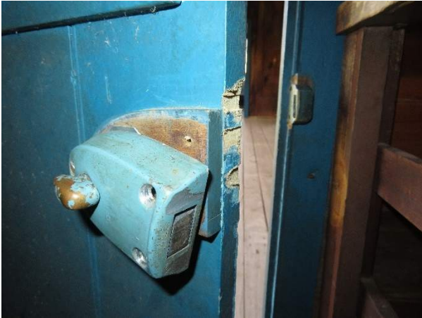
Photo 284. Damaged and partially disengaged rim lock, with damage to the edge of the door where it meets the jamb strike plate.
