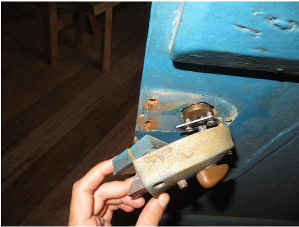
Photo 274. Broken rim lock.
