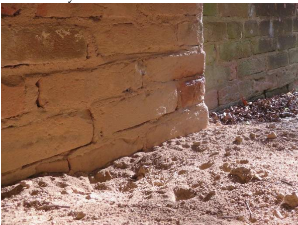
Photo 79. Mortar loss at base of west chimney.
