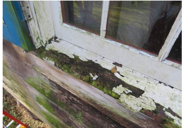
Photo 103. Severe deterioration of the sill.
