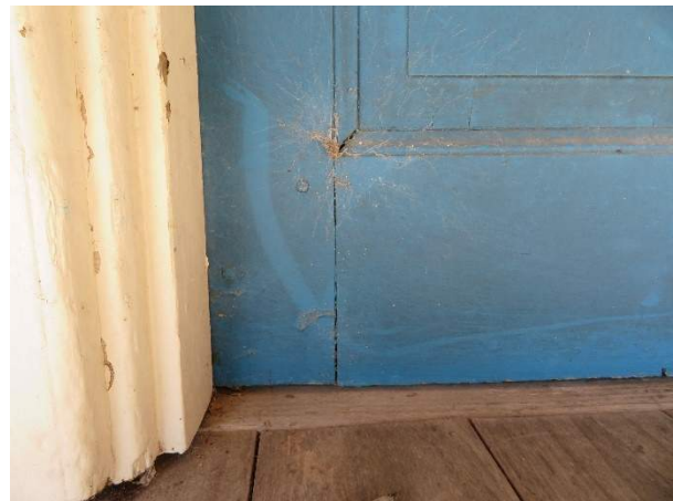
Photo 121. Minor separation of lower rail and stile of door.
