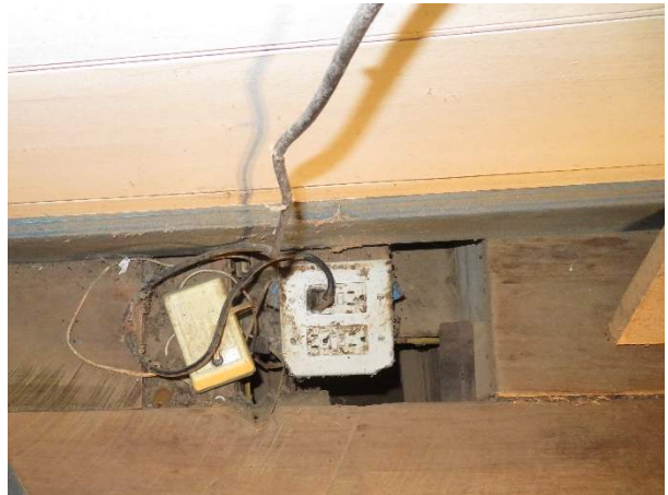
Photo 347. Damaged floor receptacle in Room 1 (101).
