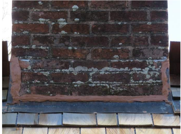
Photo 74. Central chimney above roof, which lichen growth on the north face.
