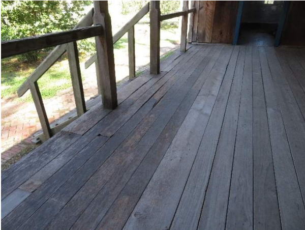
Photo 48. Deterioration of gallery decking.
