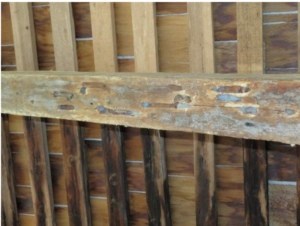
Photo 46. Carpenter bee damage to gallery beams.
