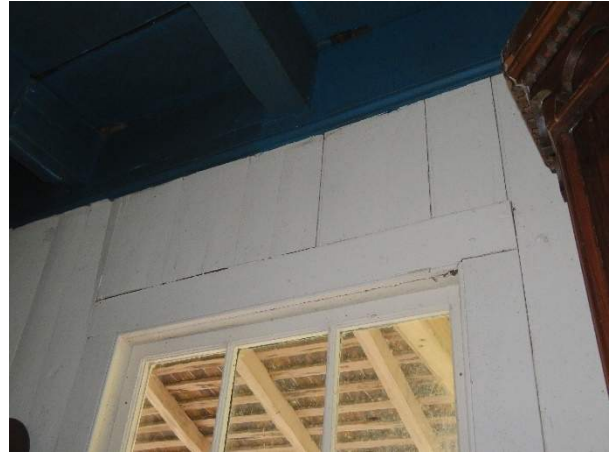
Photo 242. Head trim of Window W100, showing distress to the right-hand corner.
