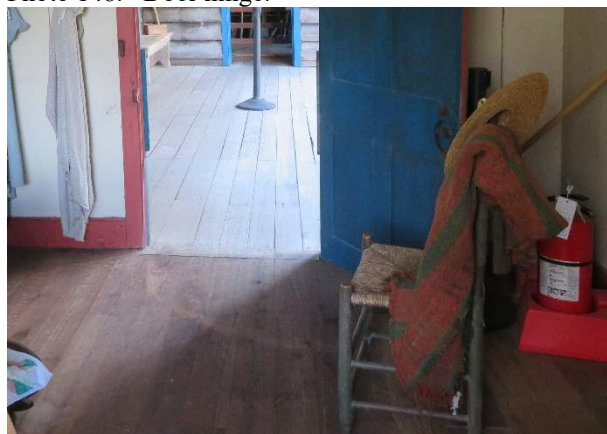
Photo 150. Abrasions to floor boards from door swing.
