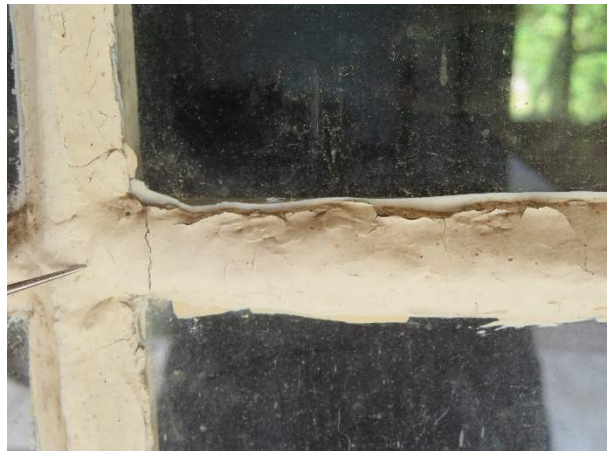
Photo 84. Failed replacement glazing putty.
