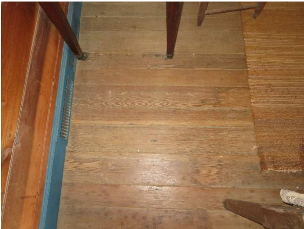
Photo 308. Minor areas of wear to the flooring.
