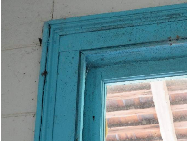
Photo 263. Minor separation of wood joints at the trim. Note the mildew on the painted surfaces.
