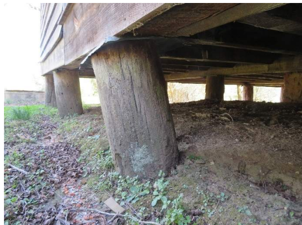
Photo 194. Pier P27 is displaced and has settled due to deterioration and is no longer supporting the perimeter beam.
