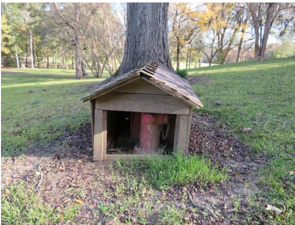
Photo 351. Hydrant, located approximately 50 feet north of the main house.
