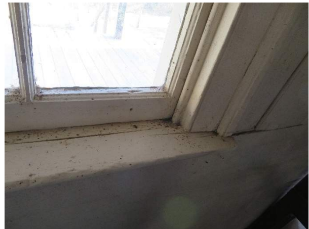
Photo 247. The interior sill had failed due to water damage.
