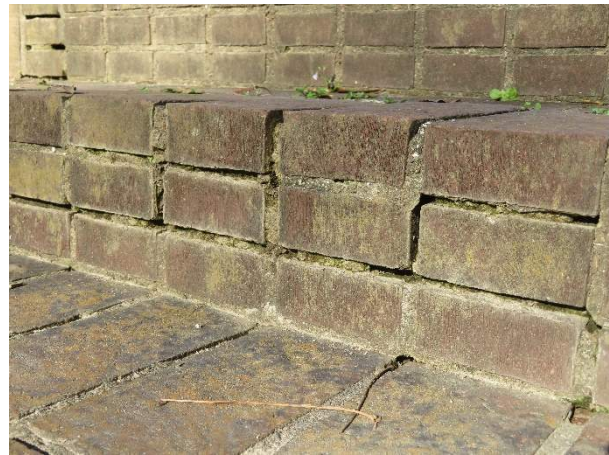
Photo 10. Localized deterioration of mortar joints between paving bricks.
