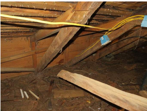
Photo 342. Romex and other unshielded electrical lines in the attic.
