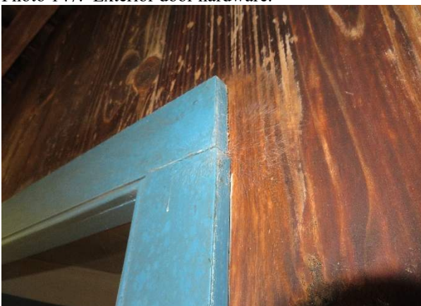
Photo 149. Minor separation of jamb and head trim.
