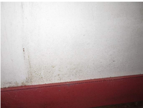
Photo 326. Mildew or biological growth on the wall board at the north wall.
