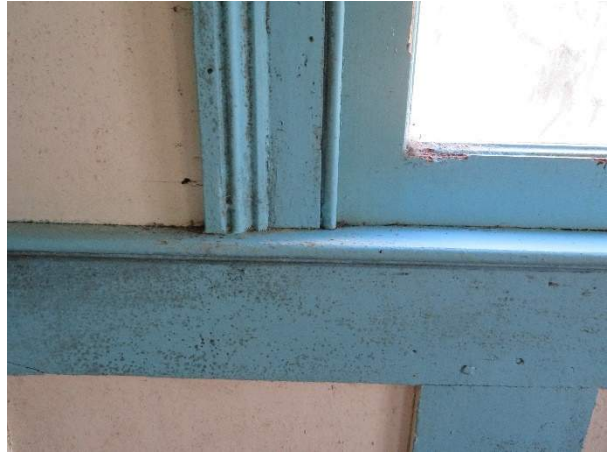
Photo 268. Damage to lower sash, potentially from squirrels. Note the mildew on the painted surfaces.
