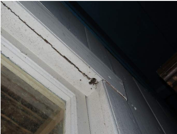
Photo 243. Detail of distress to head trim, showing separation of trim pieces and deterioration of wood.
