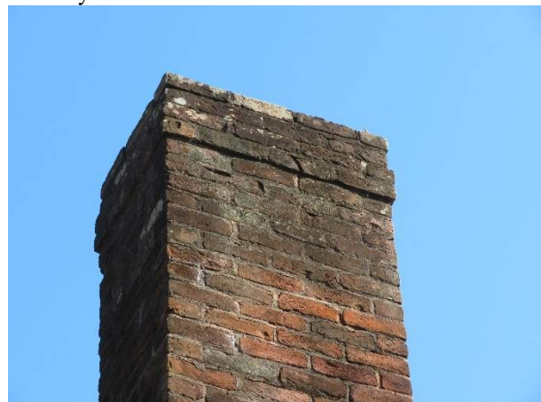
Photo 80. Deterioration of mortar at top of west chimney.
