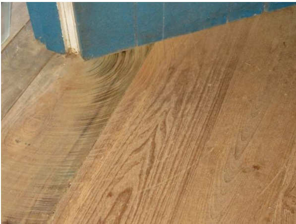
Photo 128. Abrasion to the flooring from door swing.
