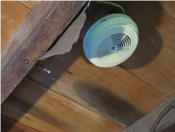
Photo 354. Ceiling-mounted detector in Room 3 (103).
