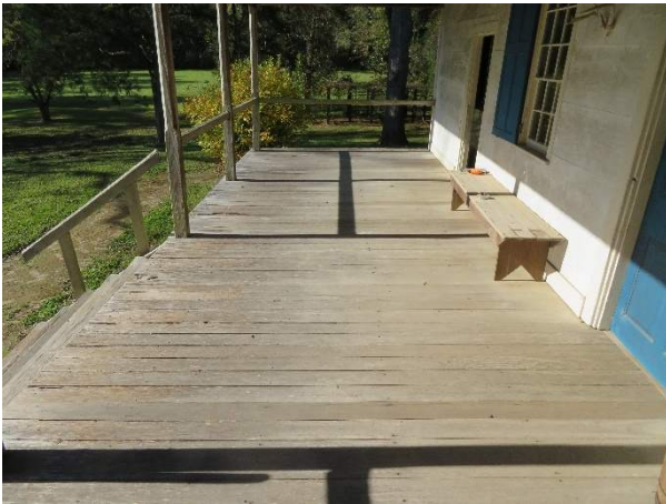
Photo 38. Decking of south gallery, showing wear and deterioration at stairs.
