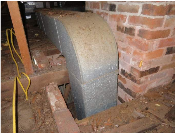
Photo 348. Abandoned HVAC unit in attic.
