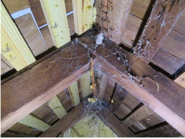
Photo 54. Spaced sheathing at ridge, with recent replacement boards on the left.
