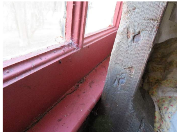
Photo 259. Water damage and wood deterioration at the interior sill.
