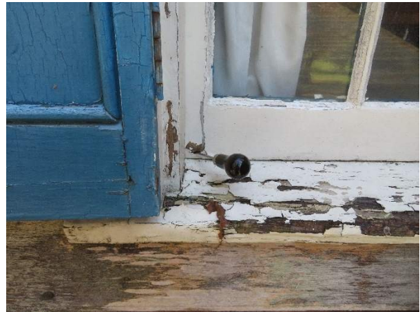
Photo 98. Severe deterioration of the sill and lower left jamb.
