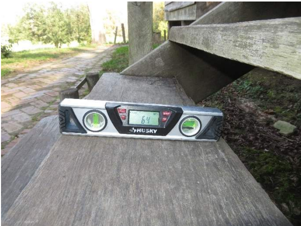
Photo 36. Excessive and uneven backwards slope of treads.
