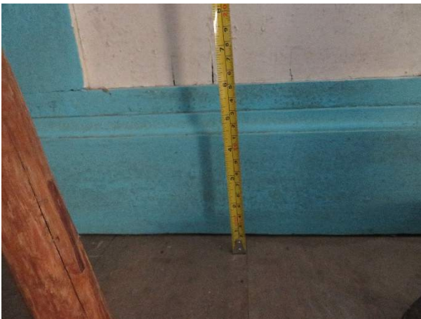
Photo 340. Heavy mildew growth on the baseboard.
