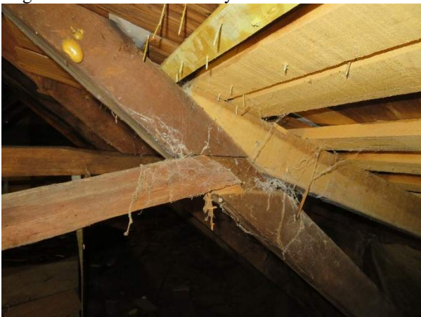
Photo 229. Failed collar tie at the north primary rafter in Rafter Bay R9.
