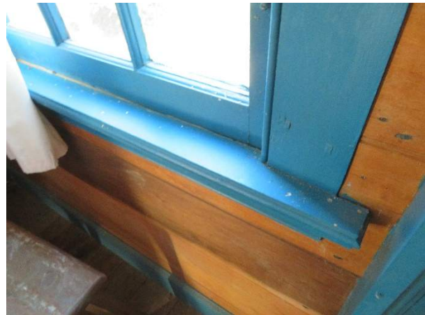
Photo 249. The interior sill of window W200 was in good condition, despite the poor condition of the exterior sill.
