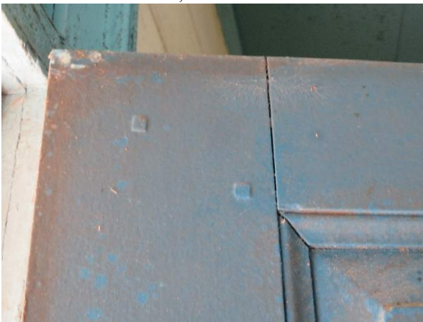
Photo 153. Connection detail of rail and top stile at door D700 with minor separation.
