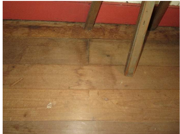
Photo 323. Water stains on the flooring at the north wall under Window W600.
