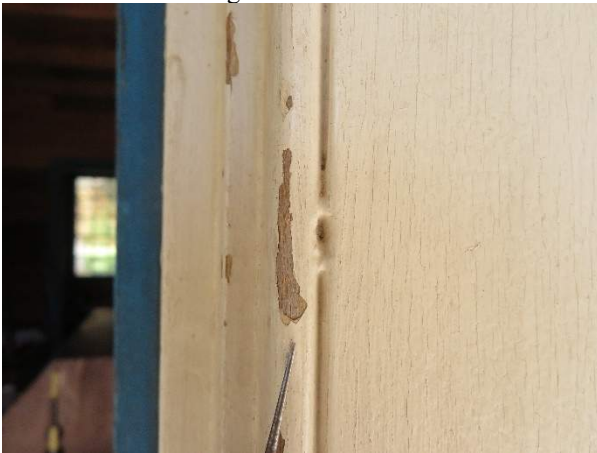
Photo 133. Failure of painted surfaces at door jamb.
