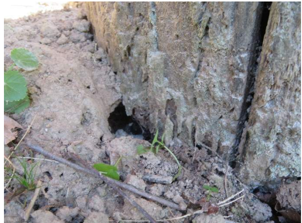
Photo 186. Pier P22 deterioration below grade.
