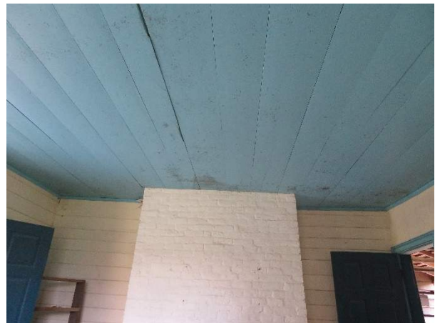
Photo 335. Ceiling boards, showing deflected board.
