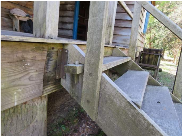
Photo 37. Distress to stair support at gallery rim joist.
