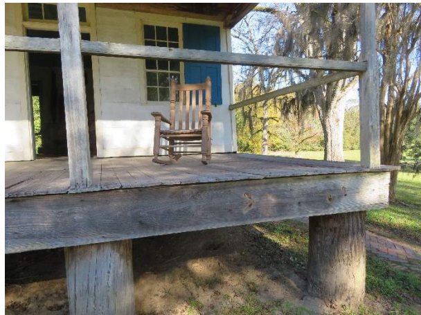
Photo 41. Deflection of decking near Room 7 (107).
