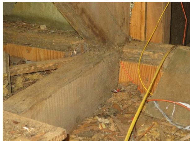
Photo 343. Romex and other unshielded electrical lines in the attic.
