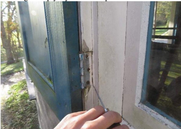
Photo 118. Distress to jamb at replacement hardware.
