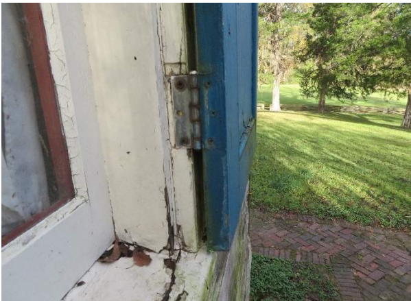
Photo 104. Deterioration of the sill and distress to the jamb at replacement hardware for right shutter.
