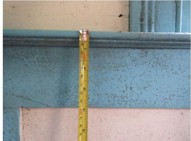
Photo 339. Heavy mildew growth on the top rail of the wainscot.
