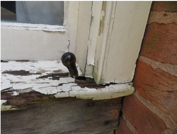
Photo 97. Severe deterioration of the sill and lower right jamb.
