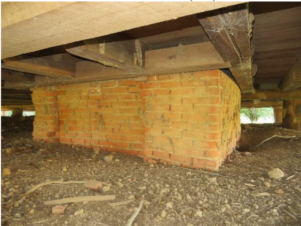
Photo 71. Foundation of central chimney, showing mortar loss with minor cracking and animal burrow.
