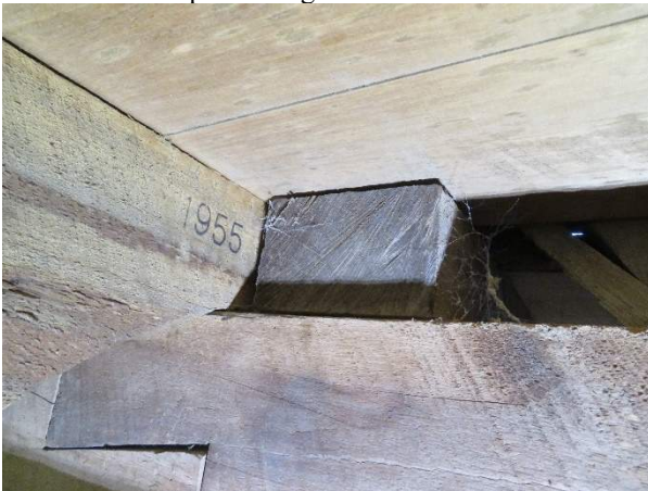
Photo 213. Joists J23 and J47 bearing ends at Beam B16 splice over Pier P17, looking north.
