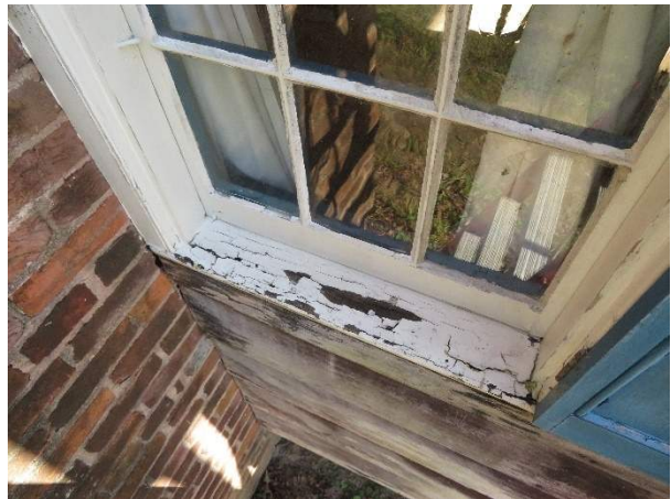
Photo 92. Severe deterioration of the sill.
