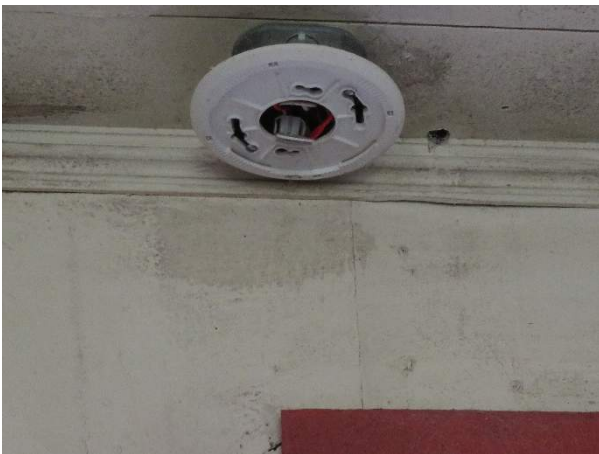
Photo 352. Damaged ceiling-mounted detector in Room 6 (106).
