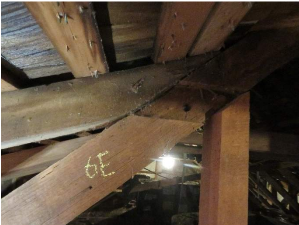
Photo 233. Missing collar tie replaced by a vertical post in Rafter Bay R12.
