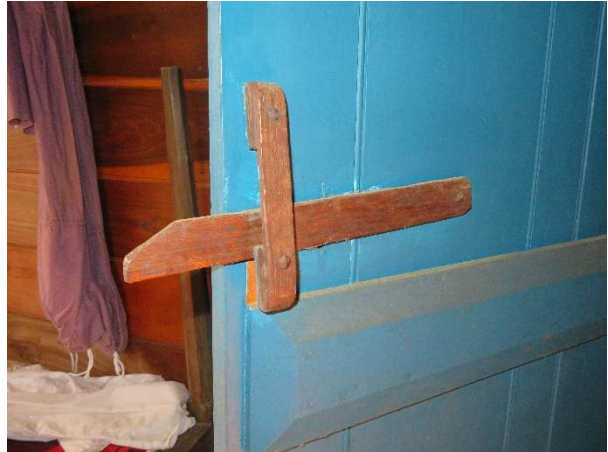
Photo 279. Loose and damaged interior hardware of Door D201.
