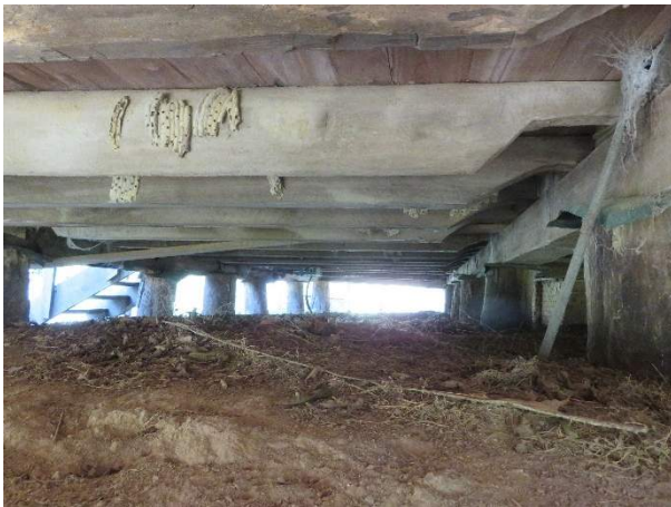
Photo 201. Uneven grade of soil in crawlspace, looking east.
