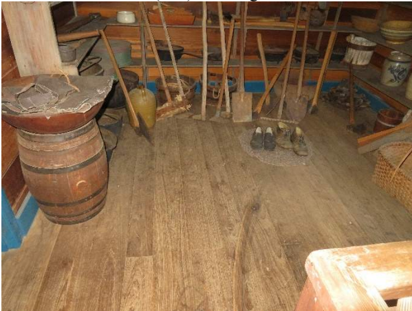
Photo 316. Evidence of minor wear on the flooring.
