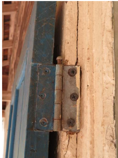
Photo 82. Distress to jamb at replacement shutter hardware.
