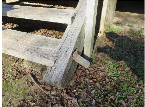
Photo 32. Deterioration of tread connection.
