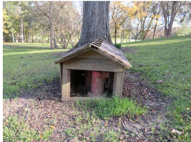
Photo 22. Wood shed over fire hydrant.
