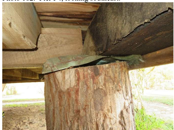
Photo 164. Copper flashing at the head of Pier P5, showing displacement of the pier.
