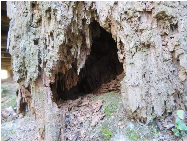
Photo 191. Pier P25 has significant loss of section due to internal and below-grade deterioration.
