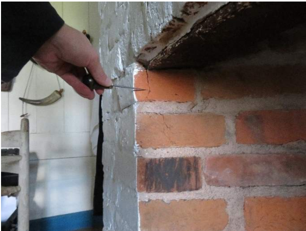
Photo 69. Distress and displacement of brick due to corrosion of steel lintel in Room 1 (101).
