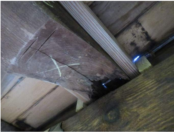
Photo 207. Joist J48, showing deterioration and sister repair at north bearing end. This is typical of several joists at the north.
