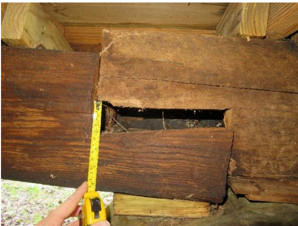
Photo 215. Beam B20 and B21 splice at Pier P25, showing 2-inch displacement due to settlement of the foundation piers at the northeast corner.
