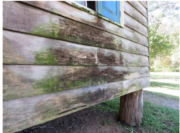
Photo 62. Biological growth and severe deterioration of weatherboard siding at northeast corner.
