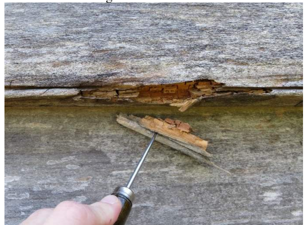
Photo 64. Deterioration of wood.
