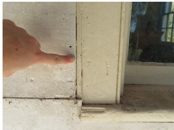
Photo 113. Minor distress to lower left jamb.
