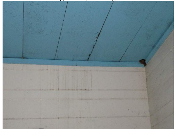
Photo 337. Deterioration of ceiling board and water stains on the wall finishes in the southeast corner.
