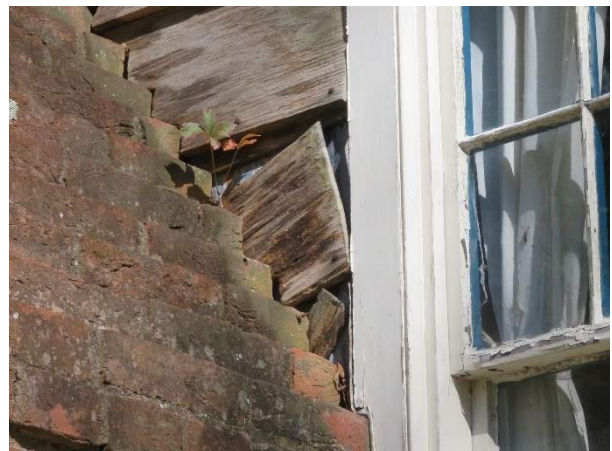
Photo 66. Loose and deteriorated siding at west wall behind brick chimney.
