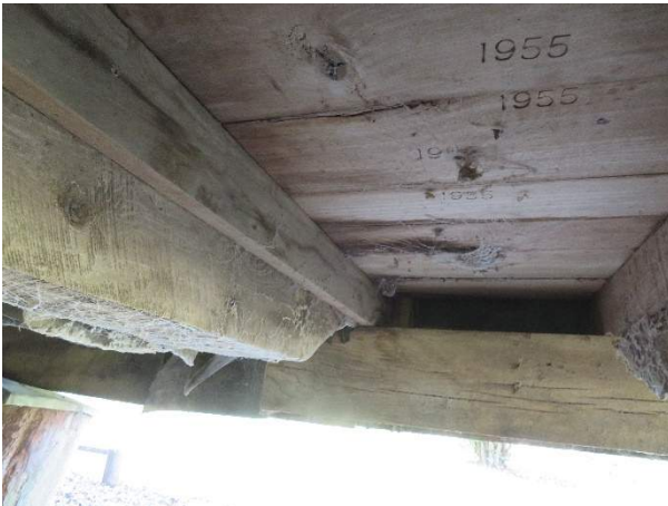
Photo 322. The underside of floorboards from the crawlspace, showing marks from the 1955 restoration.
