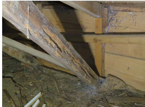
Photo 228. Termite damage at the bearing end of the south primary rafter in Rafter Bay R9.
