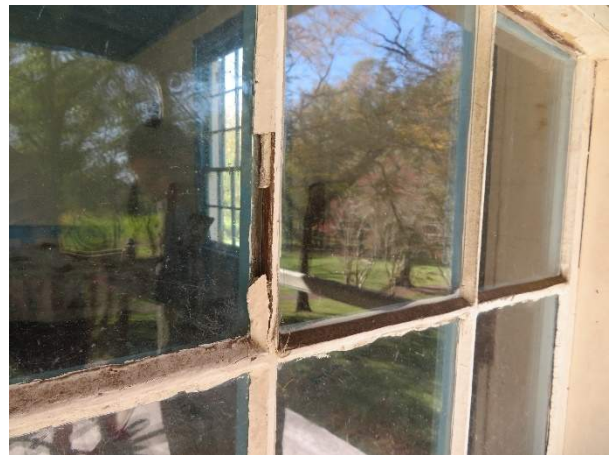
Photo 88. Failed glazing putty.
