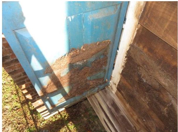
Photo 94. Soiling and guano from bats roosting being the shutters.
