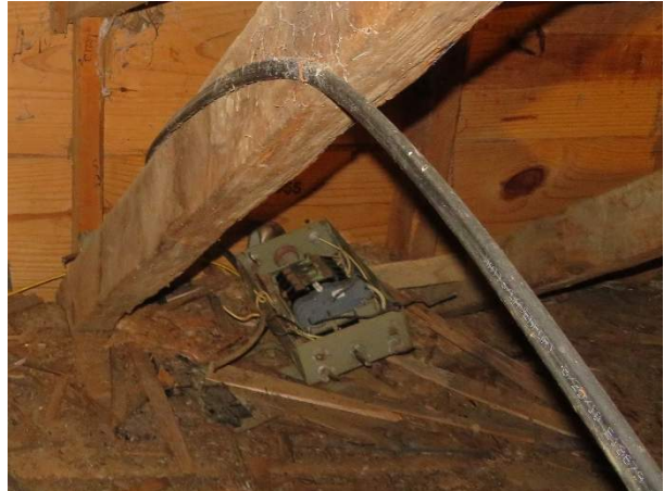
Photo 345. Damaged electrical panel in the attic.
