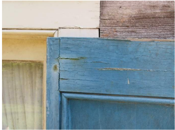
Photo 90. Minor deterioration of upper rail and stile of shutter.
