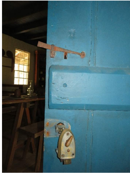
Photo 273. Interior door hardware, showing lift-latch and broken rim lock.
