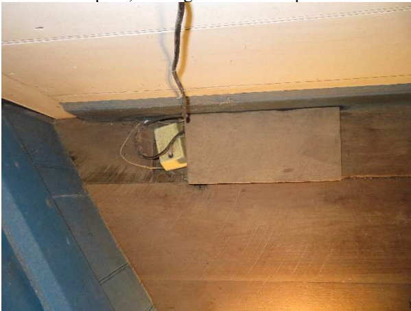
Photo 346. Damaged floor receptacle in Room 1 (101).
