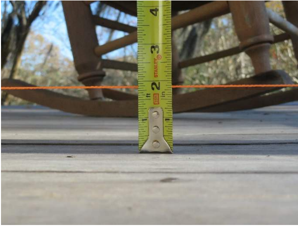
Photo 42. Deflection at deepest point.
