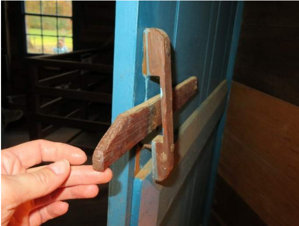
Photo 278. Loose and damaged interior hardware of Door D201.
