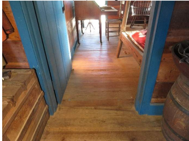
Photo 317. Wear on the flooring at the threshold to Room 2 (102).
