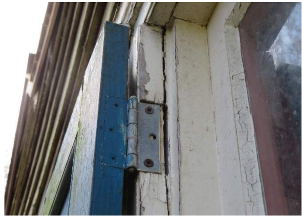
Photo 105. Distress to jamb at replacement hardware for left shutter.
