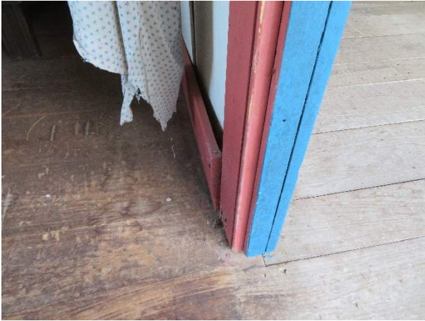
Photo 328. Displaced and loose base board near Door D600.
