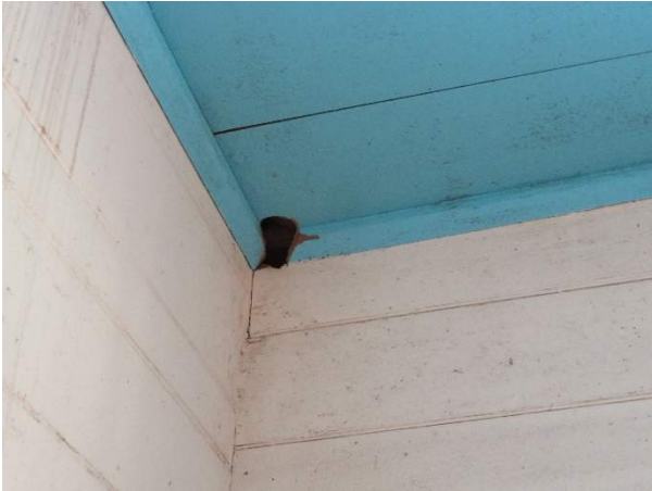
Photo 338. Pest hole in the southeast corner.
