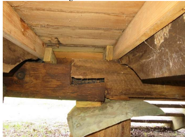
Photo 214. Beam B20 and B21 splice at Pier P25, showing displacement due to pier settlement, looking north.
