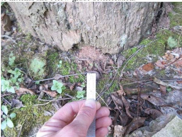
Photo 193. Deterioration at the base of Pier P26 with frass from a wood-boring insect.
