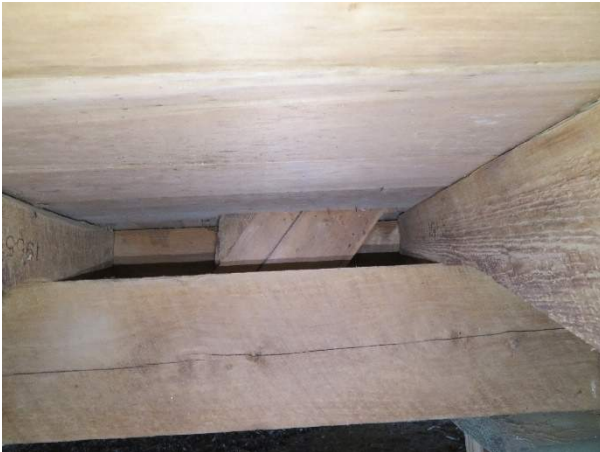
Photo 219. Wall member for the south wall of Room 2 (102), bearing on Beam B8. Note the joists on either end are branded with “1955”.
