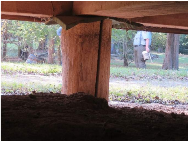
Photo 177. Pier P15, looking west, showing vertical split in pier.
