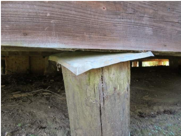
Photo 195. Pier 27 was no longer in contact with the perimeter beam.
