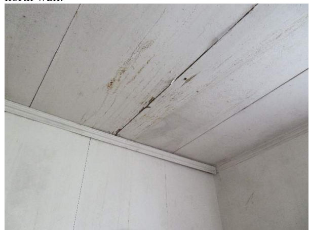
Photo 327. Water damage to the ceiling boards.
