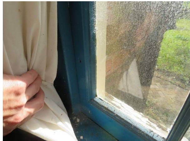
Photo 251. The interior of the lower sash and sill were in good condition, despite the poor condition of the window exterior.
