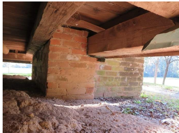
Photo 216. Beam B14 bearing end at west chimney with copper capillary break, looking south.
