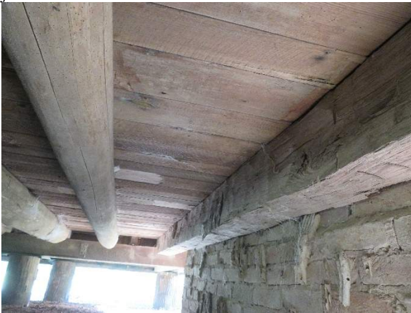
Photo 209. Reused or salvaged puncheon joists (J17 and J18) and a reused or salvaged hewn joist (J16), under Room 2 (102) looking south.
