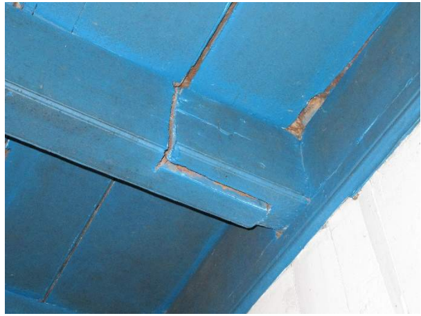
Photo 303. Distressed splice connection at the third ceiling beam from the west, south bearing end.
