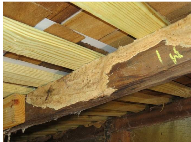
Photo 238. Significant fungal growth on the north secondary rafters in Rafter Bays R16 and R17.
