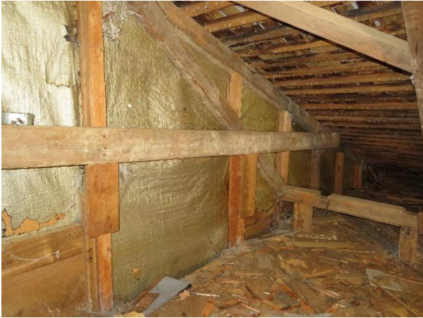
Photo 239. Mix of structural members used to frame the west gable end wall.
