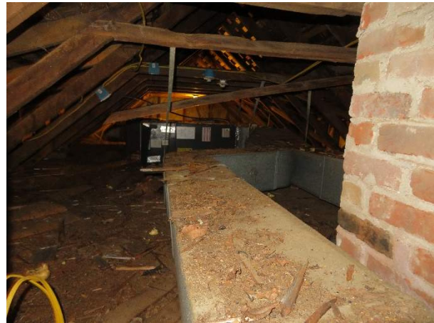
Photo 349. Abandoned HVAC unit in attic.
