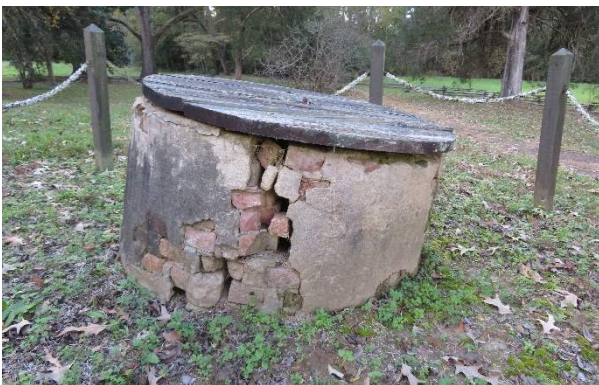
Photo 25. Cistern #1 to the northwest of the main house has failed.
