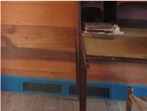
Photo 350. Abandoned registers in the base board of Room 2 (102).
