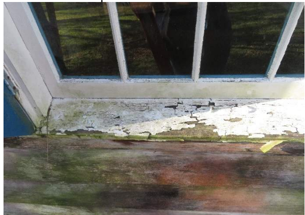
Photo 117. Deterioration of the sill.
