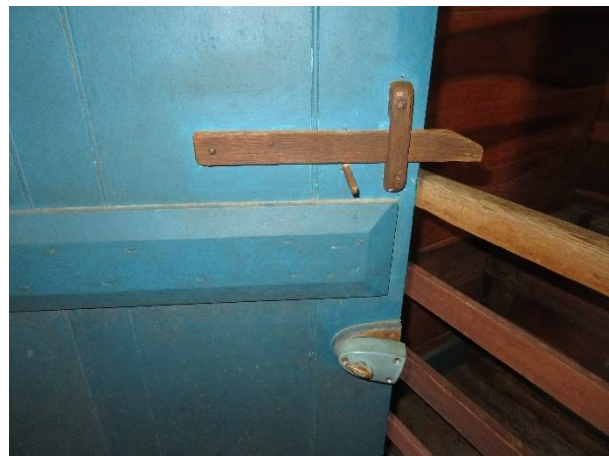
Photo 283. Interior hardware, showing the lift latch and the damaged rim lock.
