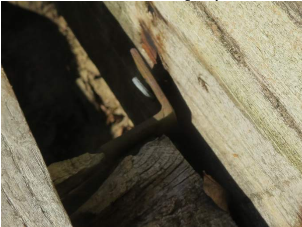
Photo 33. Distress to stair support at gallery rim joist.
