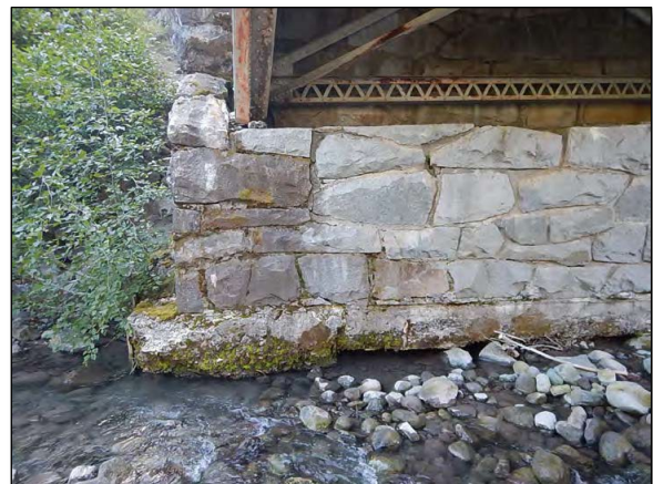
Undermining and spalling of the east bridge abutment (FHWA 2020)
