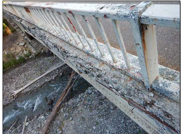
Severe spalling and exposed rebar on exterior face of curb, upstream side (FHWA 2020)
