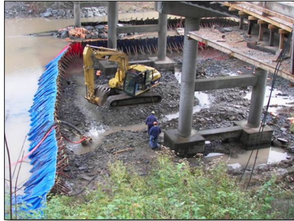
Push-up cofferdam installation in a creek with high background turbidity levels (FHWA photo)
