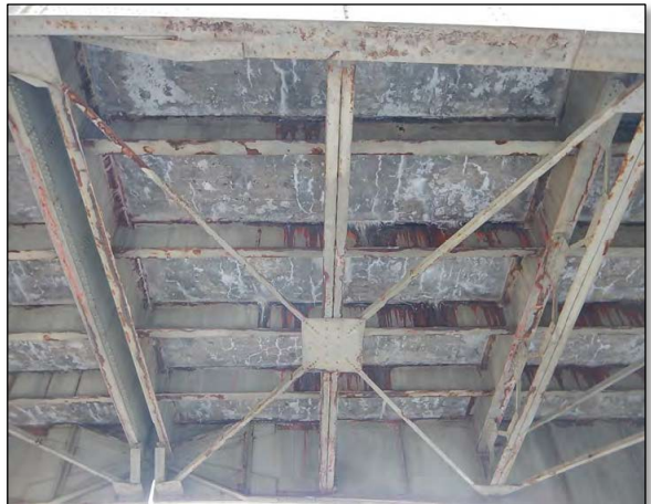
Rusting and corrosion of the floor and cross beams, underside of the bridge (FHWA 2020)
