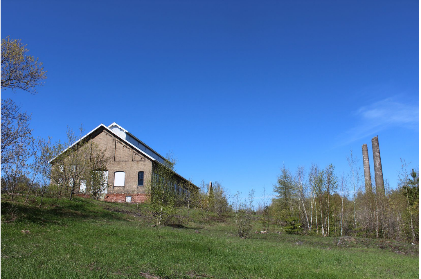
Quincy Mine Industrial Core Landscape Character Area 1. South end and east side of the Quincy Machine Shop (MAP ID# 023), the No. 2 Boiler House Stack (Map ID# 025) and the No. 6 Boiler House Stack (MAP ID#26) in the distance.
