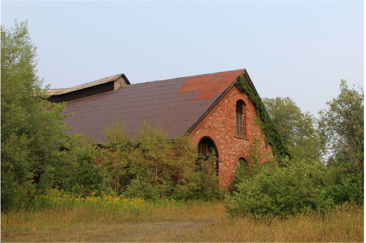
Calumet and Hecla Mine Industrial and Management Core Landscape Character Area A, the Hancock & Pewabic Boiler House (Map ID# 13).
