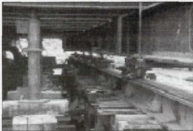
The lighthouse begins its journey after being lifted. The travel beams are supported by oak cribbing below and carry the Hillman Rollers, the main beams and the cross beams along with the lighthouse above.
