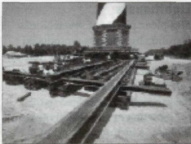
Travel beams are put in place to move the lighthouse over ground zero, the lighthouse's new home for the next 100 years.
