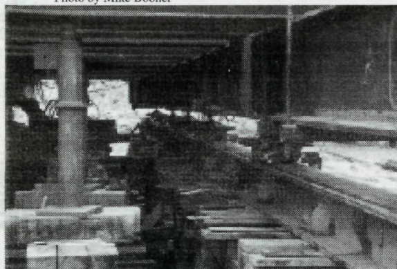
The lighthouse begins its journey after being lifted. The travel beams carry the Hillman Rollers, the main beams and cross beams along with the lighthouse above.
