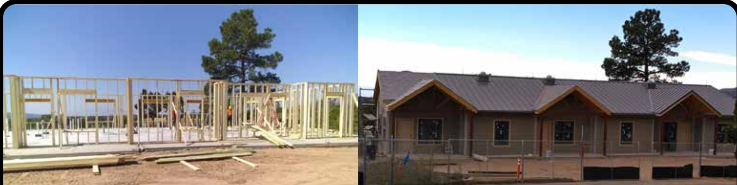
Above left, walls are erected in multiplex housing units being built at Bandelier National Monument in New Mexico. Above right are the completed units, which will house seasonal employees. Photo: Courtesy NPS
