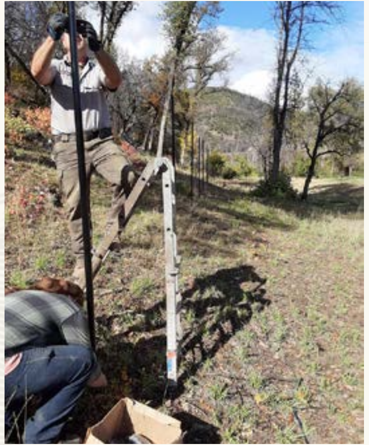
NPS staff install posts for a fence at the WHIS Back Field orchard (NPS).
