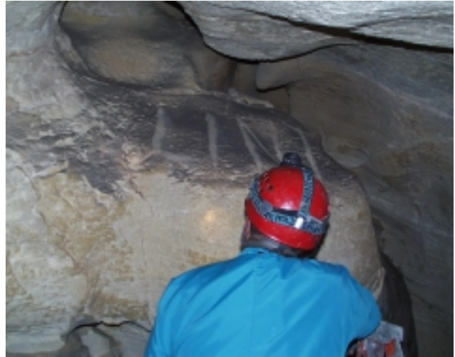
A thick layer of lint awaiting removal. (NPS Photo by Jon Jasper)
