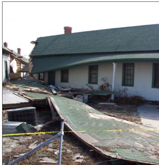
Building 5, which housed the main park exhibits, was torn from its foundations and the T-shaped structure broken apart.
